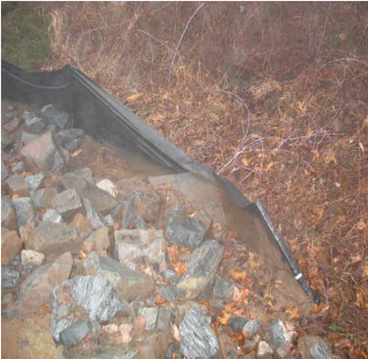
Riprap sediment trap and silt fence along the access road off Black Walnut Drive. Some run-off was pooling over the fence at the time of inspection. The accumulated sediment should be removed and the silt fence repaired, but this does not affect resource areas.
