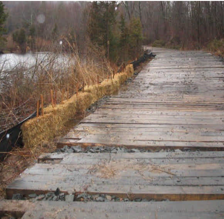
View of a low, saturated spot at the timber mats crossing in the wetlands located off Powder Hill Rd. Haybales were added for increased protection. Continue to monitor.
