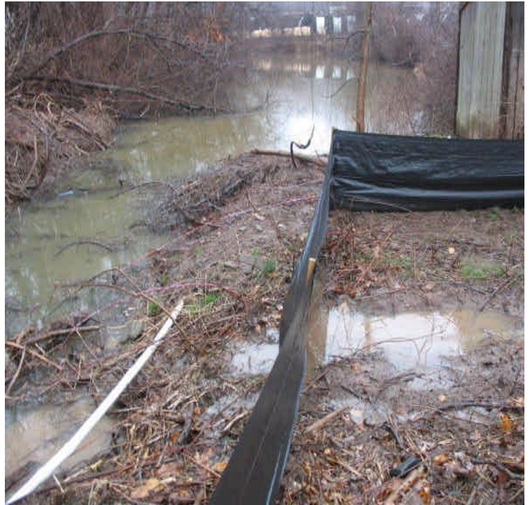
Turbidity was observed in the pond adjacent to the contractor receiving yard. During the rain event, turbid water was observed flowing under/through controls and into pre-existing drains.
