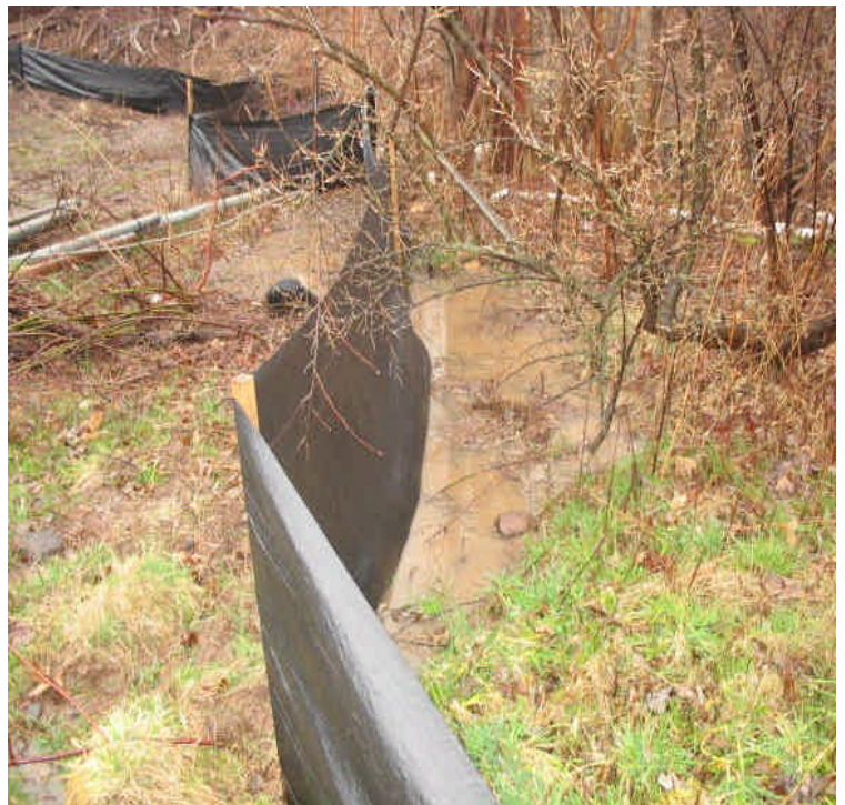
Turbid water was observed flowing under the silt fence above the pond at the contractor receiving yard.
