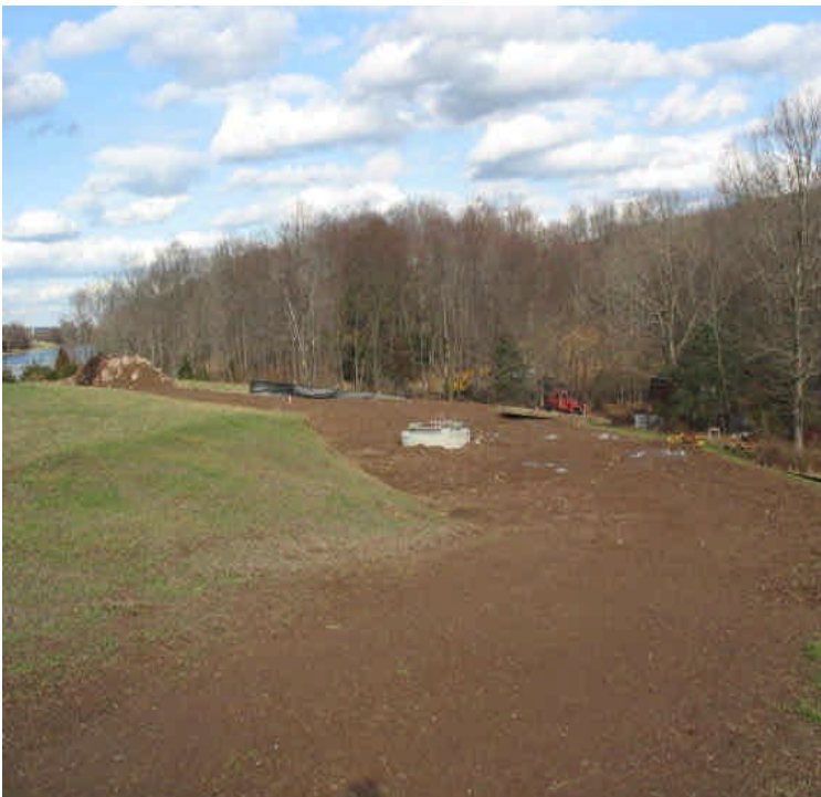
Foundations installed within the ROW north of Beseck SS. Controls are in place. Some grass cover noted.
