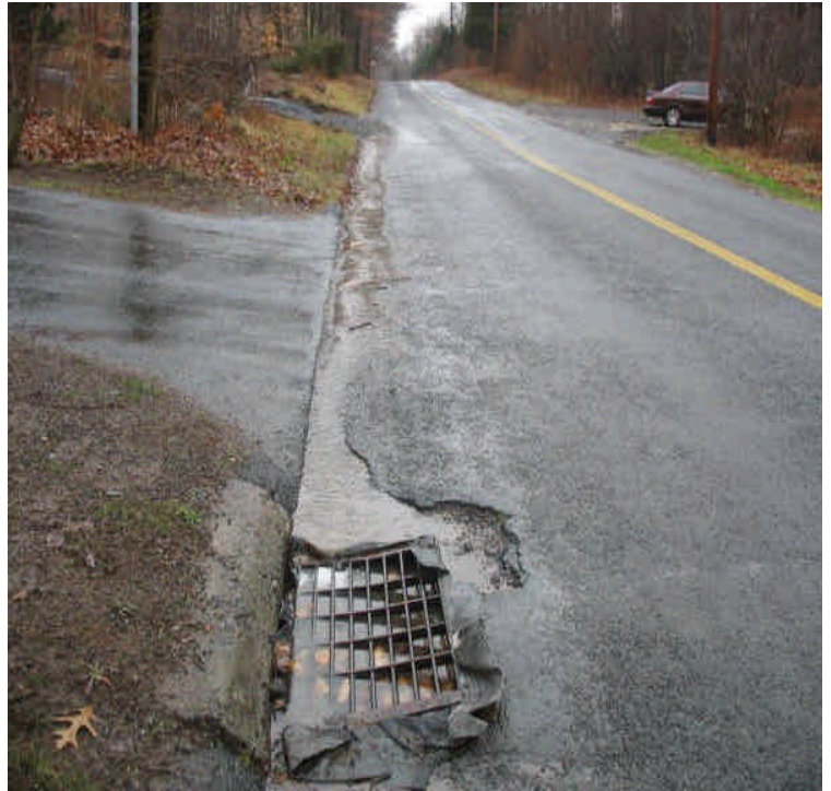
Slightly turbid run-off from the access road off Arbutus St was being filtered by controls in the CB. Pull back construction entrance stone from the roadway and maintain CB protection as needed.
