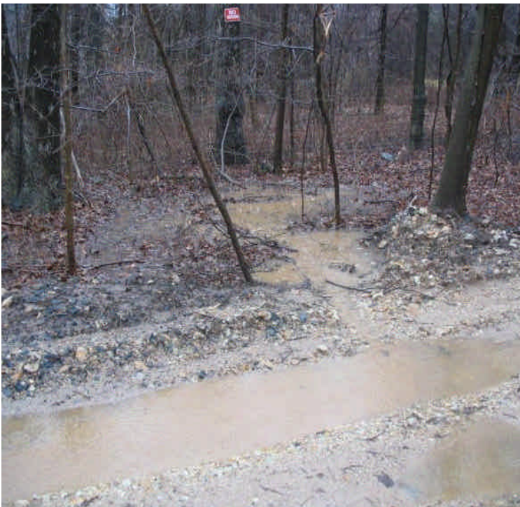
Access road off Haddam Quarter Rd. Turbid run-off from the access road was flowing off-site but was not reaching resource areas. Berm up the road or install strategically placed controls when feasible.
