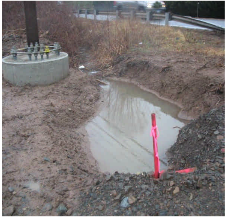
Some turbid run-off was noted in the swale adjacent to the foundation in the ROW north of the contractor yard along Rte 17. The stormwater flows to the slurry holding areas where it remains contained.
