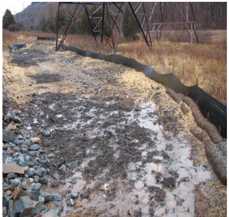
Silt fence/filter-sock barrier along the access road adjacent to Black Pond used for dewatering slurry and controlling run-off. Run-off was filtering through the fence and appeared free of sediment on the other side.
