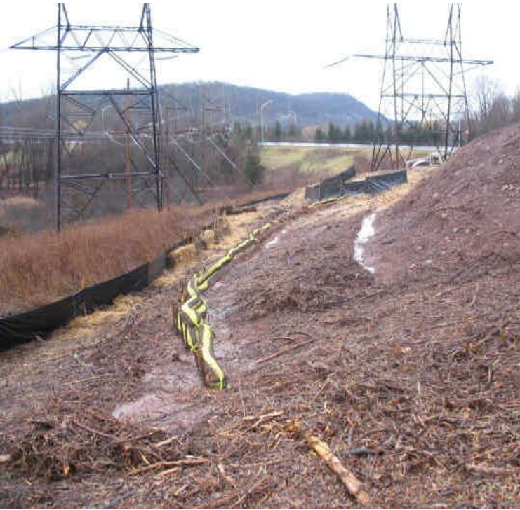
Overview of the haybales, silt fence, and filter socks at Black Pond. Mulch is in place around the site for increased stabilization.
