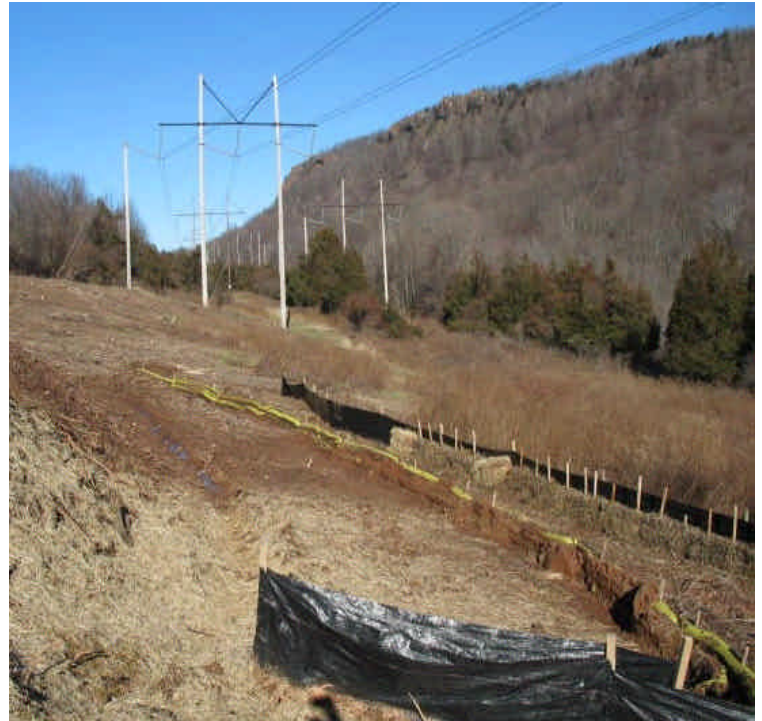
Silt fence/bio-sock barrier along the access road adjacent to Black Pond used for dewatering slurry. Slurry has been spread around the site.
