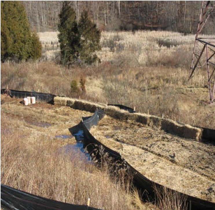
View of the new haybales and silt fence at Black Pond. Mulch is in place around the site for increased stabilization.
