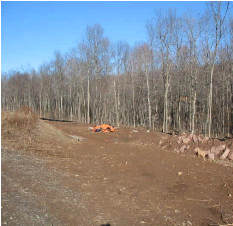
Foundations installed within the ROW north of Beseck SS. Controls are in place.
