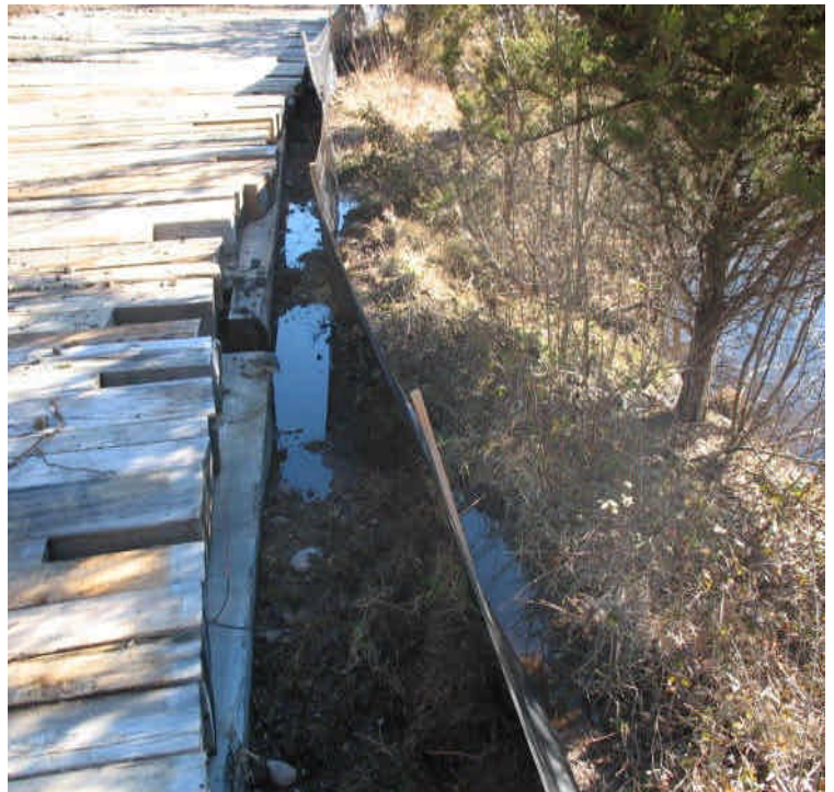
Silt fence and timber mats are in place along the access road off Powder Hill Rd. Access road follows an existing road through a wetland; silt fence protects a pond adjacent to the access road.
