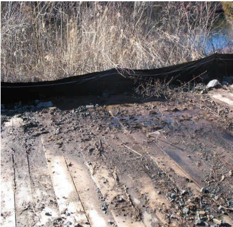
Sediment buildup along the timber mats crossing at a saturated spot in the wetlands located off Powder Hill Rd. Monitor controls and stabilize mats as necessary.
