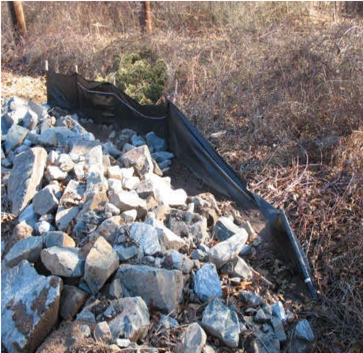
Riprap sediment trap and silt fence along the access road off Black Walnut Drive. Accumulated sediment should be removed and the silt fence repaired.
