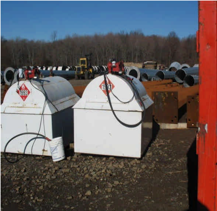
Fuel tanks and dumpster moved, controls for nozzles were partially reinstalled.
