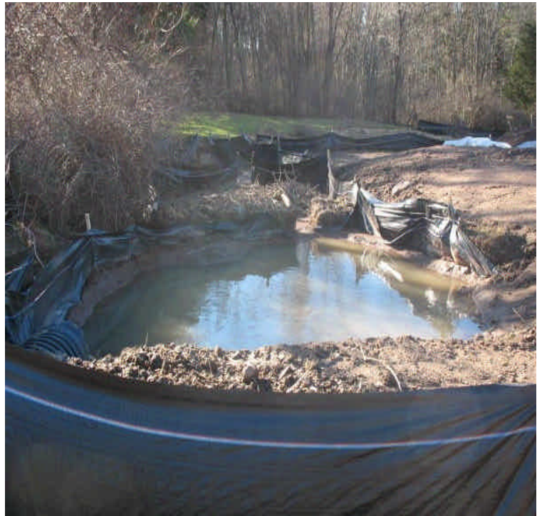
Slurry containment areas located in the ROW north of the contractor yard along Rte 17. Stormwater remains contained in the basin.
