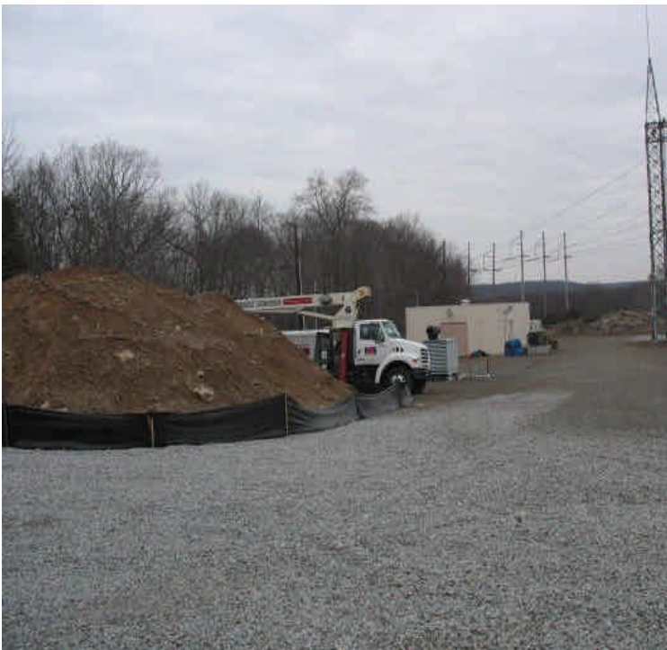
The remaining soil stockpile is surrounded by silt fence. Fallen section of silt fence has been repaired. All soils remain well contained to the site.
