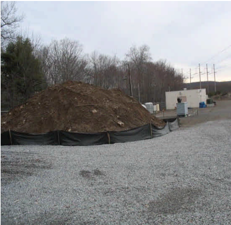
The remaining soil stockpile is surrounded by silt fence. Fallen section of silt fence has been repaired; remove soil from site when feasible. All soils remain well contained to the site.
