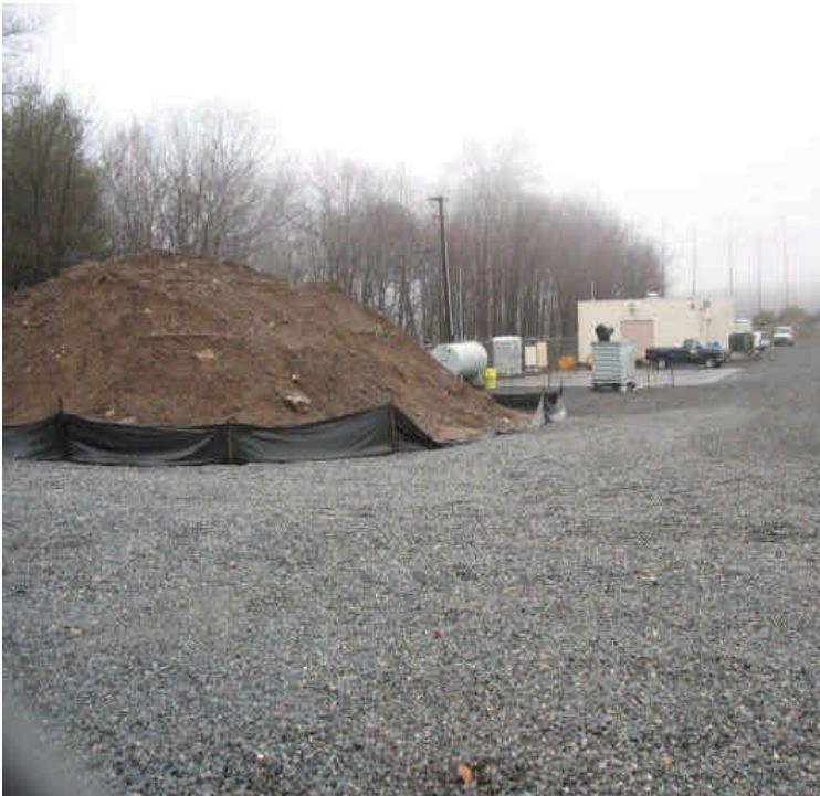
The remaining soil stockpile is surrounded by silt fence. Repair fallen section of silt fence and remove soil from site when feasible. All soil remains well contained to the site.
