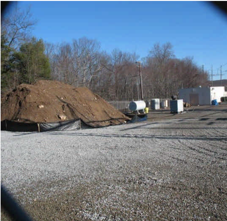
The remaining soil stockpile is surrounded by silt fence. Repair fallen section of silt fence and remove soil from site when feasible.
