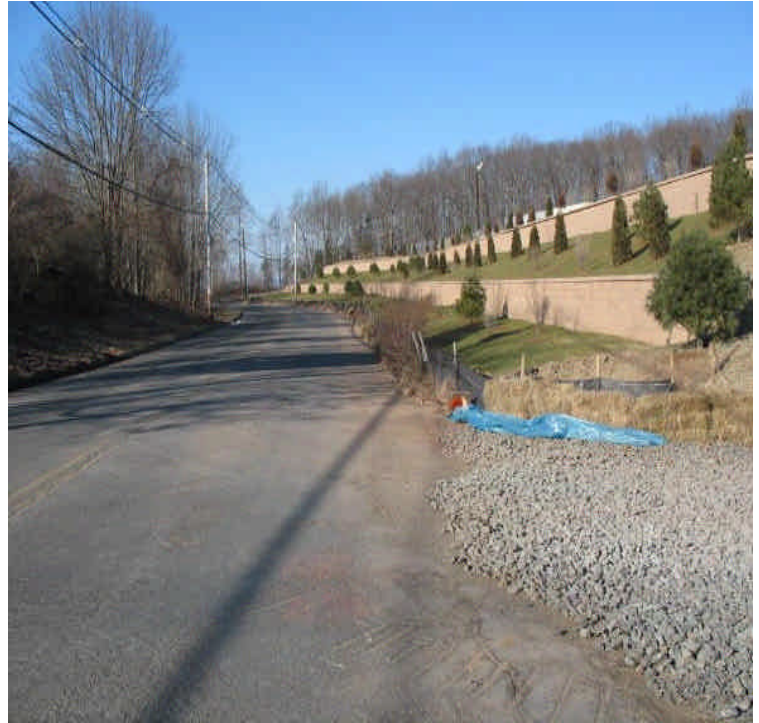
View of Carpenter Lane and retaining walls. Since the improvements were made at the stone pas and along the roadway, sediment tracking And turbid run-off were not issues at this time.
