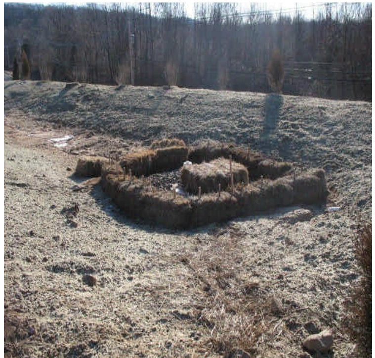
Surface areas on site are fully hydroseeded (including a tackifier) in an effort to stabilize soils. Additional haybales were installed at the inlet. Hay mulch covers the eroded gullies on the basin slope. No run-off was observed this week.
