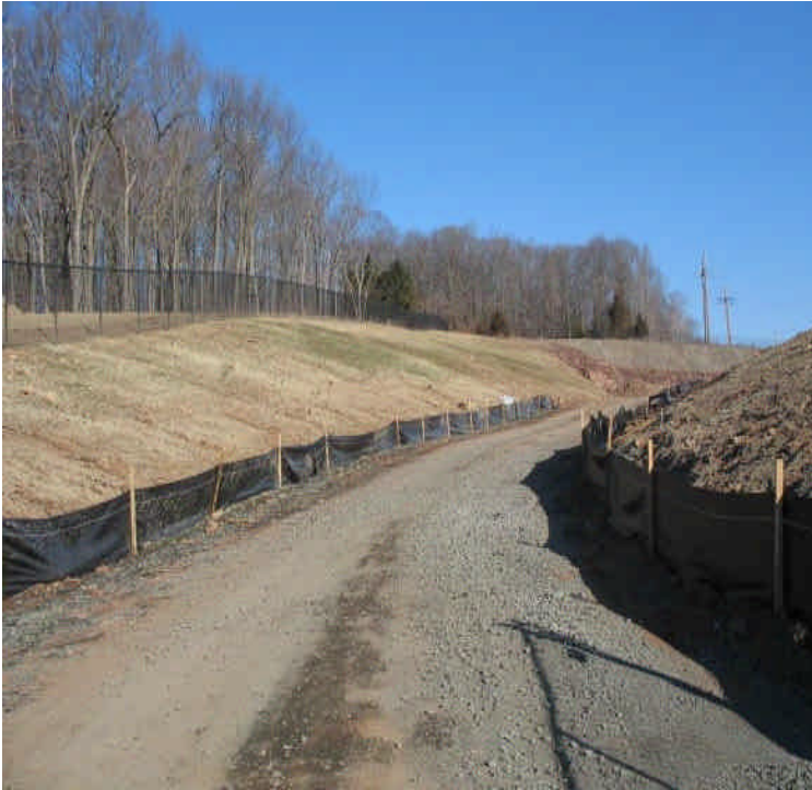
Site entrance off Carpenter Lane is at final grade; erosion controls have been restored following conduit installation. Monitor carefully for run-off.
