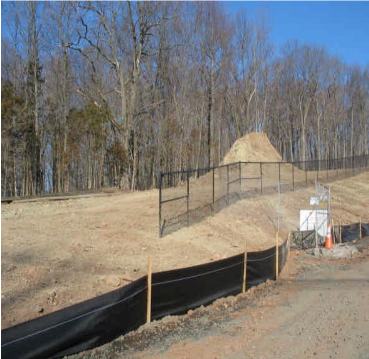
Haybales were in place across the old Zolnik driveway. The remaining stockpile and exposed surfaces are hydroseeded (including a tackifier).
