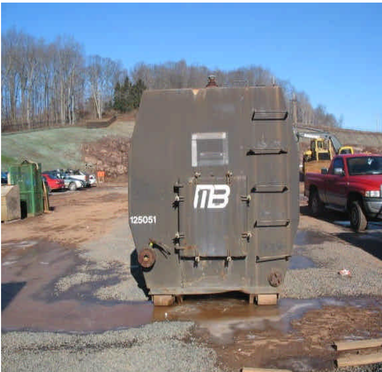
Dewatering from foundation pits is being pumped into frac tanks to settle and eventually released to the site. Clean water could be pumped directly to the protected CB at a low flow rate so as not to overwhelm controls.
