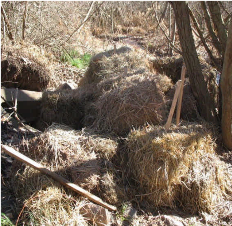
Sediment has settled out at the storm drain outlet across Carpenter Lane. Clear water was noted flowing through the recently replaced haybales. The additional efforts on site appear to be effective at reducing sediment. Continue to monitor.
