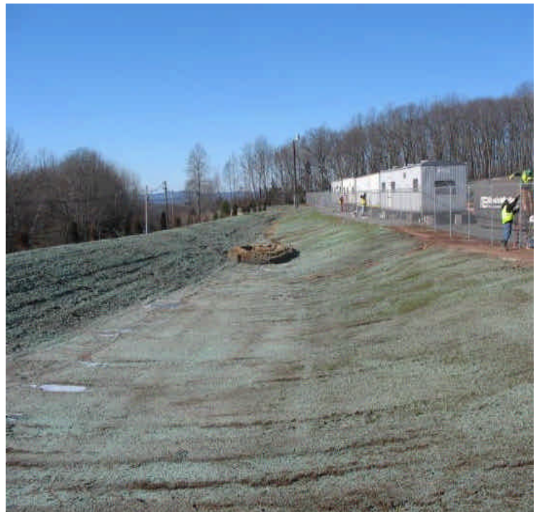
Surface areas on site have been fully hydroseeded (including a tackifier in an effort to stabilize soils. Additional haybales were installed at the inlet. Hay mulch was also added to the eroded gullies on the basin slope.
