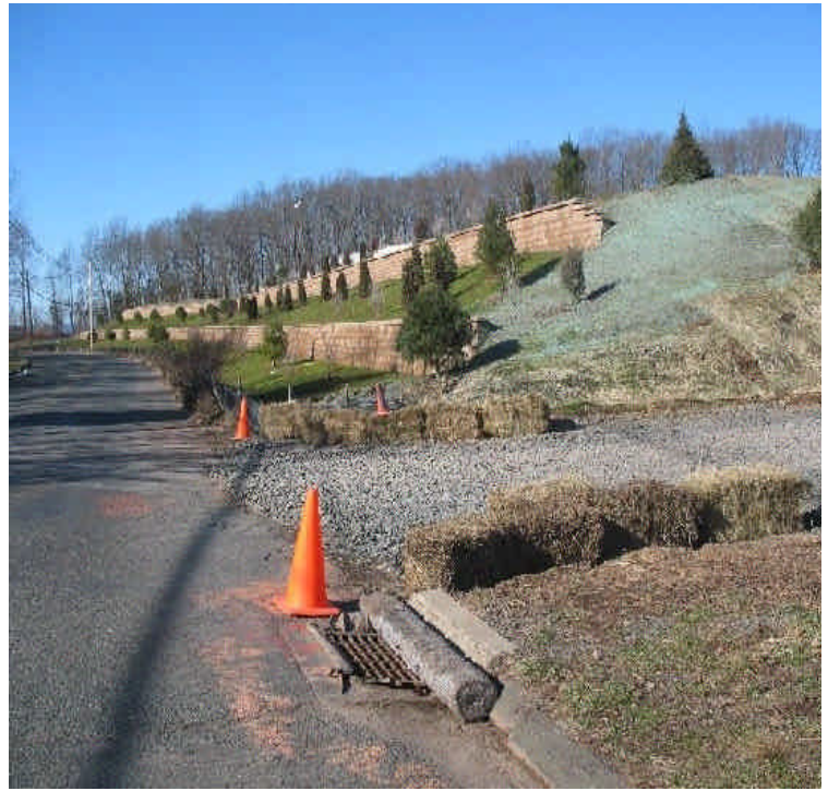
View of Carpenter Lane and retaining walls. Sediment accumulation was removed from the gutters, new haybales were installed, CB controls were cleaned and the stone entrance was improved.
