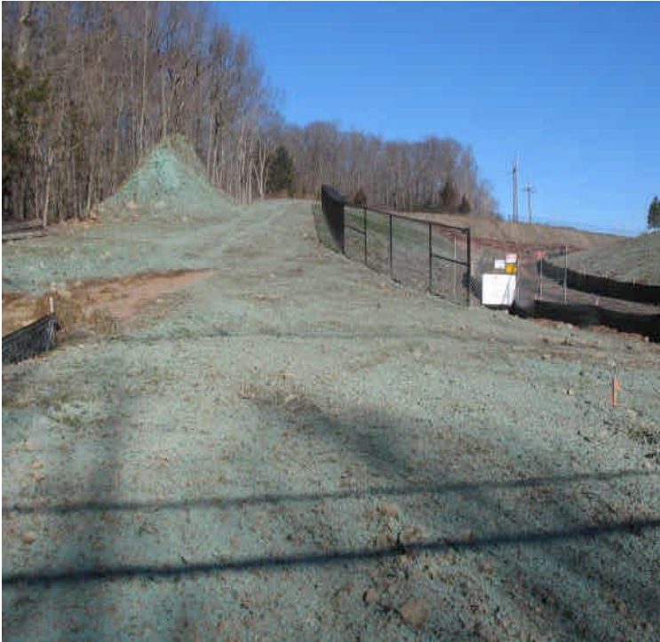
Haybales were replaced across the old Zolnik driveway. The remaining stockpile and exposed surfaces have been hydroseeded (including a tackifier).
