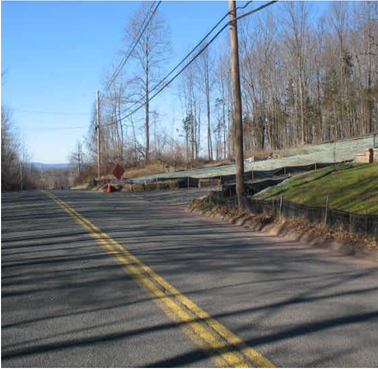
Site entrance off Carpenter Lane is at final grade; erosion controls have been removed. Monitor carefully for run-off.
