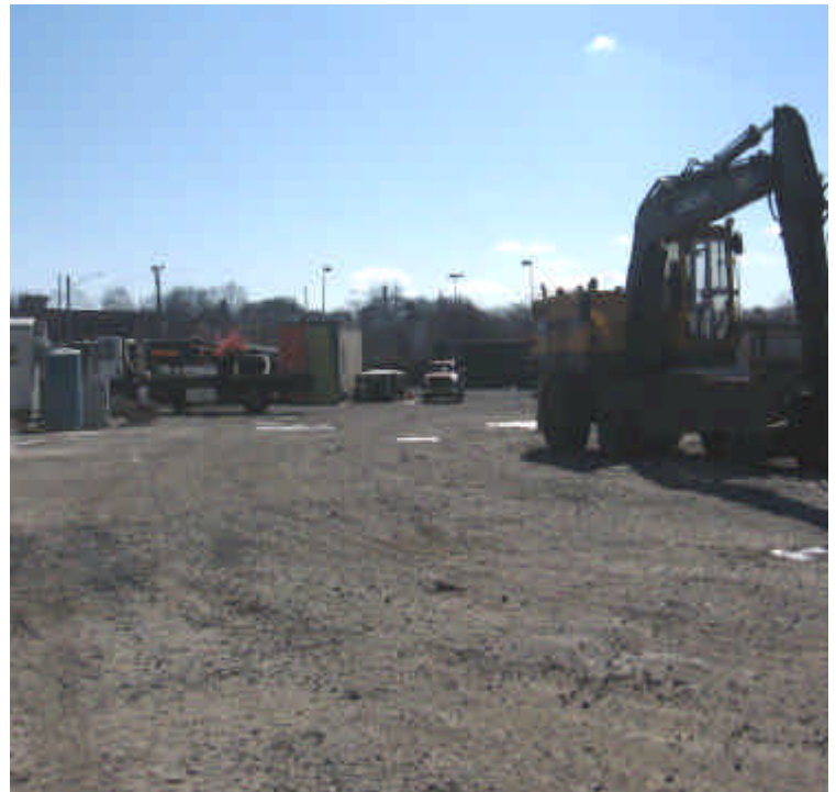
Airborne dust was noted in the Kings Highway lay down Yard at the time of our inspection. Attempt to water down soils or provide other dust control.
