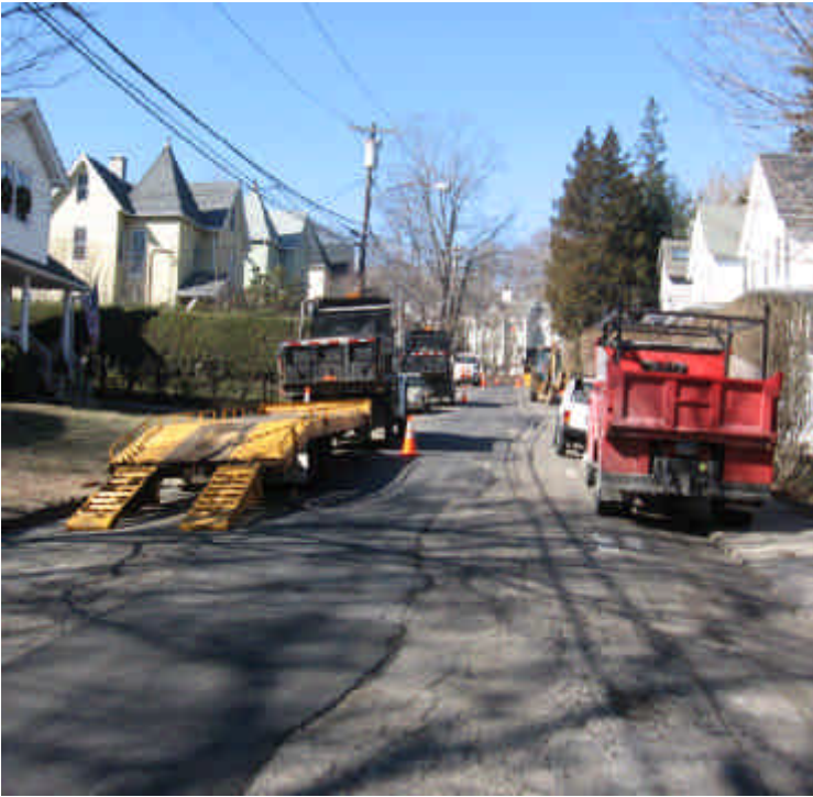
Photo of completed trenching activities on Lincoln St. Some related utility work continues here (performed by others).
