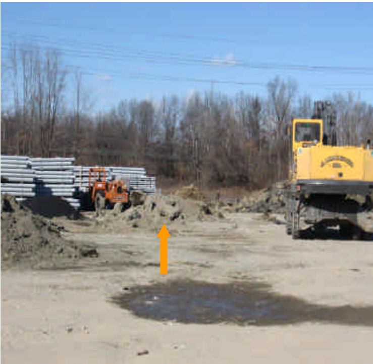
The small stockpiles indicated are the remnants of the concrete washout area within the Kings Highway lay-down yard.
