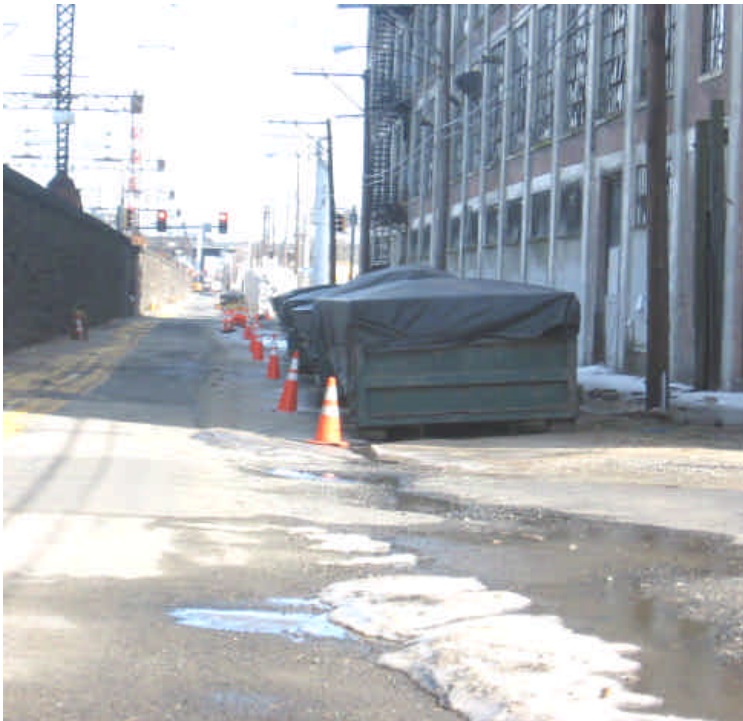
Photo of covered dumpsters storing soil along the shoulder of Railroad Ave. near its intersection with Howard Ave. It is anticipated that these dumpsters will be removed within the week.
