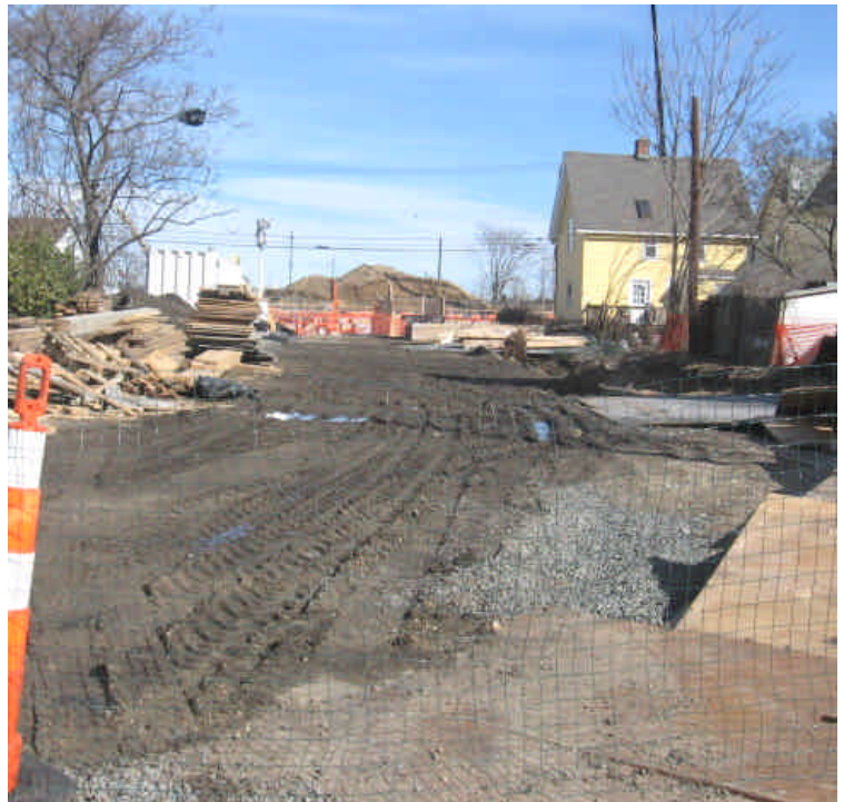
Photo of trenching activities between Broad St. and Main St. No issues were noted.
