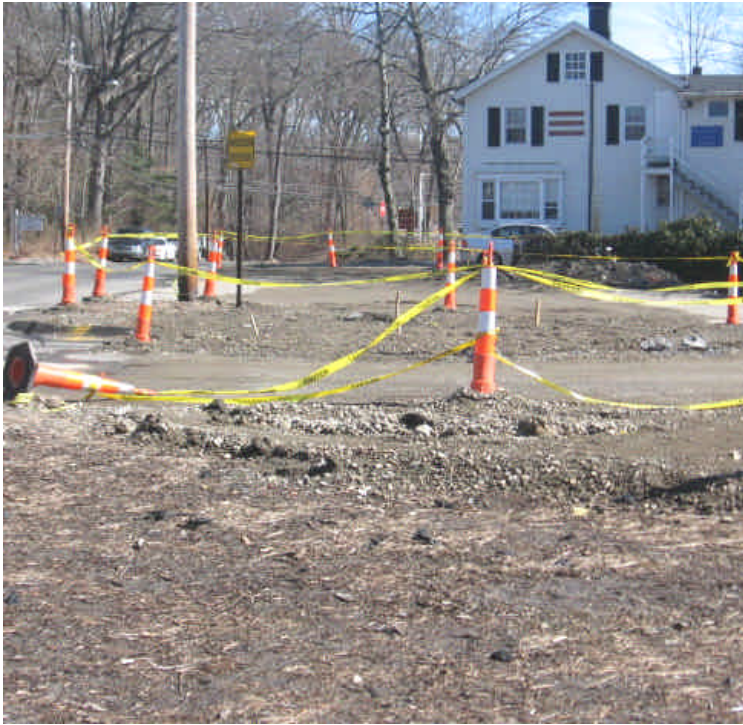
Trenching activities near Vault #28 are complete. Exposed soils are comprised of hard pack that resists erosion. Final stabilization will still be necessary.
