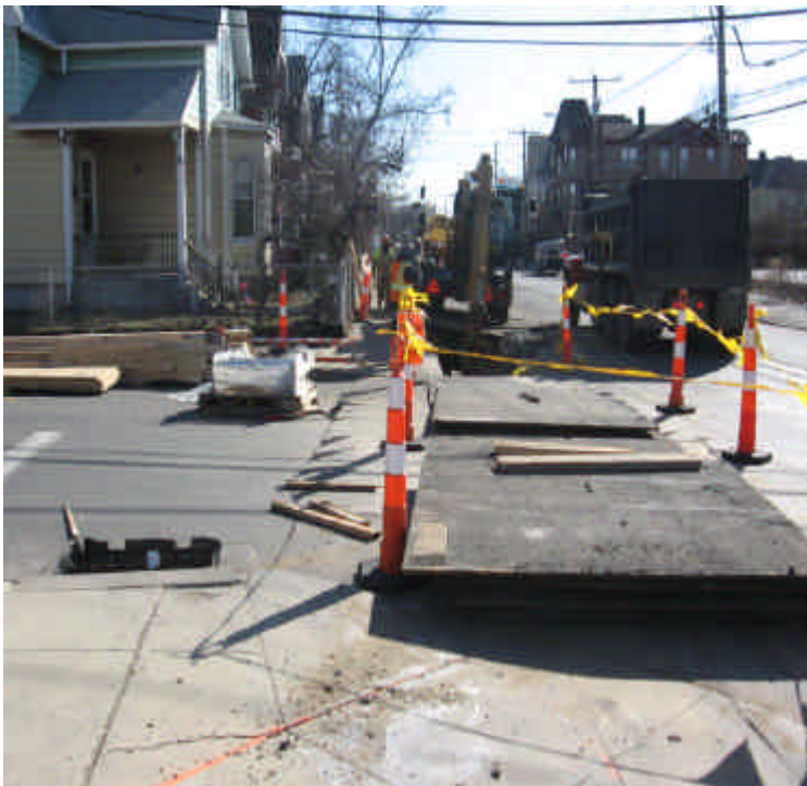
Trenching activities along Broad St., all catch basins have appropriate controls in place.
