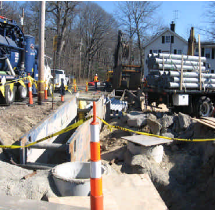
Trenching activities adjacent to Vault #28. Catch basins located downgradient of trenching activities remain unprotected.
