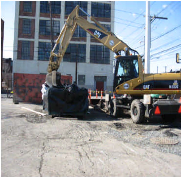
Trenching activities at the intersection of Howard Ave. and Railroad Ave. Soils being removed were high in lead content and appeared to be handled appropriately.
