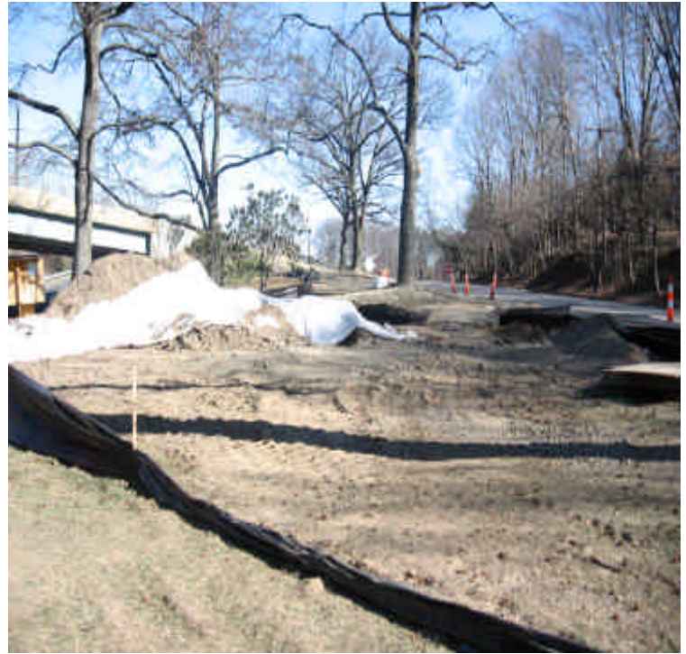
Construction area along Pequot Ave. Soil pile remains stable. It is recommended that compromised erosion controls be re-established.
