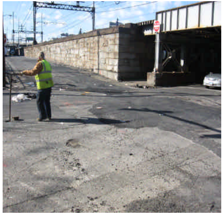
Photo of a completed section of trench on Railroad Ave. near near its intersection with Myrtle Ave.
