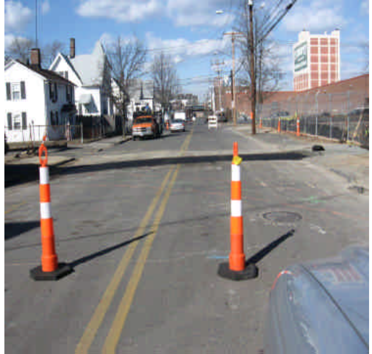
Trenching activities across Main St. to the Singer substation yard appear to have been completed.
