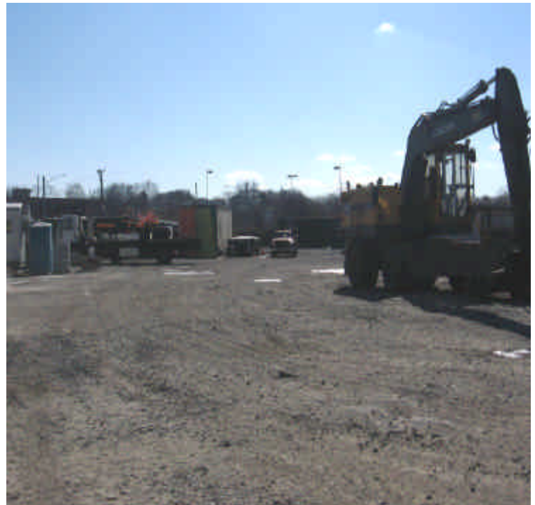
Airborne dust was noted in the Kings Highway lay down yard at the time of our inspection. Attempt to water down soils or provide other dust control.
