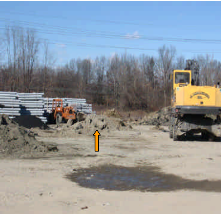
The small stockpiles indicated are the remnants of the concrete washout area within the Kings Highway lay-down yard.
