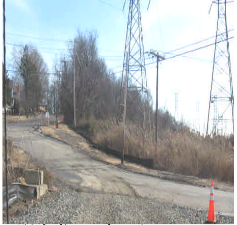
Minimal tracking was noted near station #1052 onto Naugatuck Ave. Sweep the roadway when necessary.
