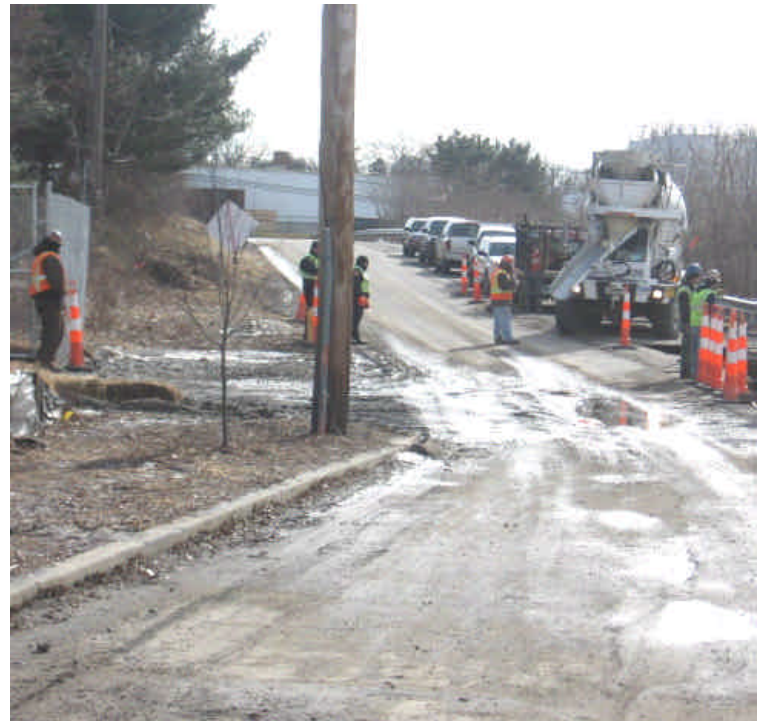
Photo of trenching activities on Shelland St. near the entrance to the Milford lay-down yard. Minimal sediment tracking was noted and the stone entrance pad had been refreshed since last week's inspection.
