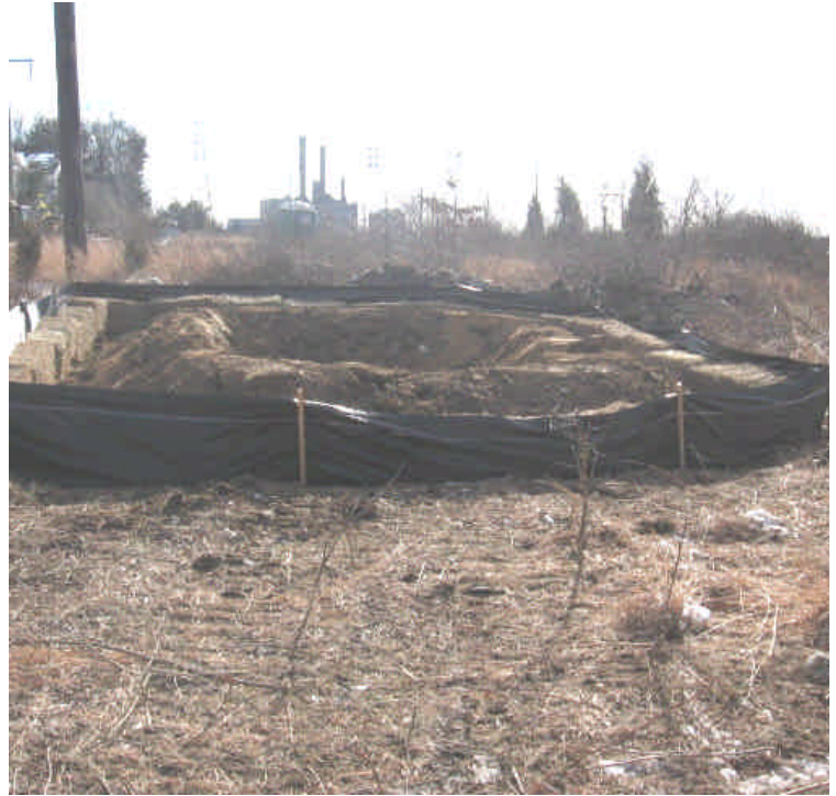
In preparation for construction activities, and potential dewatering or washout, a contained basin has been installed near station #1073.
