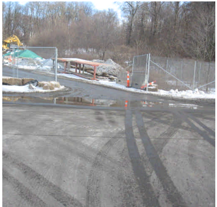
Minor sediment tracking noted from the Milford contractor lay-down yard. Continue to monitor and mitigate if necessary.
