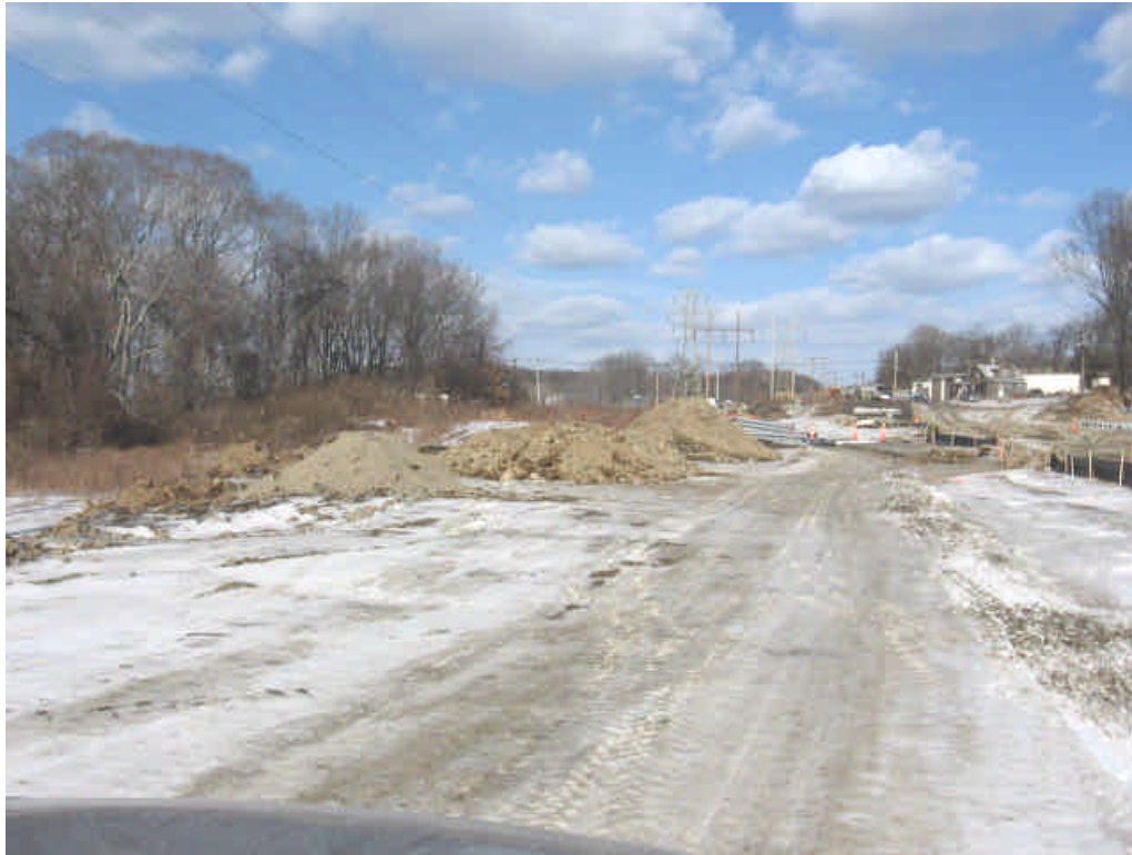
Photo taken near station #1111. Trenching activities shown to the right of the photo while wetland resource area is located to the far left. Stockpiles have potential to migrate towards wetland and into its buffer zone but do not appear to be here as a result of the project (noted for the record). NU contractors should continue to remain aware of the adjacent resource area.
