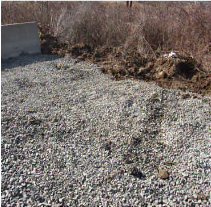
Remnants of the concrete washout near station 1055 have been removed and properly disposed of.
