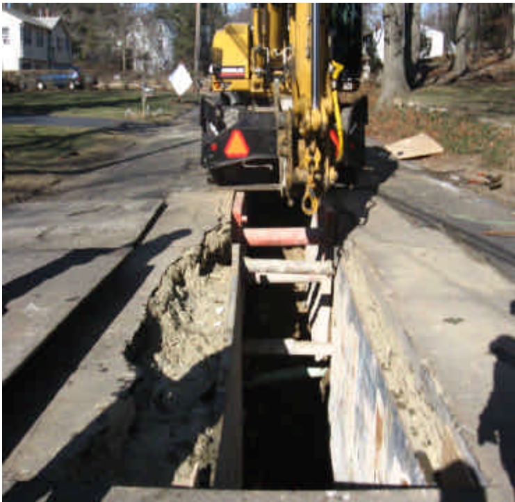
Photograph of trenching activities from station 1035 to 1037,. Dewatering activities were being conducted.
