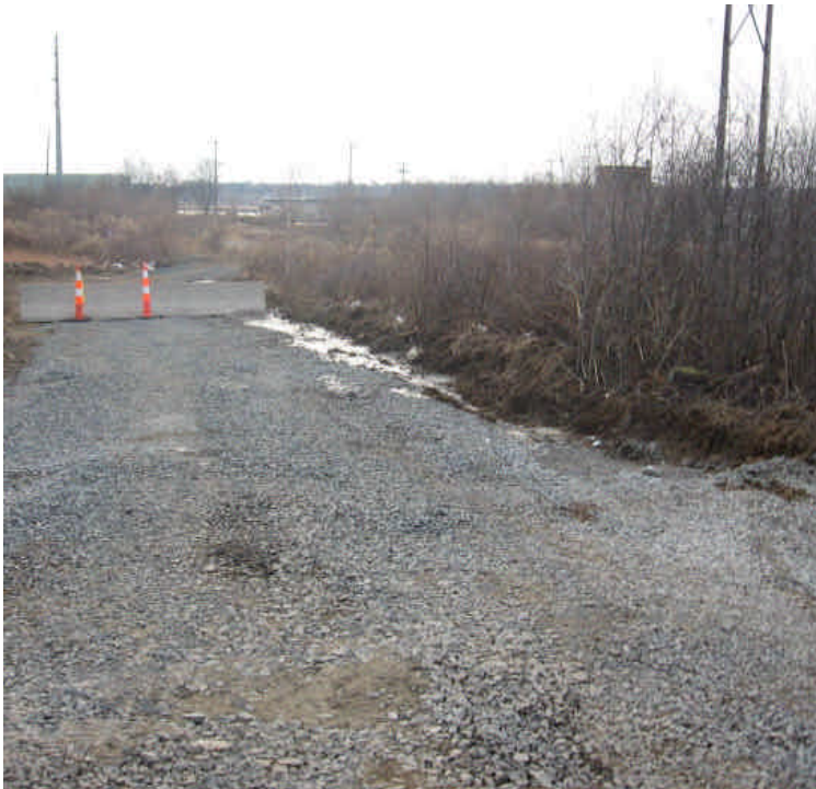
The uncontained concrete washout remains along the access road near station #1055. The concrete should be removed and properly disposed of.
