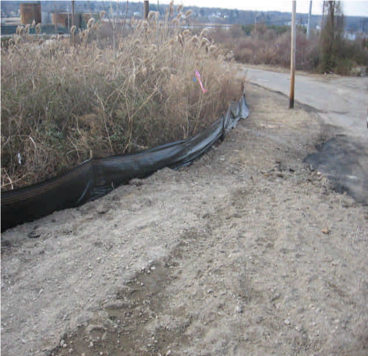
A portion of silt fence near station #1051 still needs to be toed-in. While soils are somewhat frozen and stable at this time, a wetland area is adjacent.
