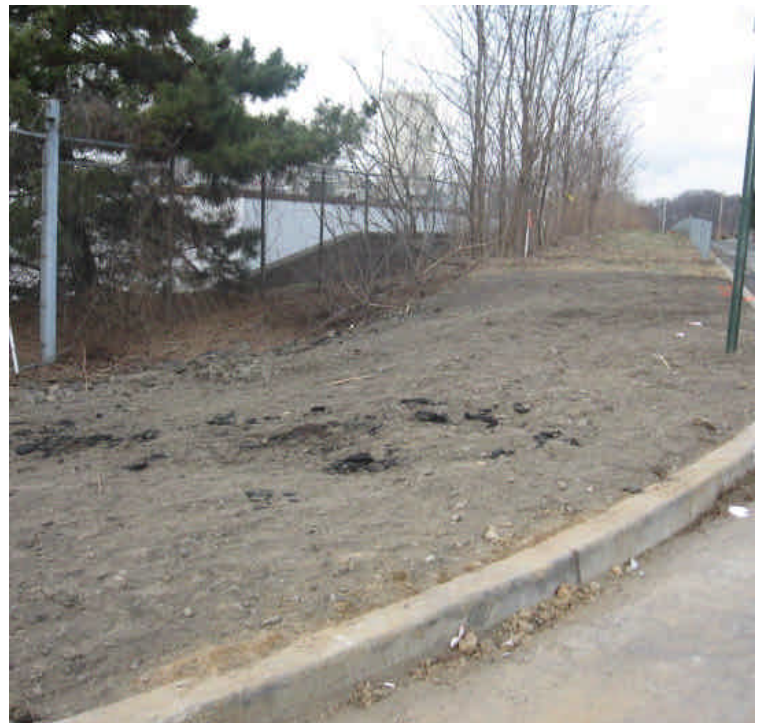
Exposed soils on the corner of Shelland and Caswell Sts. Although freezing temperatures are likely helping to stabilize soils, spread mulch or similar when feasible.
