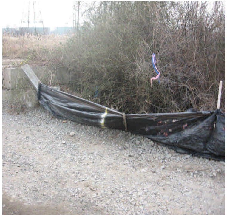
Ensure that the silt fence near station #1052 is toed-in and maintained as necessary.
