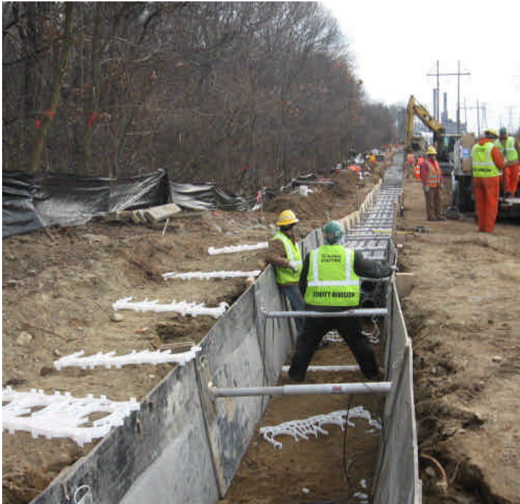
Trenching activities near station #1072. Vegetation has been cleared to accommodate the installation of the utilities.
