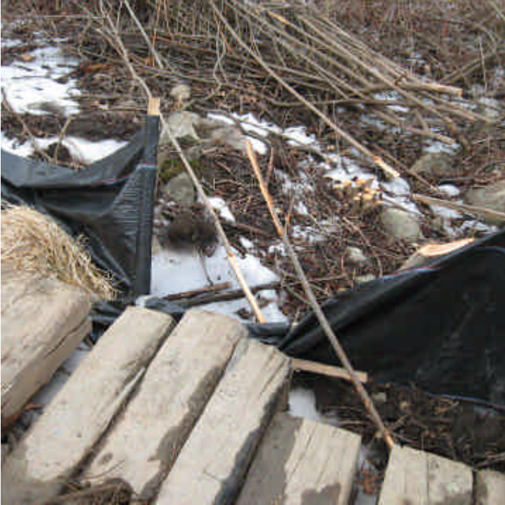
Portions of the silt fence should be repaired around the perimeter of the crane pad off Racebrook Road.
