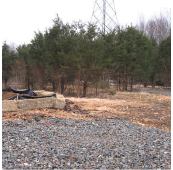
Dewatering controls were installed proactively near the proposed foundation locations off Salem Road.
