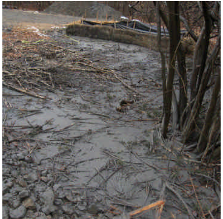
The dewatering controls were breached off Pine Tree Dr (east) and a significant amount of sediment was released into an upland area within the ROW. Improve containment to avoid adjacent run-off issues.
