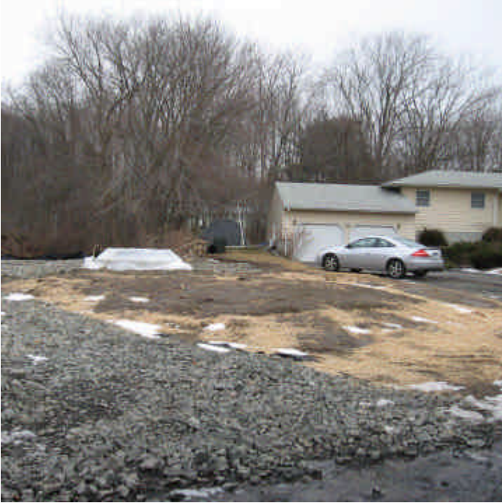
Some of the hay mulch was washed downslope leaving areas of exposed soil in the ROW off Edward Court. The catch basins remain protected here.
