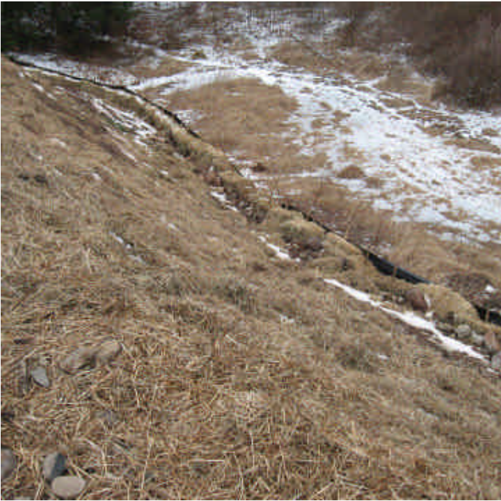
Hay mulch was applied to the disturbed slopes at the crane pad off Lambert Rd. proactively. Erosion controls remain intact here.
