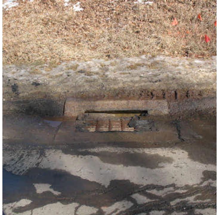
Some of the catch basins here do not appear to be adequately protected with gutter buddies or similar drop inlet protection. These were likely removed for town plowing purposes but need to be replaced.
