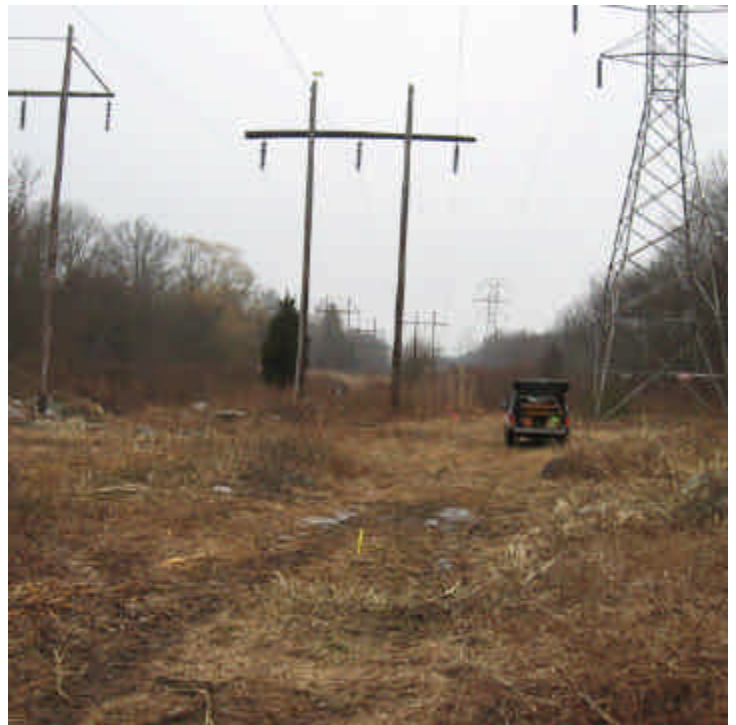
View of the recent clearing within the ROW off Manville Road in Woodbridge.
