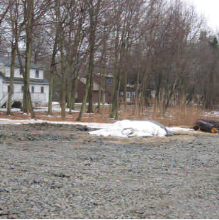
View of the newly poured foundation within the ROW off Pine Tree Drive (west).
