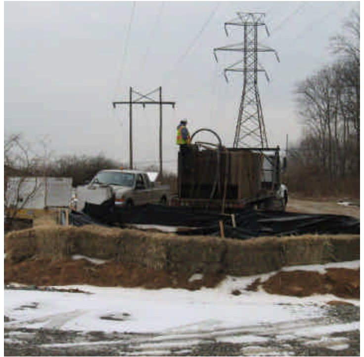
View of the dewatering basin constructed within the ROW off Dogwood Rd (east). Water is being trucked here from work areas to the west of Dogwood Rd.
