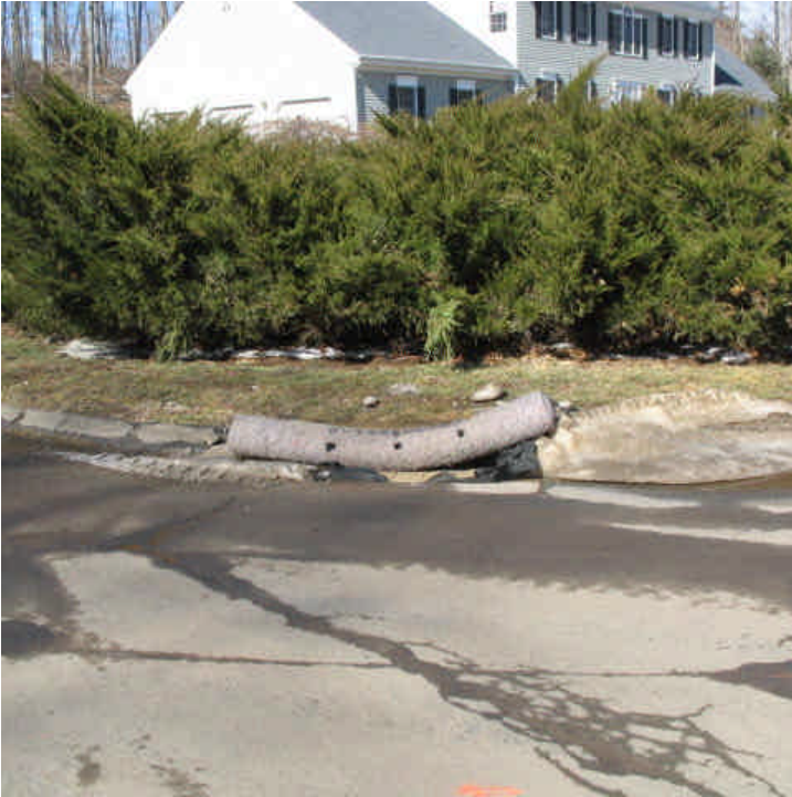
Gutter buddies were installed to protect the drop inlets in the catch basins near the 115 kV underground work in Hamden.
