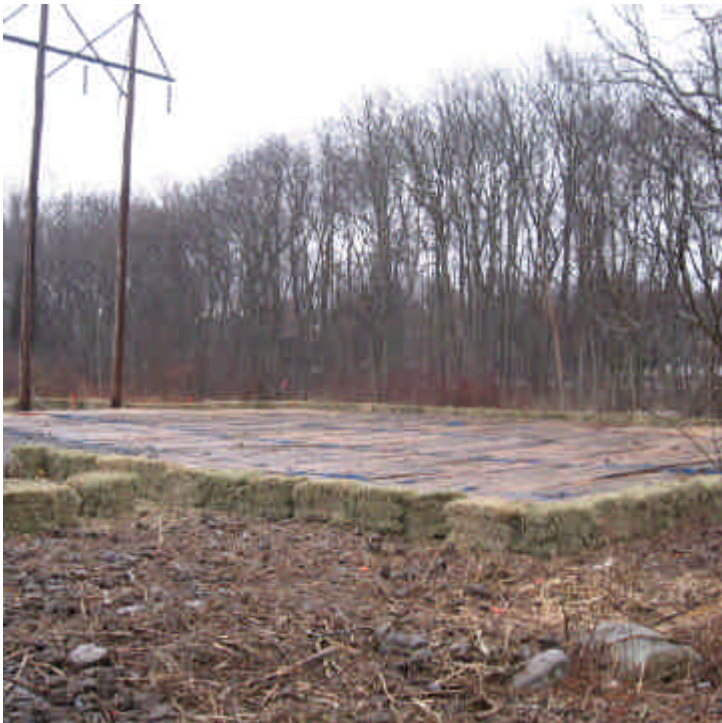
View of the timber mat crane pad and haybale barrier installed in the wetland off Salem Road.
