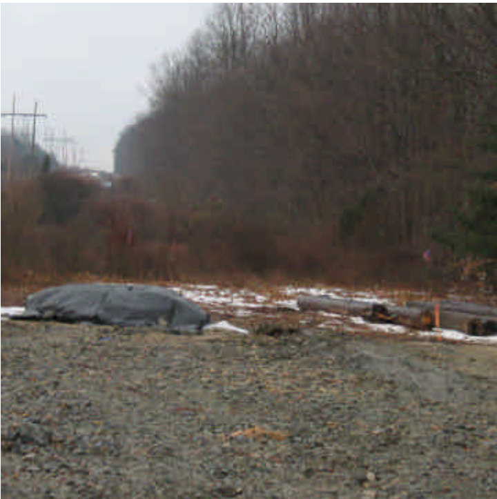
View of the newly poured foundation within the ROW off Pine Tree Drive (east).
