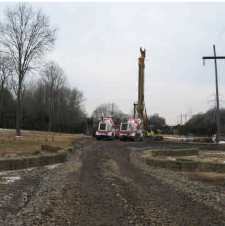
View of the foundation drilling/pouring within the wetland area off Dogwood Rd. (west). Haybales were in place at the stream.
