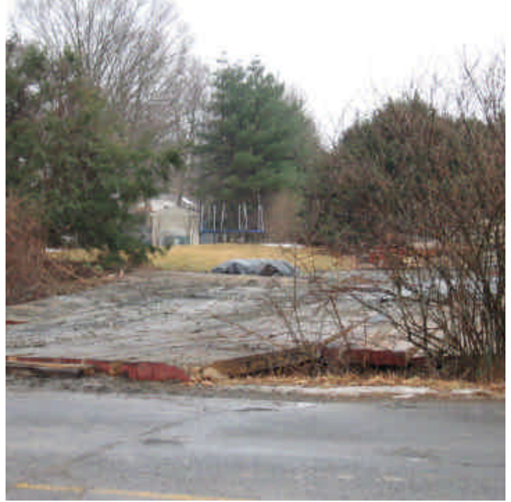
The small wetland area at the entrance of Pine Tree Dr (west) was matted for access to foundation construction.
