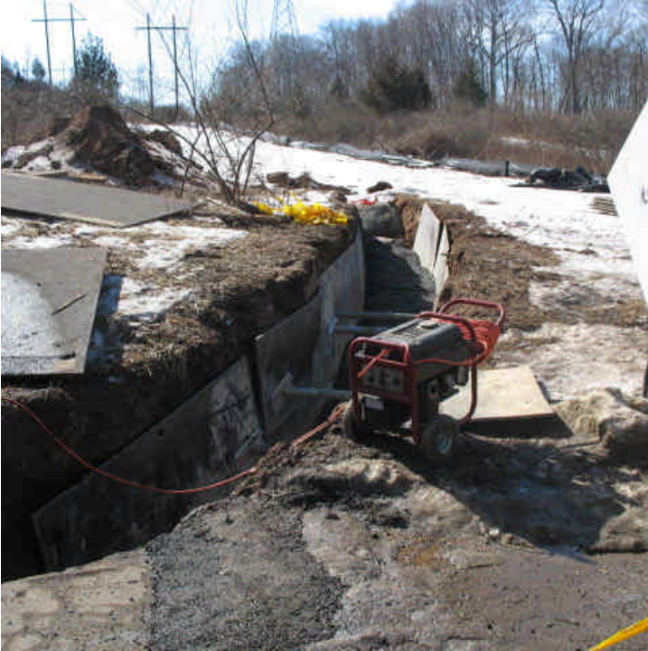
View of the trench work extending from the existing overhead ROW into Old Lane Road.
