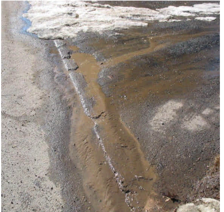
With the thaw, turbid run-off was again flowing from the low saturated area, filled by the access road installation. Run-off was reaching Old Farms Rd and entering a CB that did not have a gutter buddy in place.
