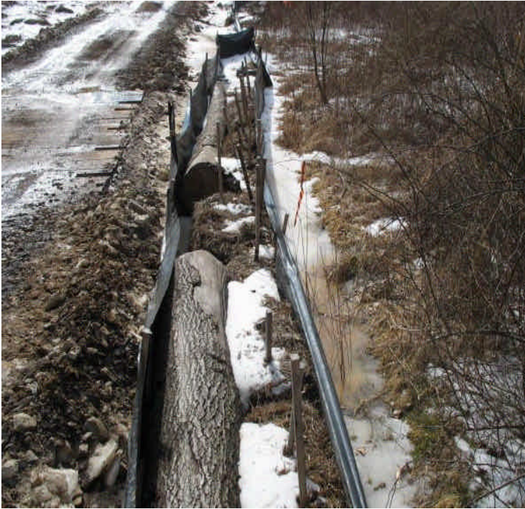
Some turbid run-off was observed flowing under or through controls in the ROW off High Hill Road.
