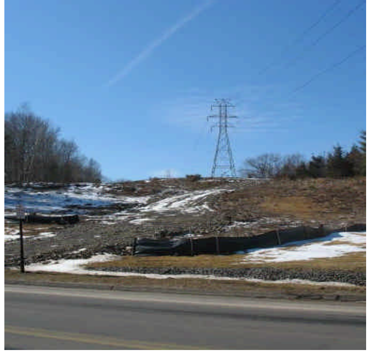
Silt fence remains intact along South Turnpike. Continue to monitor the slope for erosion, issues with run-off were not observed at this time.
