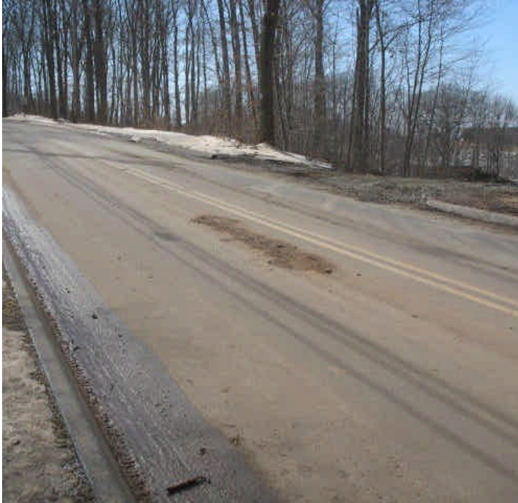
Some sediment tracking and accumulation was noted along High Hill Rd. Sweep roadway and remove sediment.
