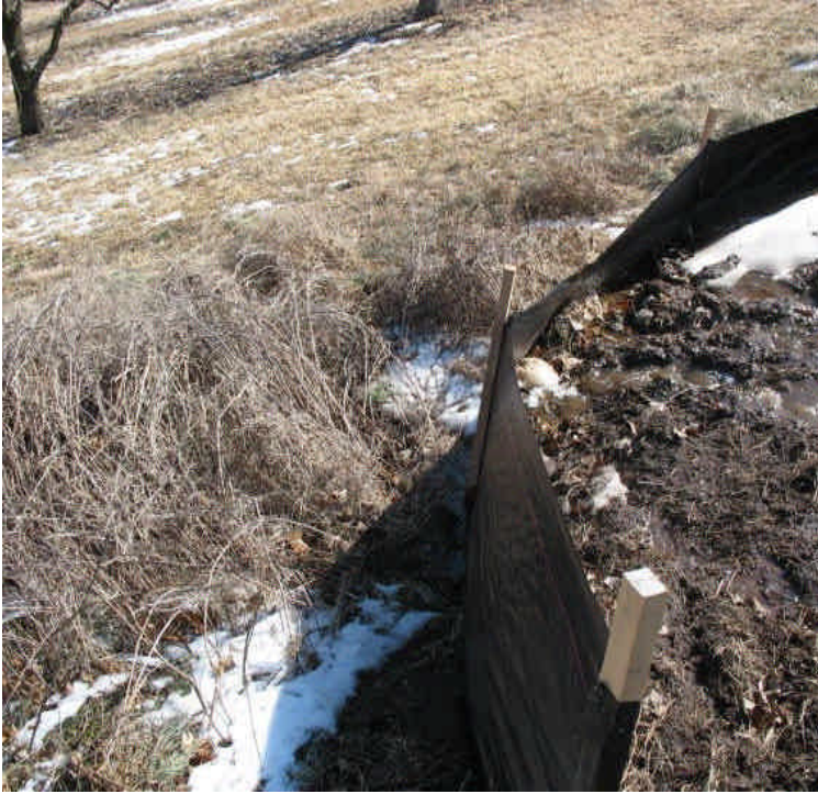
Small sections of silt fence were appropriately placed along the access road at points of run-off. This section within the apple orchard off Mansion Rd. was observed filtering run-off effectively.
