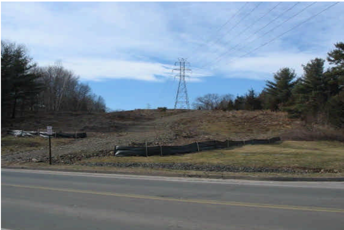
Silt fence remains intact along South Turnpike. Continue to monitor the slope for erosion, issues with run-off were not observed at this time.
