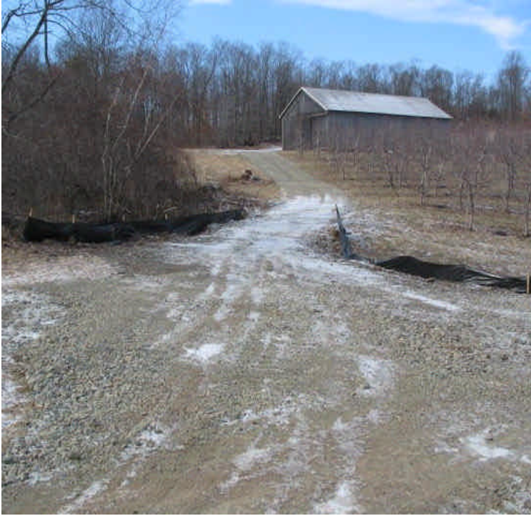
Silt fence remains intact along the access road adjacent to wetlands within the apple orchard off Mansion Rd.
