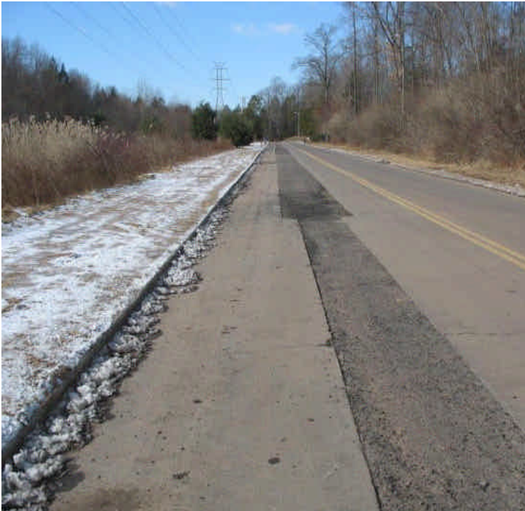
View of completed trench for the underground 115kv work on Old Farms Rd. Sweep up remaining asphalt/pebbles where work is complete. Cold weather appears to exacerbate the asphalt patch "crumbling".
