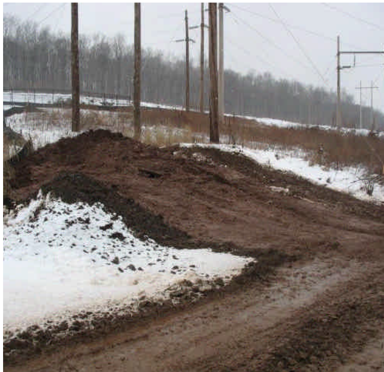
Slurry from foundation drilling in the wetland was being trucked and placed on a slope upgradient. Stabilize soils or install controls as necessary to prevent sedimentation from migrating
