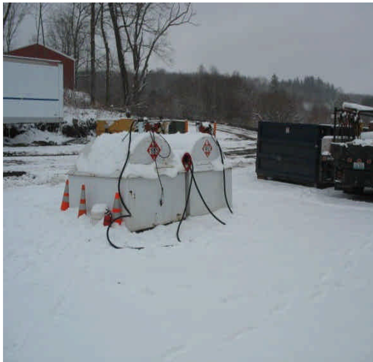
The fuel storage tanks remain in place on the stone spill pad and nozzles are contained. Small drip stains are noted and are contained to the stone.
