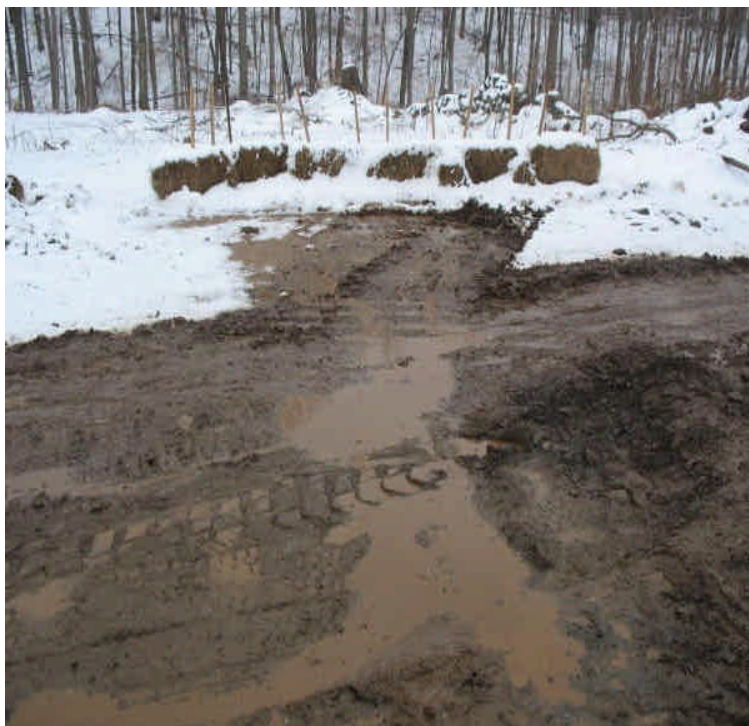
Water bars were installed along the access road north of Beseck SS. Turbid water is diverted off the road and towards haybales installed to filter sediment.
