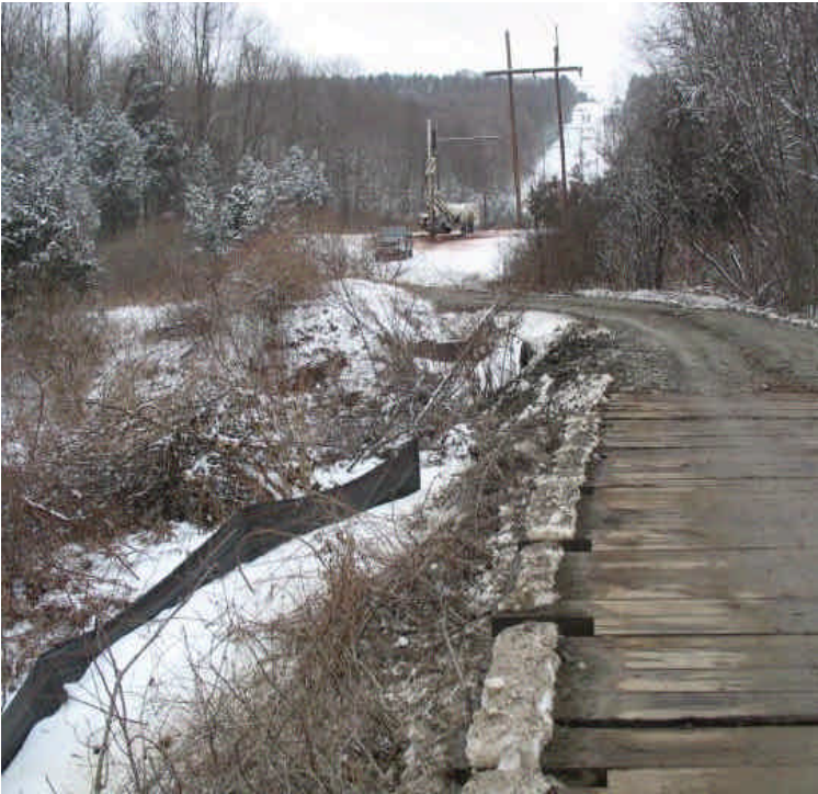
Wetland crossing off Powder Hill Road. No sediment observed Coming from the stone crossing
