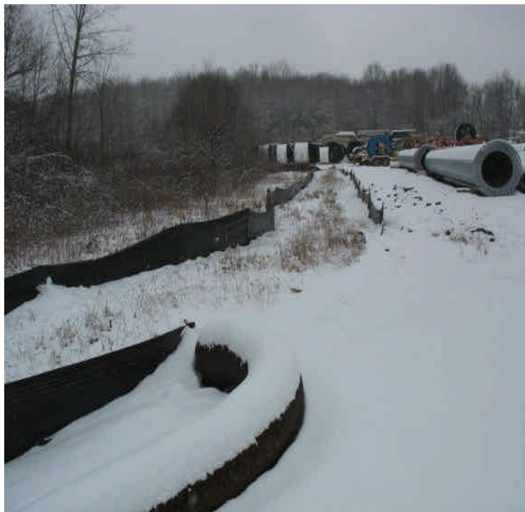
Silt fence, fiber rolls, and hay mulch are in place as a buffer for wetlands around the perimeter of the contractor receiving yard. Replace fallen sections of silt fence and filter sock that was run over.
