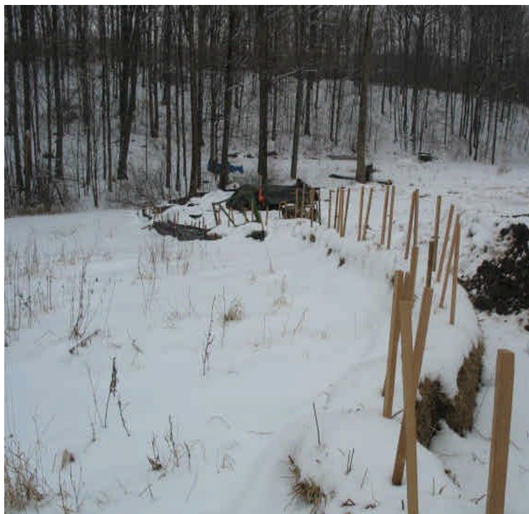
Controls were left in place after drilling the foundation adjacent to to the pond, north of Beseck SS.
