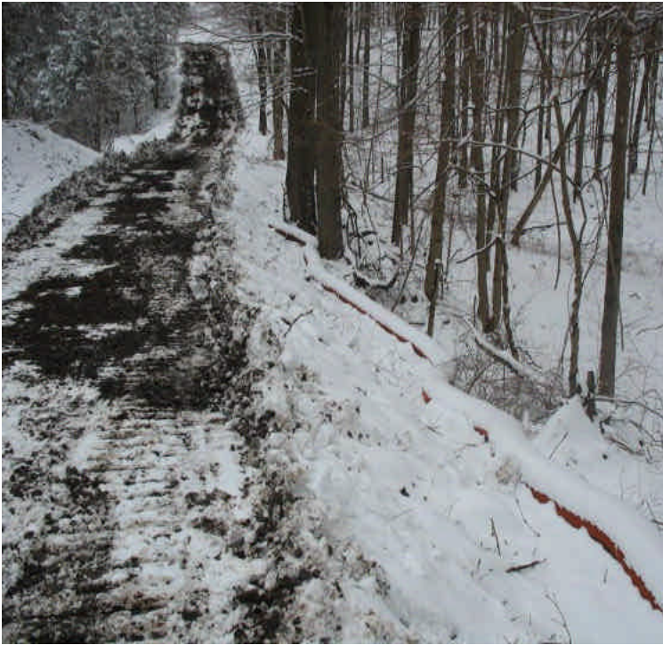
View of access road and culvert in place off Black Walnut Dr. Filter socks were installed along the base of slope of the access road. Continue to monitor to ensure filter socks are controlling run-off appropriately
