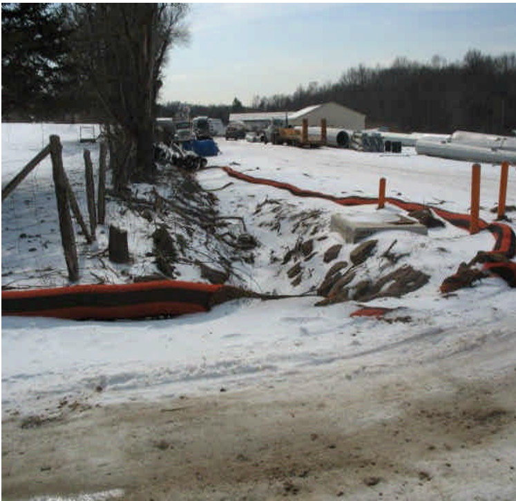
Silt fence, fiber rolls, and hay mulch are in place as a buffer for wetlands around the perimeter of the contractor receiving yard. Replace the section of filter sock that was run over.
