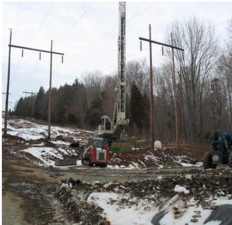
Foundation drilling west of Powder Hill Rd. No active dewatering was noted during the inspection. Controls were in place downgradient. Ensure soils remain contained or temporarily stabilized along these slopes during thaw and snow melt.
