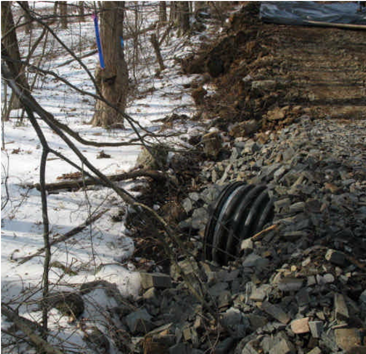
Close-up view of culvert installation off Black Walnut Dr. Ensure water bars and/or silt fence are installed along the access road base of slope to protect wetlands.
