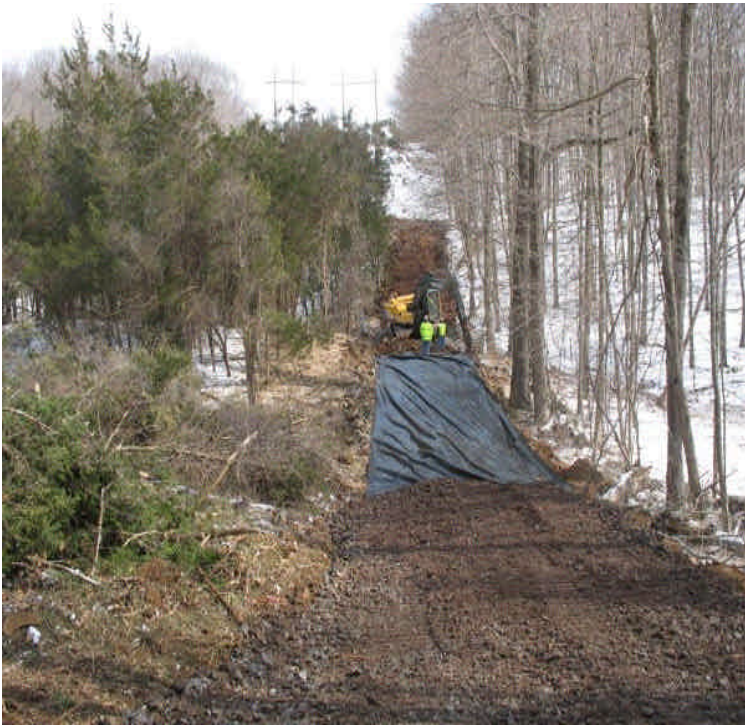
Additional view of access road and culvert installation off Black Walnut Dr.
