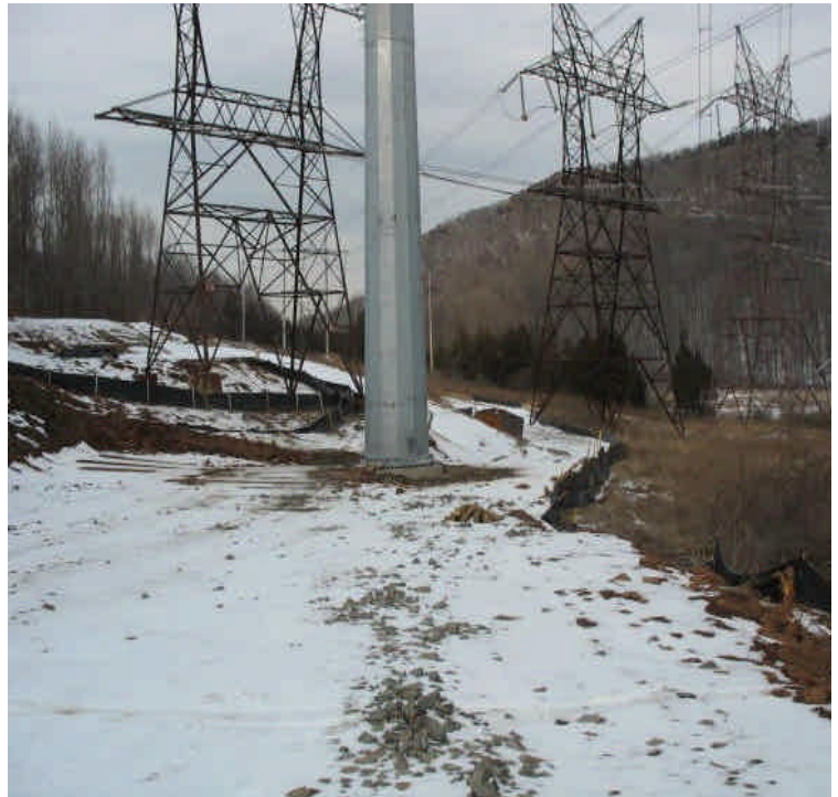
View of mono-pole and controls at Black Pond. Controls are intact and look good.
