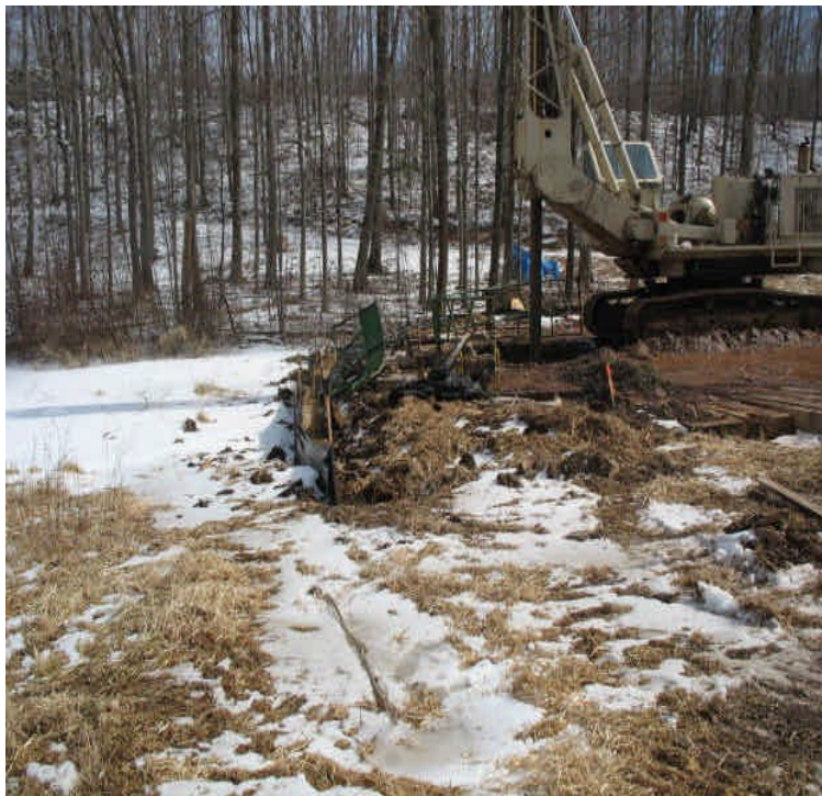
Foundation drilling along the ROW north of the Beseck SS. Controls were in place to prevent sediment from entering the wetlands but any dewatering should be monitored carefully here.
