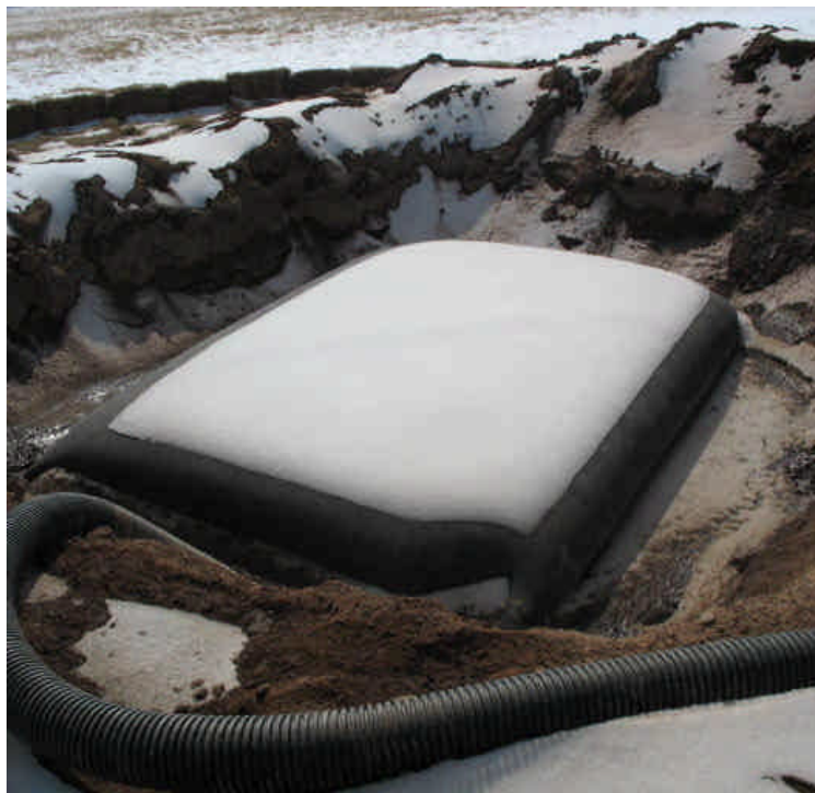
Filter bag and containment basins are in place for dewatering foundation work. Controls are in good shape.
