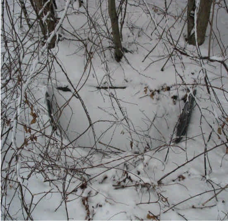
View of the culvert under the access drive. No sediment issues have been observed. Heavy snow cover is present.
