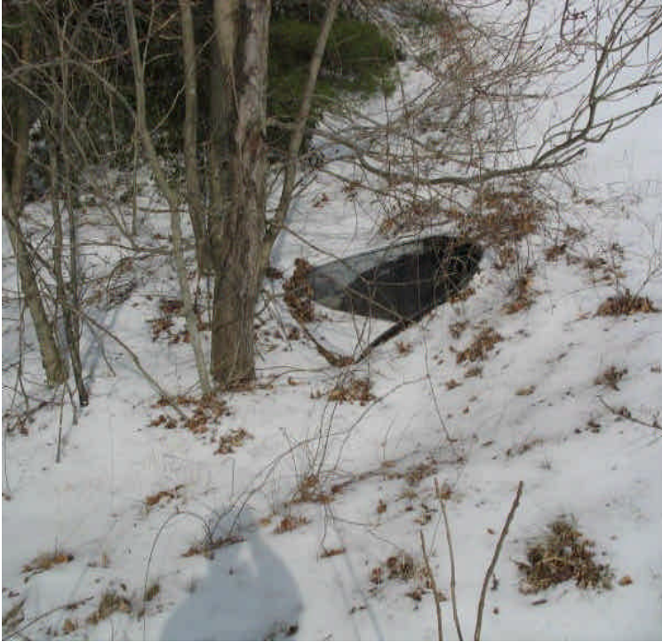
View of the culvert under the access drive. No sediment issues have been observed.
