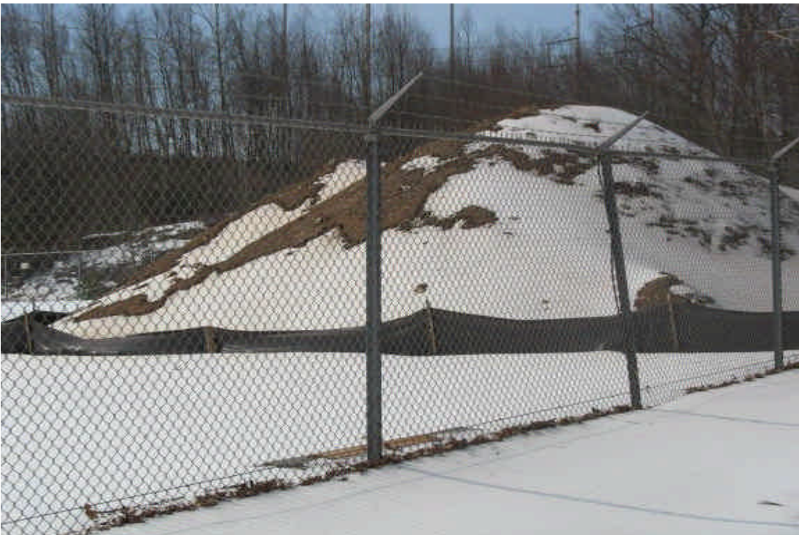
Soil stockpile to be removed with controls in place. No sediment issues have been observed.
