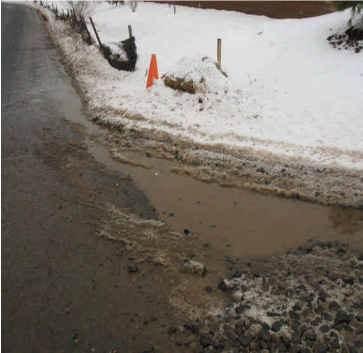
Site entrance/exit off Carpenter Lane is at final grade; erosion controls are intact along the driveway. Minor amounts of turbid run-off were noted reaching the roadway.
