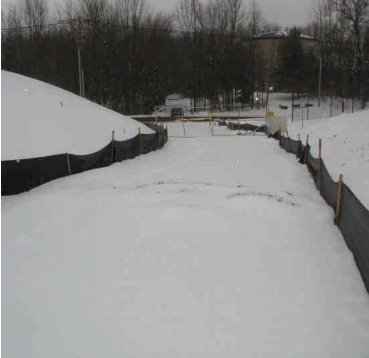
Another view of the closed site entrance where a water bar was installed in an effort to divert turbid run-off from leaving the site.
