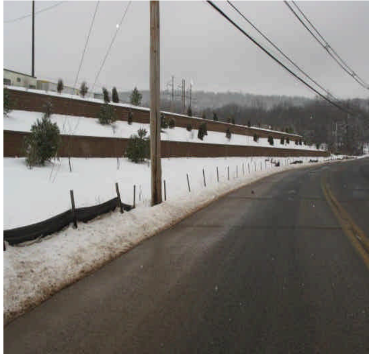
View of Carpenter Lane and retaining walls. Sand accumulation was noted along the gutters from town sanders but is not a result of the project. However, catch basins controls could use maintenance.
