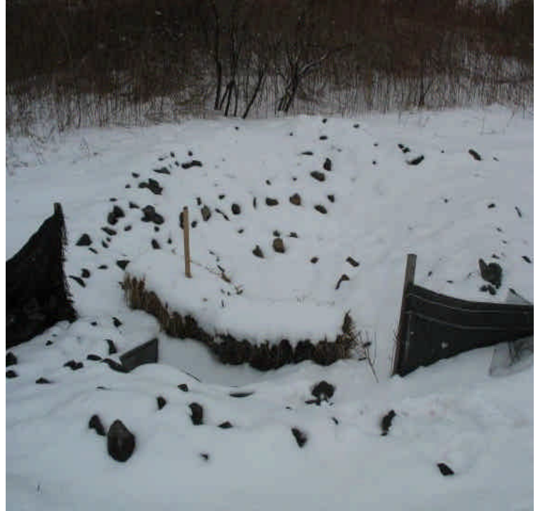
View of the culvert under the new access road. Turbid water from last week has since filtered out of the trap. Sediment appears contained within the trap.
