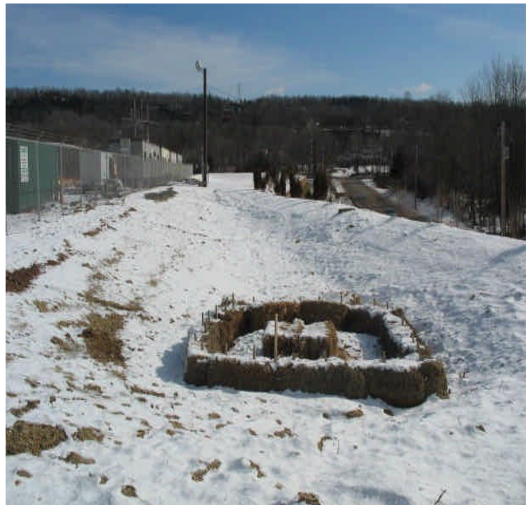
Surface areas on site are temporarily stabilized with tackified hydroseed and as a result of freezing temperatures. Haybales are in place at the inlet and no run-off was noted this week.
