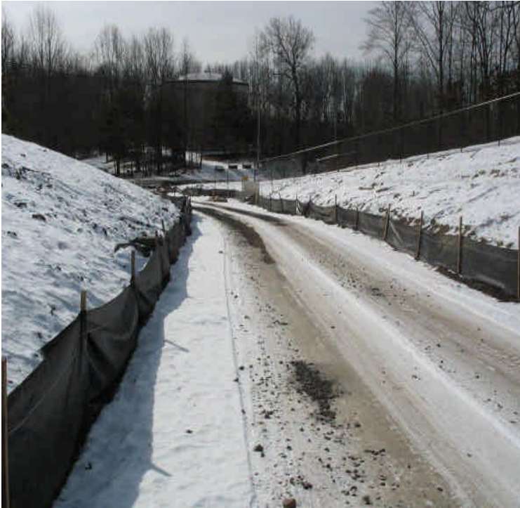
Site entrance off Carpenter Lane is at final grade; erosion controls are intact along the driveway. Monitor carefully for run-off.
