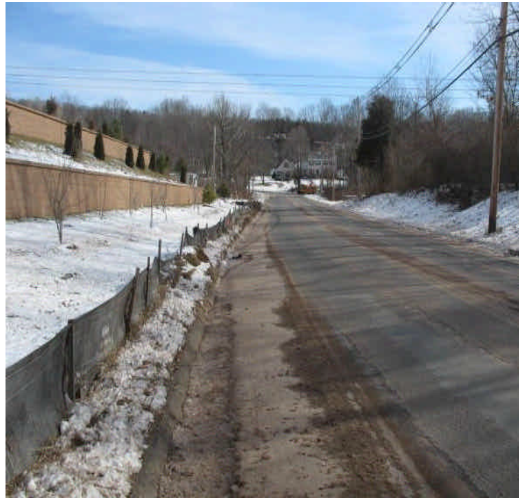
View of Carpenter Lane and retaining walls. Sand accumulation was noted along the gutters from town plows and sanders but is not a result of the project. Gutter buddies were removed from the catch basins during plowing but liners are in place.
