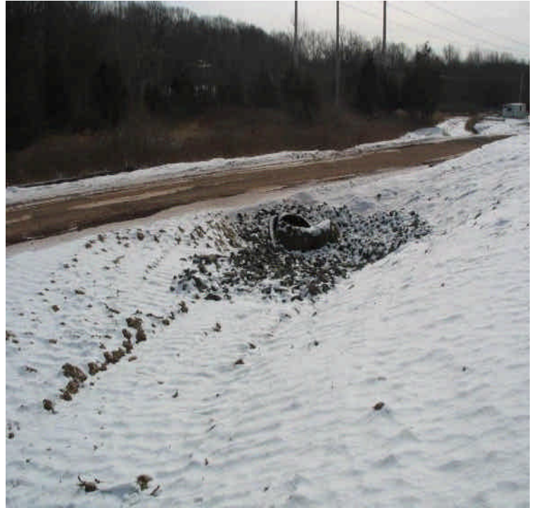
View of the culvert under the new access road. A minor amount of sediment was noted but appears well contained within the trap. Beseck and Seg. 1A contractors are jointly sharing the access road.
