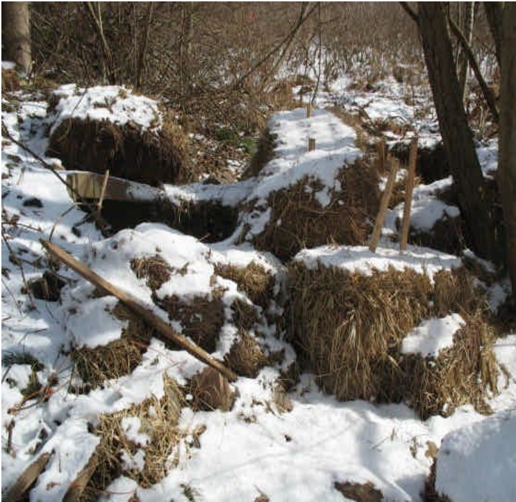
Sediment appears to have settled out at the storm drain outlet across Carpenter Lane. Ice was observed in the culvert but sedimentation was not apparent. The additional efforts on site appear to be effective at reducing sediment. Continue to monitor.
