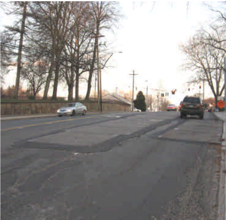
Photo taken on Rt 1 looking towards N. Compo Rd. at the trenching activities.
