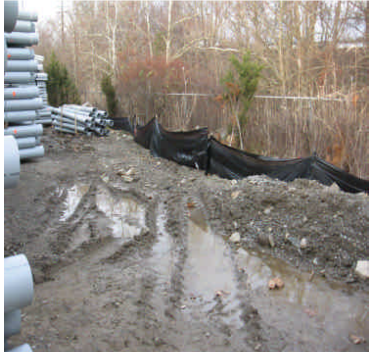
The portion of perimeter silt fence along the side of the yard adjacent to the sensitive area was repaired as recommended
