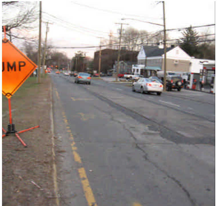
Photo of trenching activities on Rt. 1 near its intersection with Long Lots Rd.
