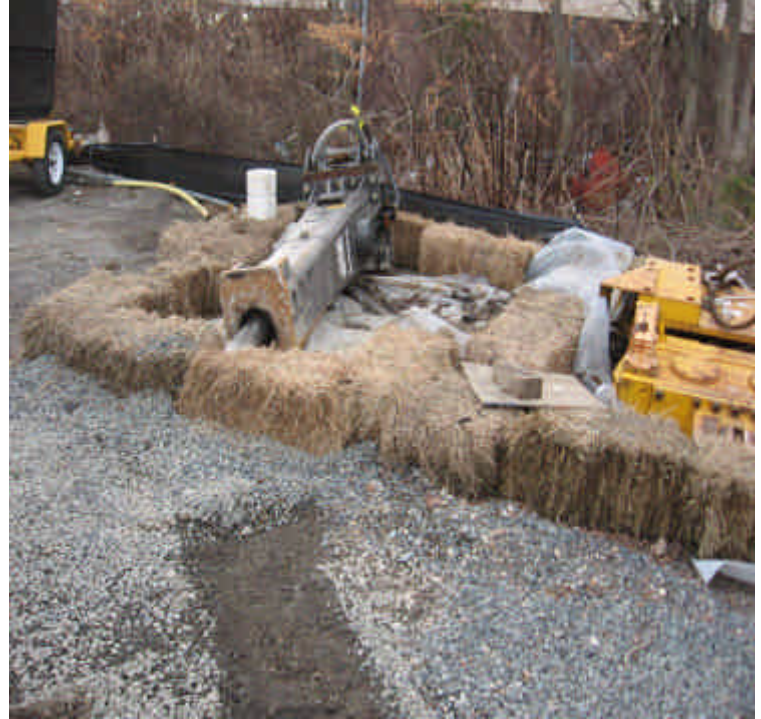
Equipment attachment storage area has now been fully enclosed with controls as recommended.
