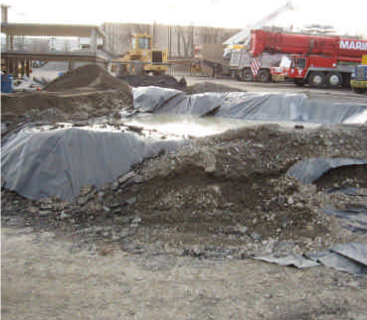
Newly constructed concrete washout basin that is properly lined with fabric and has additional storage capacity.
