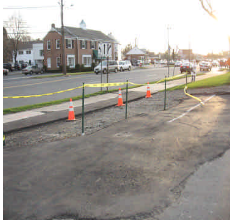
Photo of Vault #7536 location remains to be restored, but is temporarily stabilized.
