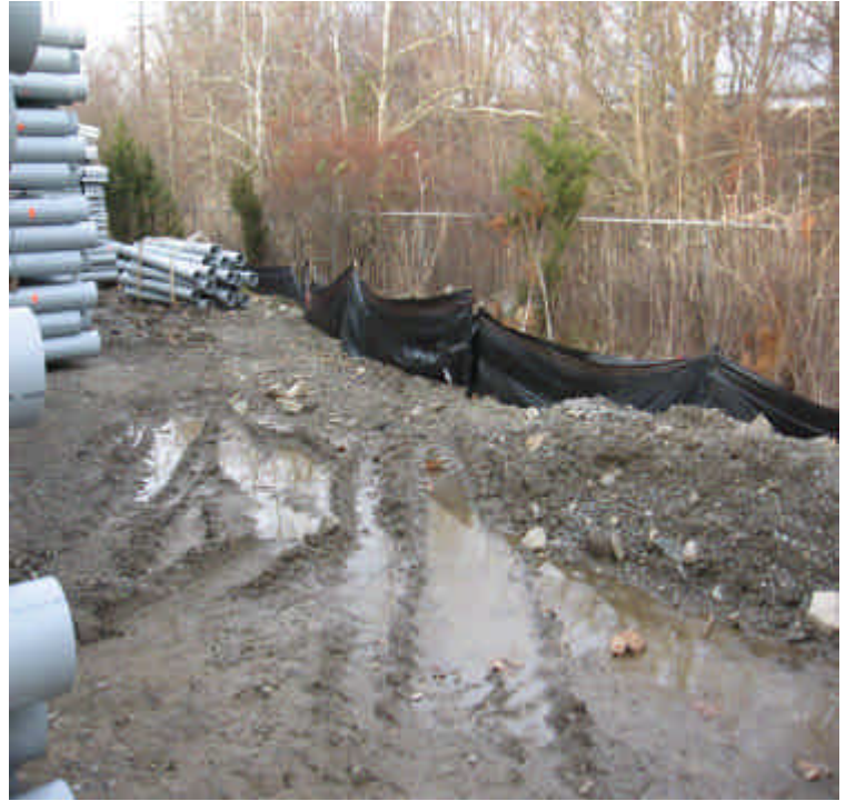
The portion of perimeter silt fence along the side of the yard adjacent to the sensitive area was repaired as recommended since the last inspection.
