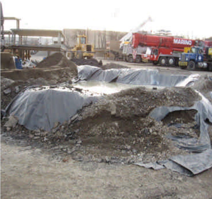
Newly constructed concrete washout basin that is properly lined with fabric and has additional storage capacity.
