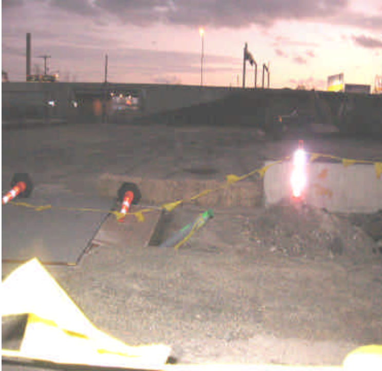
Photo taken from Railroad Ave. of trenching activities near its intersection with Bostwick Ave. Private storage yard with catch basin downgradient of activities is in background. A line of haybales have been placed between construction activities and catch basin to prevent sedimentation.
