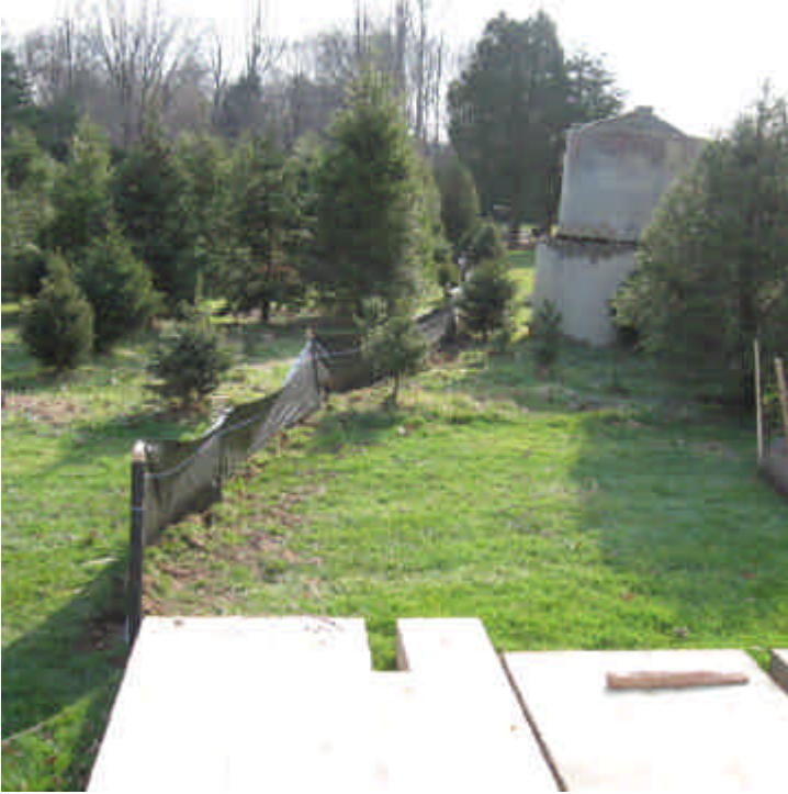
Silt fence was installed upgradient of the wetland near the tree farm located within the ROW off Overland Drive (east).
