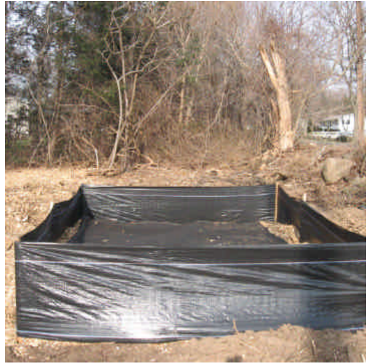
Dewatering containment areas were proactively placed within the ROW off Ridge Road.
