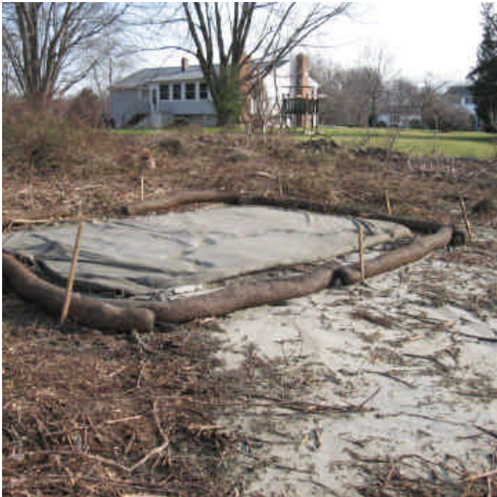
View of the dewatering area located within the ROW off Overland Drive (west). Sediment/slurry has flowed beyond the controls here.
