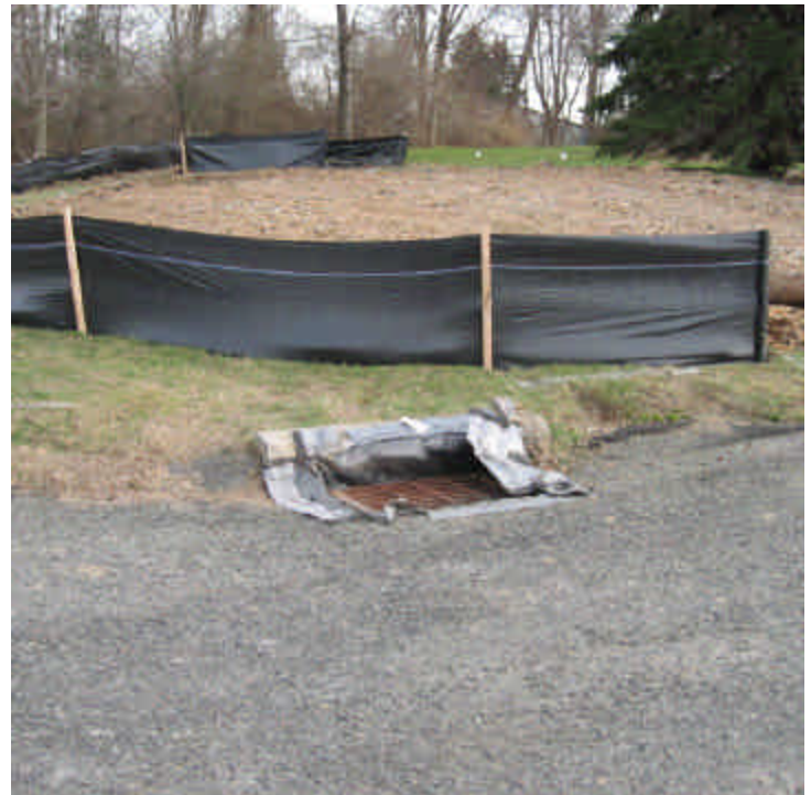
A silt sack, completely protecting the catch basin and curb drop inlet, has been installed at the intersection of Saddle Ridge Road and Harbor View Place. Silt fence was also in place here.
