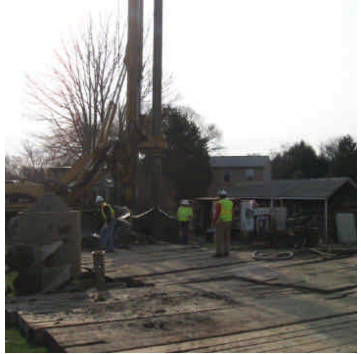
Foundation drilling continues off Overland Drive (east). Timber mats were used where necessary.
