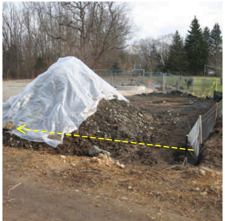
Silt fence was installed between the stockpile and NFJ wetland within the ROW off Sunset Dr. The silt fence should be extended towards Sunset, along the access road.
