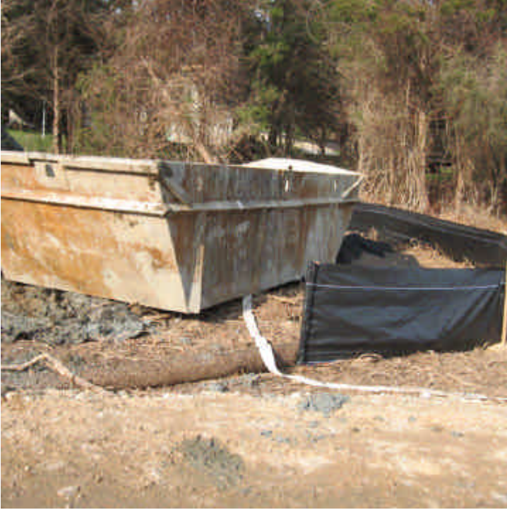
View of the dewatering area within the ROW located off Overland Drive (east). Foundation drilling and pouring continues here.
