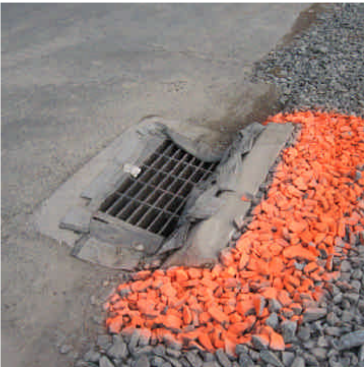
The catch basin on Sunset Drive remains protected. No sediment tracking was observed here this week.
