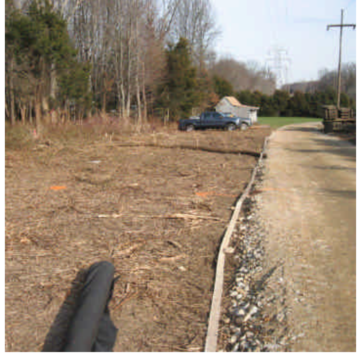
View of the filter sock check dams installed within the ROW off Overland Drive (east).
