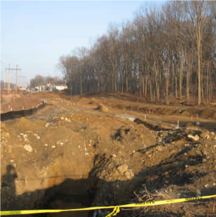
View of the work associated with the relocation of Shelland Street in Milford. All exposed soil and sediment is contained on site.
