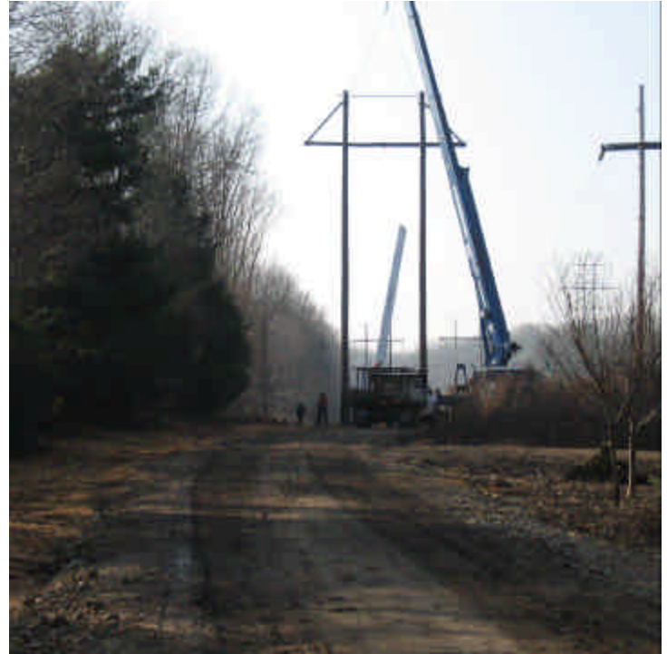
Crews were removing existing H-frame structures within the ROW off Route 152 (west) at the time of inspection.
