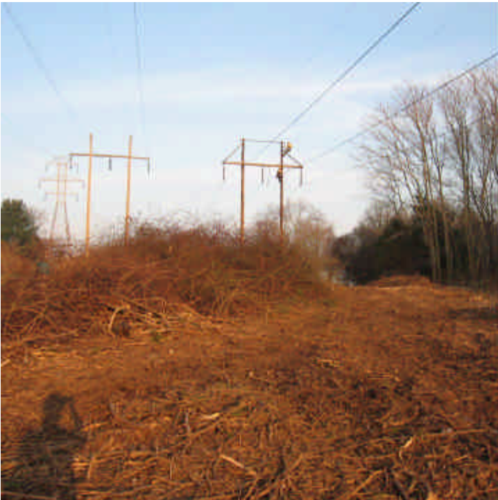
View of the clearing within the ROW off Rolling Ridge Road. Shrubs were retained where feasible.
