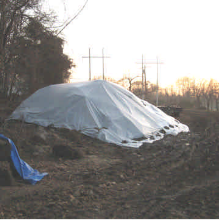
All spoil piles stored within the ROW off Russell Ave have been covered with plastic. Foundation drilling/pouring is nearly complete.
