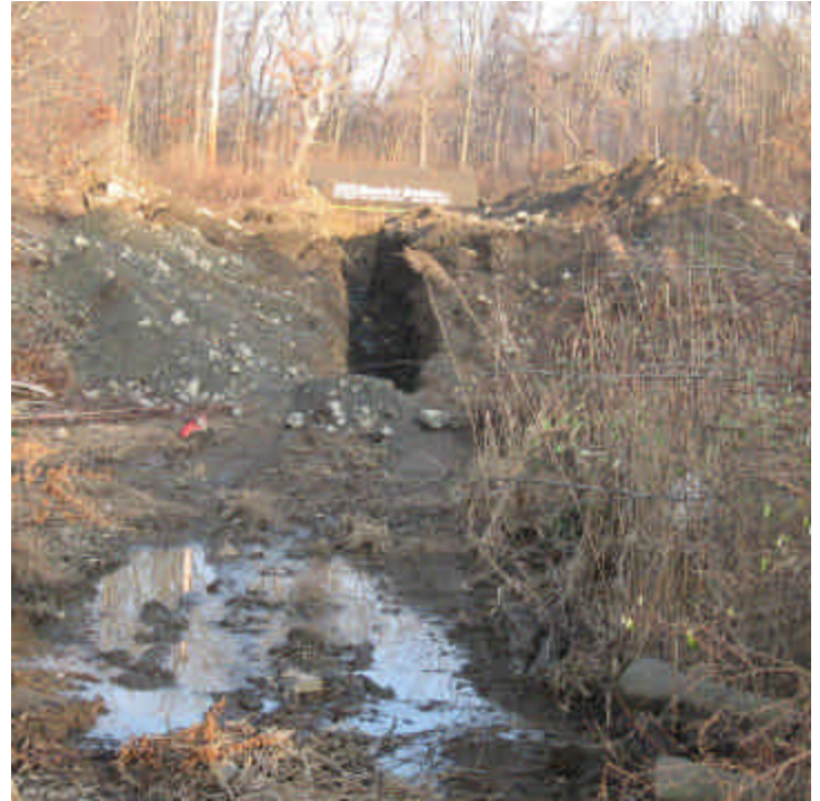
Site preparation associated with the proposed East Devon Substation continues near Shelland Street. All exposed soil and sediment is contained on site.
