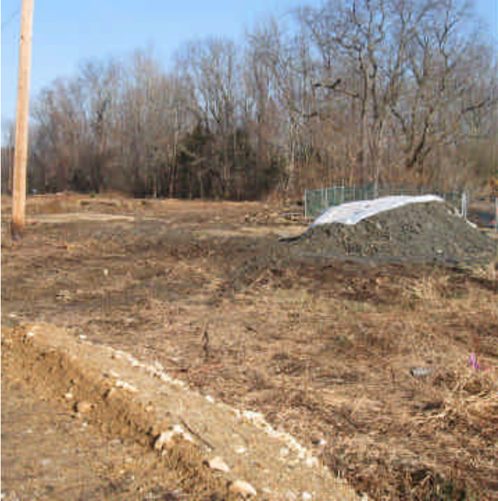
View of the partially covered stockpile located near the NFJ wetland within the ROW off Sunset Drive. Silt fence or additional controls should be installed here.
