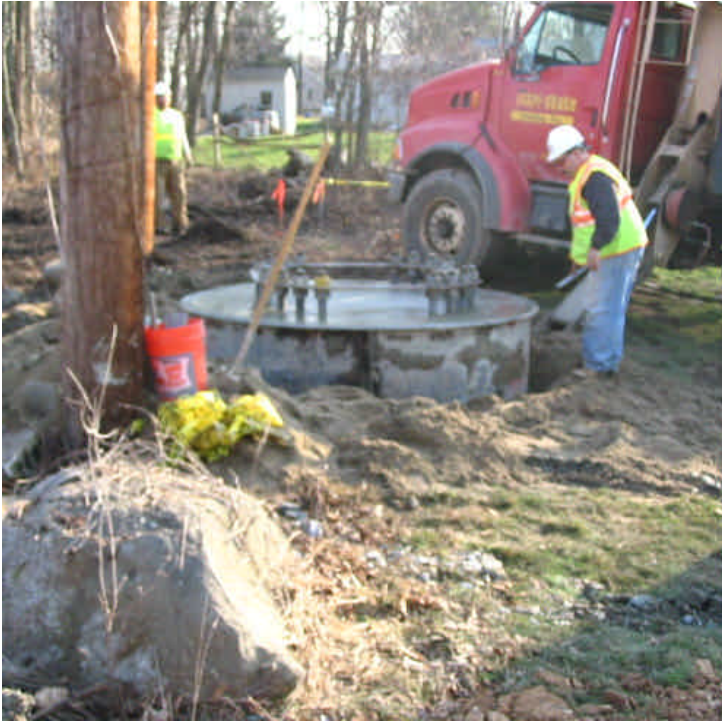
View of the foundation installed at the second proposed structure location off Russell Ave.
