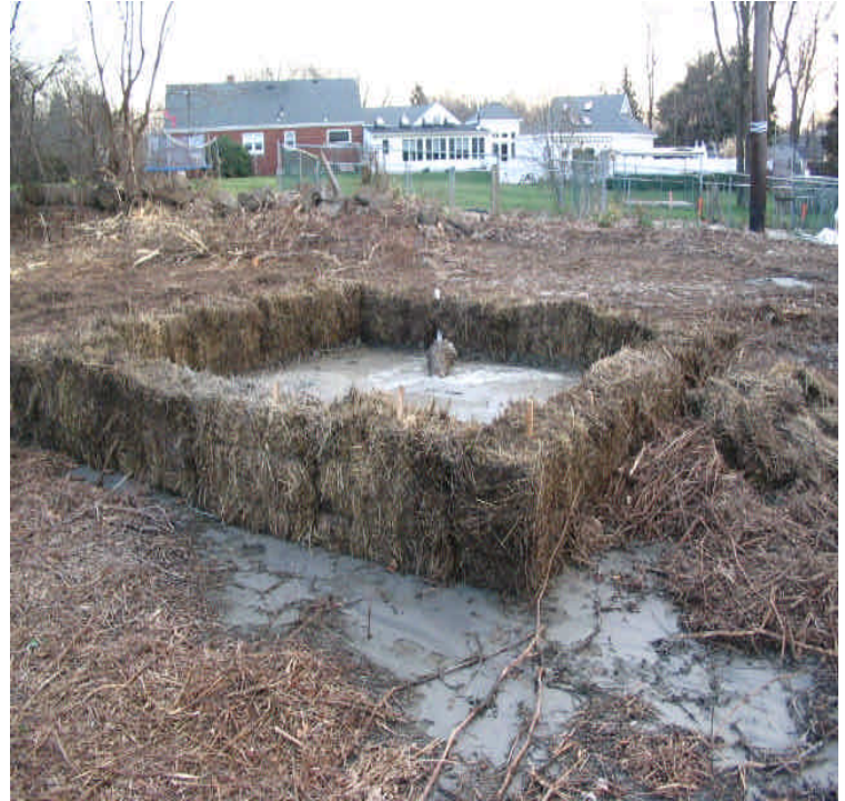
View of the dewatering area near the second proposed structure location off Sunset Dr. A filter bag was not used here, allowing sediment/slurry to escape and flow in the direction of the wetland.
