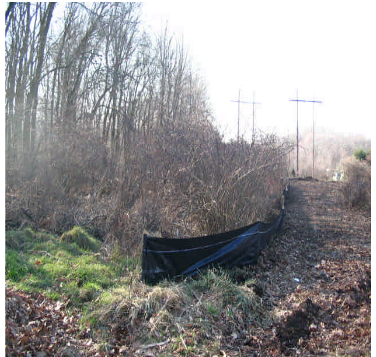
Silt fence was installed along the wetland located within the ROW off Orange Center Road/Route 152 (west). Clearing and access road construction continue in this area.
