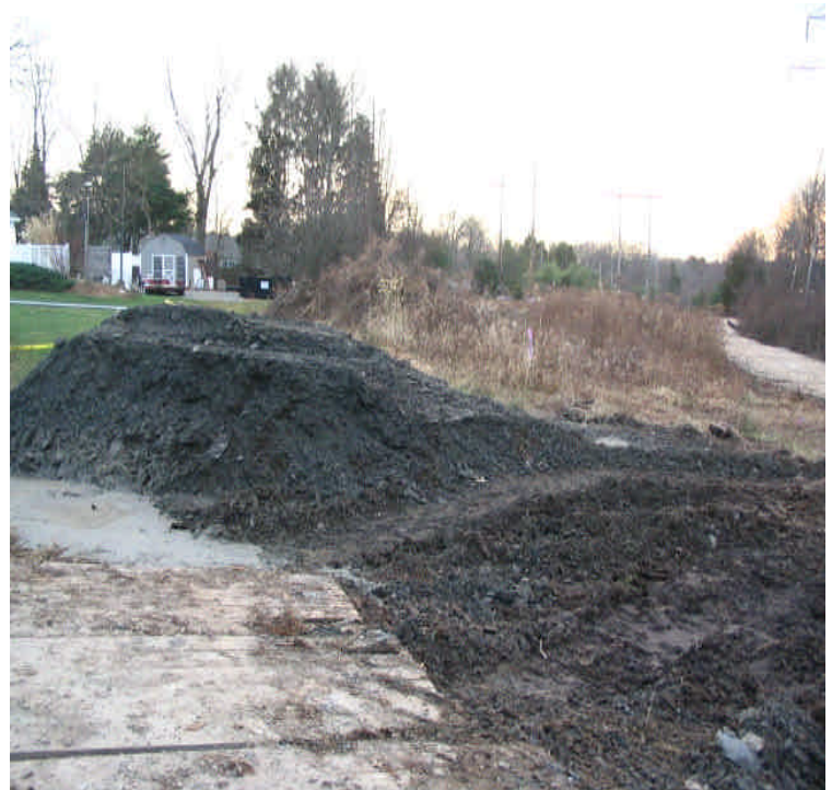
View of the stockpile stored near the wetland off Sunset Drive. Erosion controls should be installed downgradient of the pile to contain potential sedimentation.
