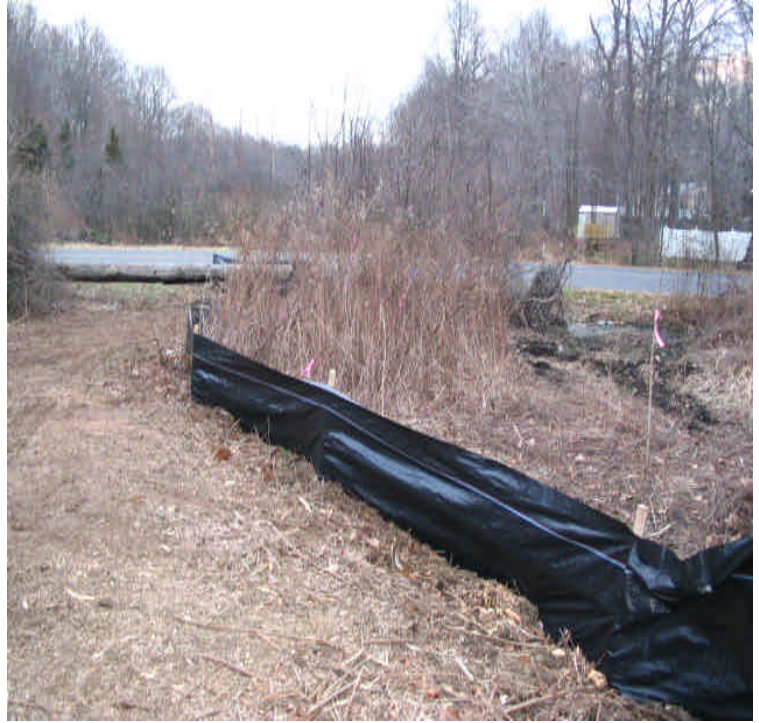
View of the silt fence installed at the wetland within the ROW off Pine Tree Drive (west). Clearing was noted here.
