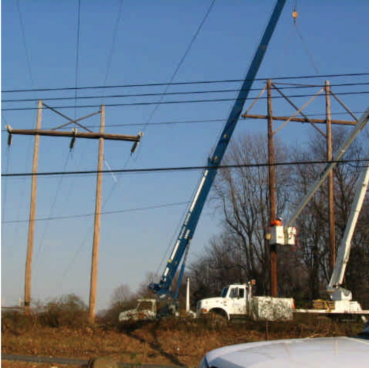
Crews were in the process of removing the existing H-frame structures from the ROW off Dogwood Road (east).
