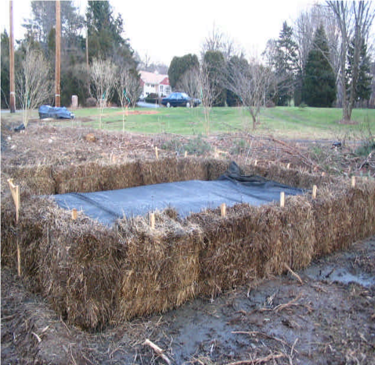
View of the dewatering area placed near the first proposed structure location off Sunset Dr. The filter bag, in combination with the haybales, was effective in retaining sediment prior to releasing the water.
