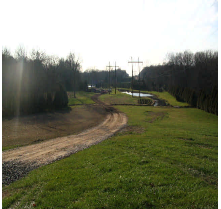
View of the new access road constructed within the ROW off Dogwood Road (west).
