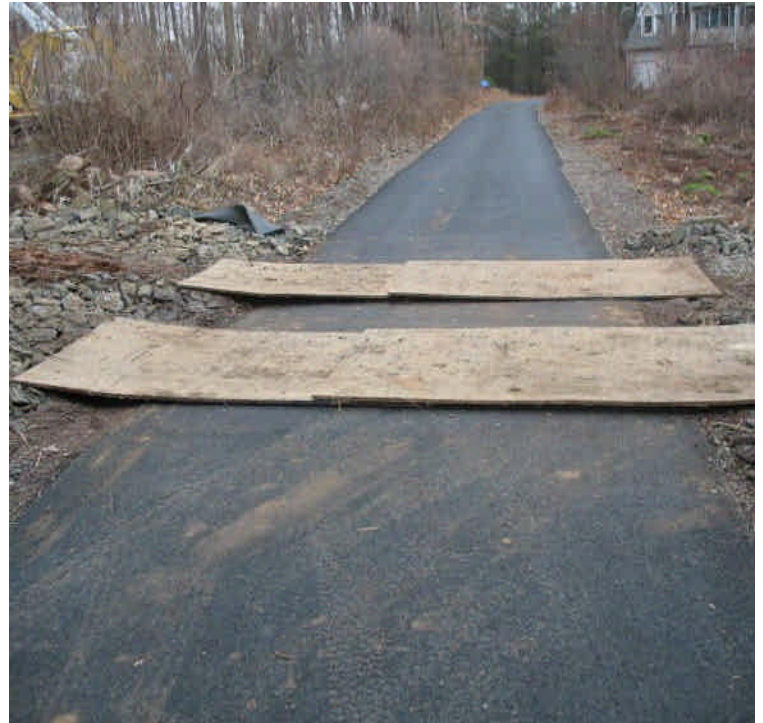
Plywood installed to protect driveways from equipment crossing on the ROW off Old Farm Rd. Minimal sediment tracking was noted.
