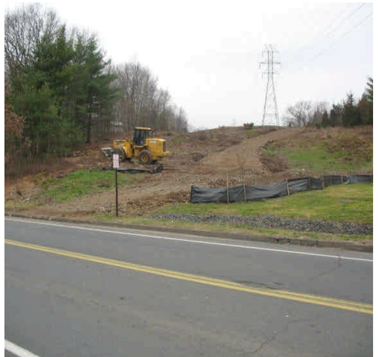
Eroded gullies/washouts were repaired; the new access road and silt fence were installed off South Turnpike. Continue to monitor this slope for run-off issues.
