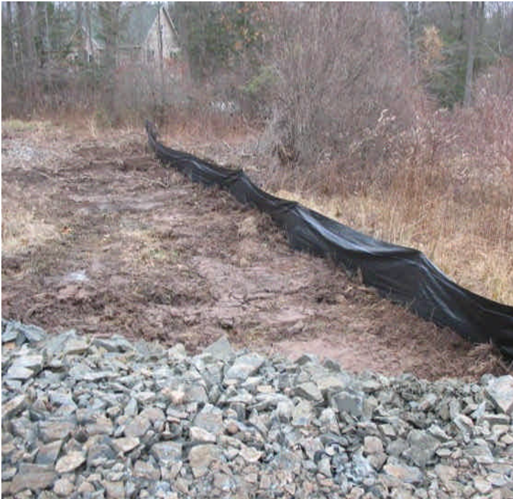
Silt fence installed upgradient from the non-federally jurisdictional wetland finger off Old Farm Rd.
