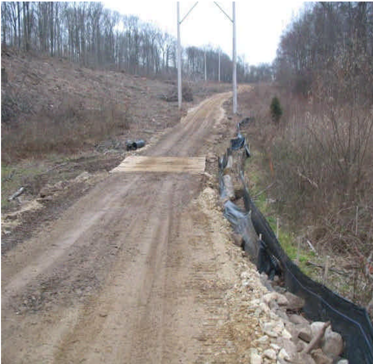
New access road, mats, and erosion controls off High Hill Rd at a non-jurisdictional wetland crossing
