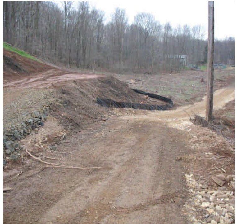
New staging areas prepared for pole construction. Temporary stabilization measures were added.
