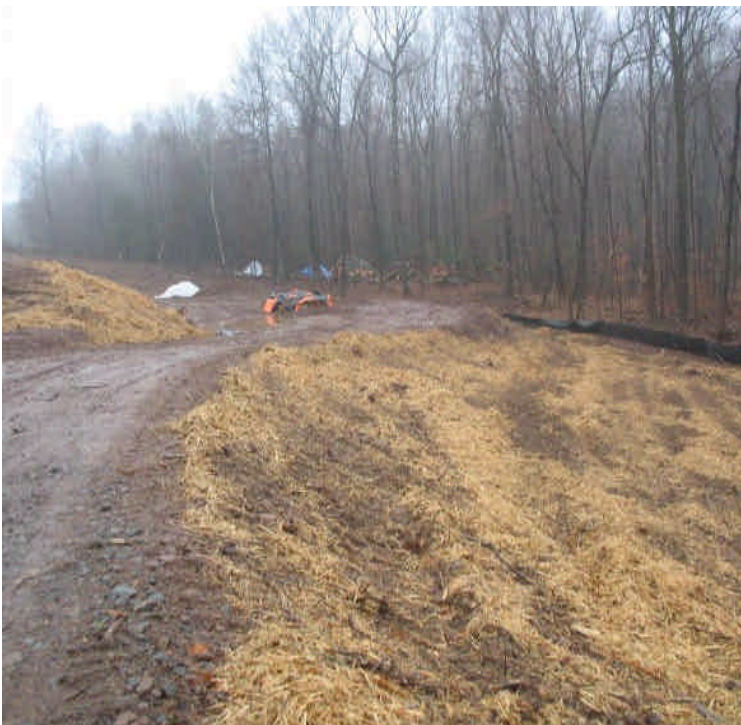
Foundations installed within the ROW north of Beseck SS. Controls are in place.
