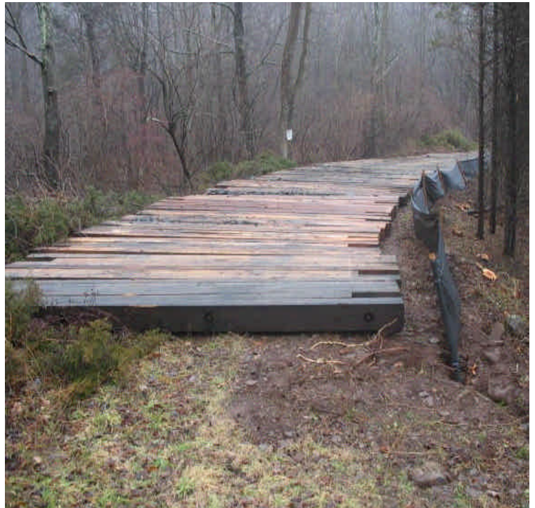
Silt fence and timber mat installation along an existing access road off Powder Hill Rd. The installation follows an existing road through a wetland and was determined to be maintenance by the contractor. Silt fence protects an existing pond adjacent to the access road.
