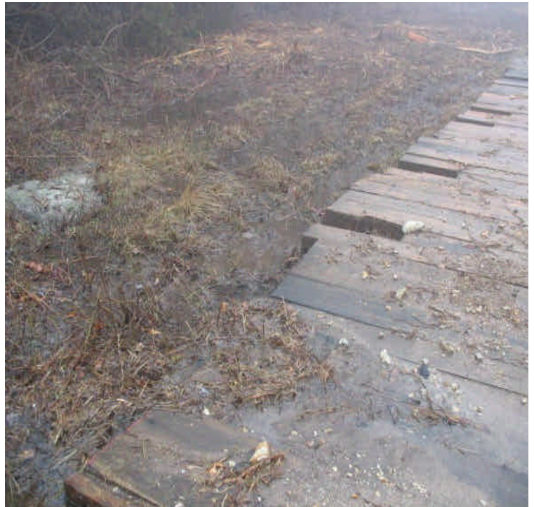
Non-jurisdictional wetland crossing area in the access ROW off Haddam Quarter Rd. Mats are in place and clean water was leaving the site. Reduce sediment tracking on the mat as feasible.
