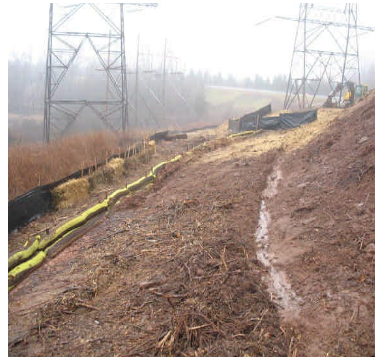
Silt fence/filter-sock barrier along the access road adjacent to Black Pond used for dewatering slurry. Slurry has been pulled back from the controls and spread around the site.
