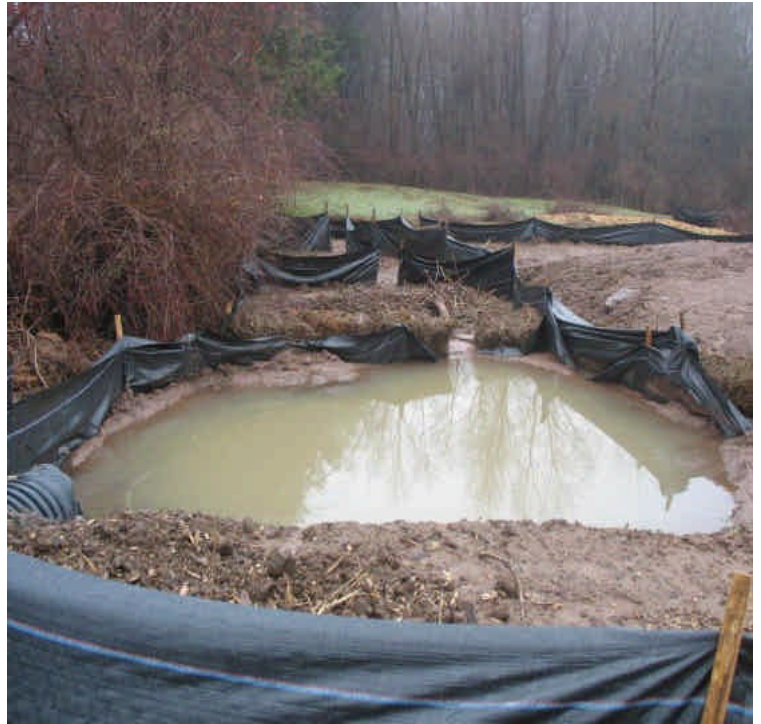
Slurry containment areas located in the ROW north of the contractor yard along Rte 17. Sediment was removed and stormwater contained.
