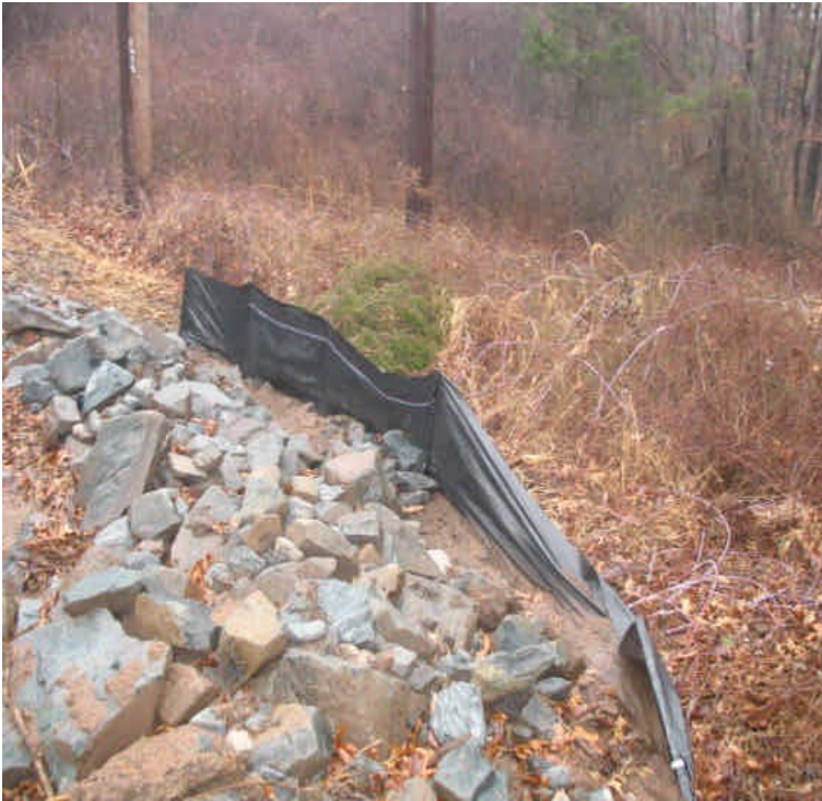
Riprap sediment trap and silt fence along the access road off Black Walnut Drive. Accumulated sediment should be removed and the silt fence maintained.
