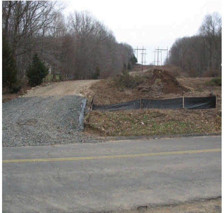
Silt fence, clearing, grading, and access road off Arbutus Street. Pull back stone from the roadway as needed.
