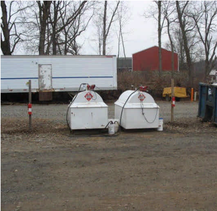
Nozzles for the fuel tank have been placed inside of 5-gallon buckets with spill controls at the contractor yard. Fire extinguishers were installed
