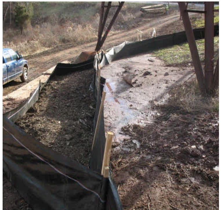
Silt fence/haybale barrier along the access road adjacent to Black Pond used for dewatering slurry. Slurry remains contained.
