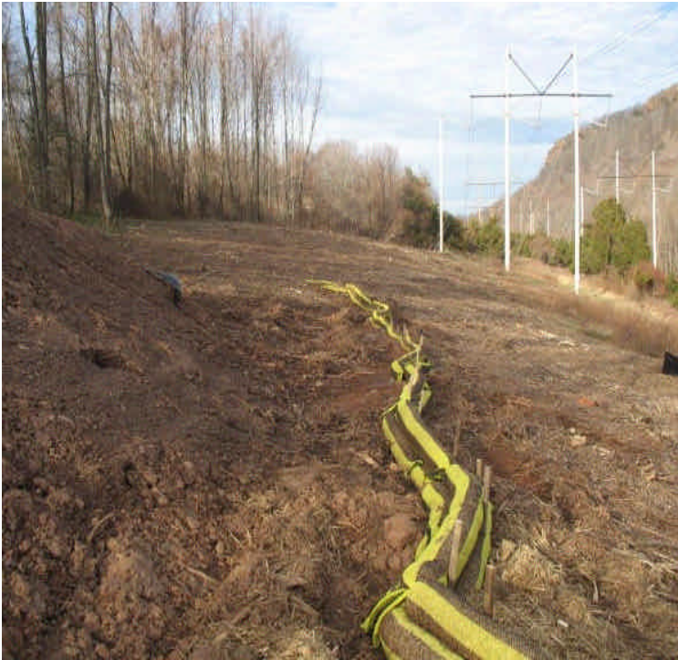
Bio-socks used to trap/filter slurry and sediment from dewatering efforts at Black Pond.
