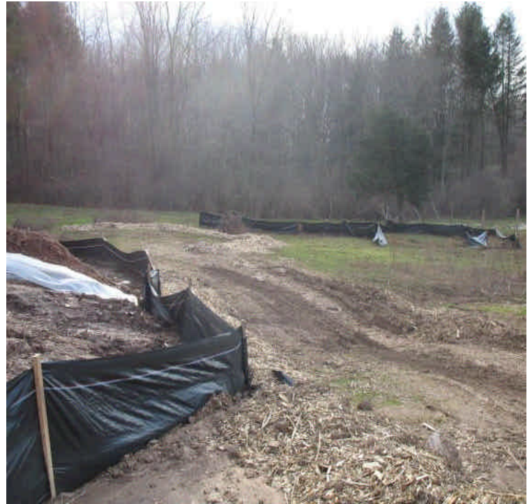
Slurry containment areas located in the ROW north of the contractor yard along Rte 17. Sediment is being removed and spread, and is mostly dry at this time.
