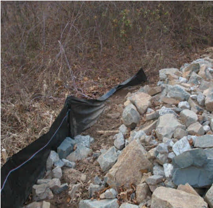
Riprap sediment trap and silt fence along the access road off Black Walnut Dr. Accumulated sediment should be removed and the silt fence repaired.
