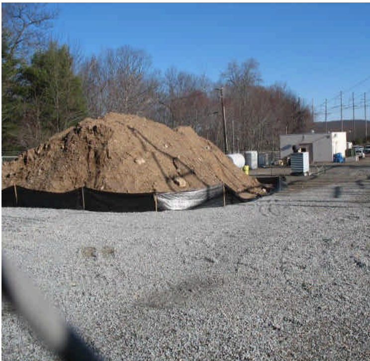
The remaining soil stockpile is surrounded by silt fence. Repair fallen section of silt fence and remove soil from site when feasible.
