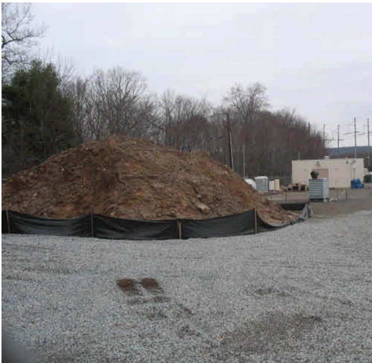
The remaining soil stockpile is surrounded by silt fence. Fix fallen section of silt fence and remove soil from site when feasible.
