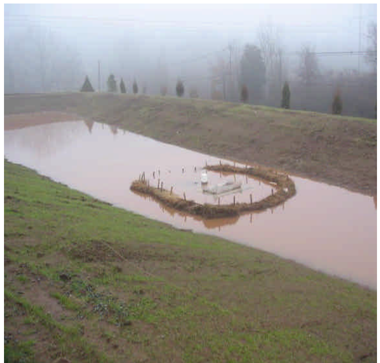
Additional/alternative controls are still recommended. Turbid water from dewatering activities has overtopped the controls at the inlet. Consider additional filtration/containment for dewatering discharge as well.
