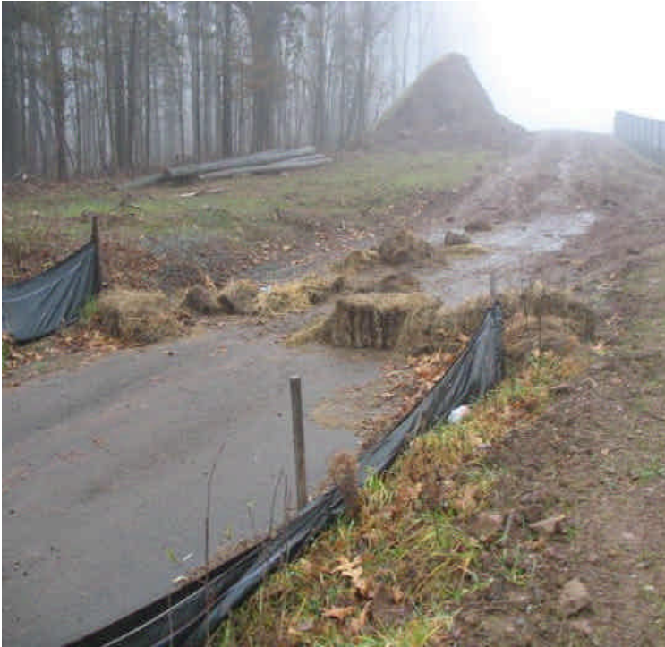
Replace haybales across the old Zolnik driveway. Adjacent areas have been graded and seeded.
