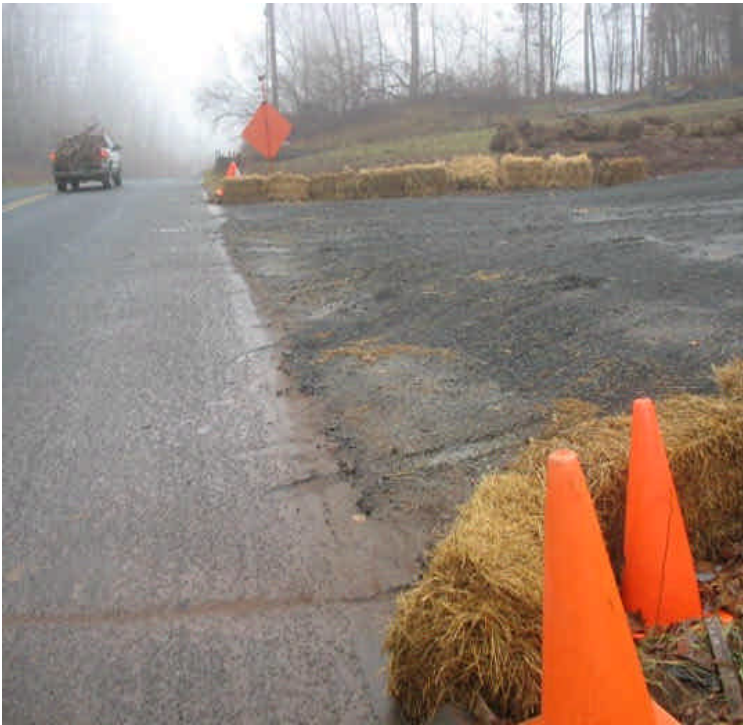
New entrance off Carpenter Lane at final grade; erosion controls have been removed. Monitor carefully for run-off.
