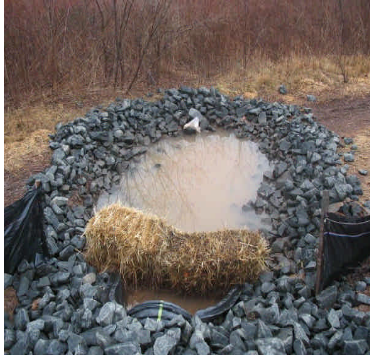
View of the culvert under the new access road. Some minor amounts of turbid water were noted but appears contained within the trap. Beseck and Seg. 1A contractors are jointly sharing the access road.
