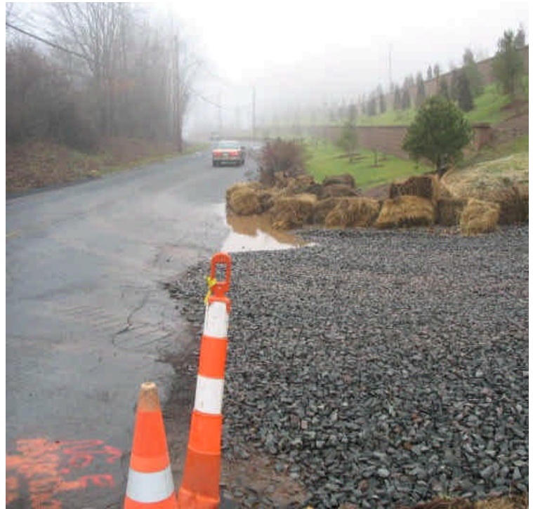
View of Carpenter Lane and retaining walls. Sediment accumulation was noted in the gutters. Turbid water was observed flowing past the controls at the site entrance.
