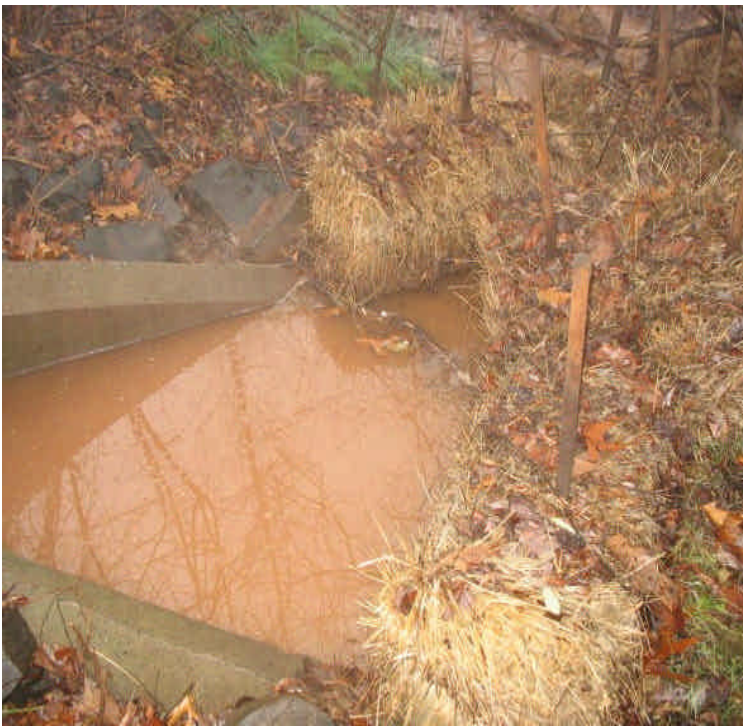
Storm drain outlet across Carpenter Lane again had turbid water flowing through the outlet pipe and past the degraded haybales into the wetland. New haybales and alternative controls on-site are needed.
