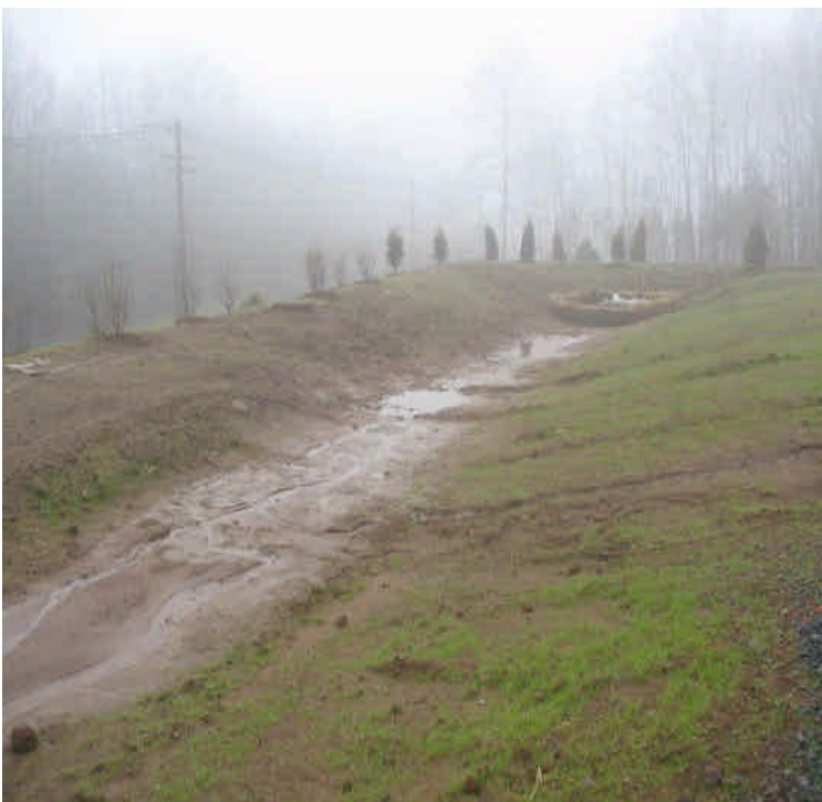
Some grass has become established in the western detention basin. No water was pumped into this basin.
