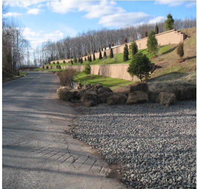
View of Carpenter Lane and retaining walls. Minor sediment accumulation was noted in the gutters on the north side of the road. This should be swept by hand to prevent entry into the catch basins.
