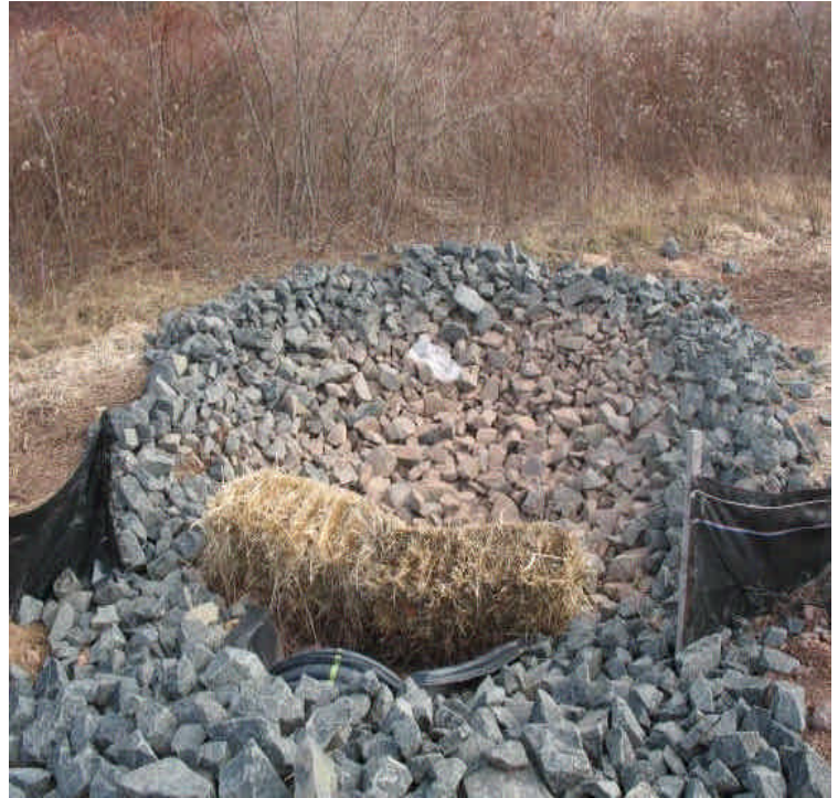
View of the culvert under the new access road. Some minor sediment was noted but was well contained in the trap. Beseck and Seg. 1A contractors are jointly sharing the access road.
