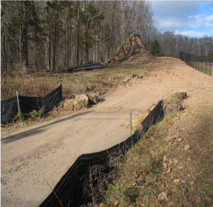
Replace haybales across the old Zolnik driveway (they had been moved for access). Adjacent areas have been graded and seeded.
