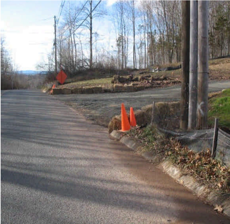
New entrance off Carpenter Lane at final grade, erosion controls have been removed. Monitor carefully for run-off.
