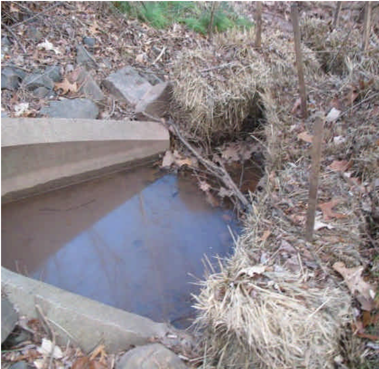
Storm drain outlet across Carpenter Lane contained settled sediment with clear standing water at the outlet pipe. The haybale configuration could still use some adjustment for better control.
