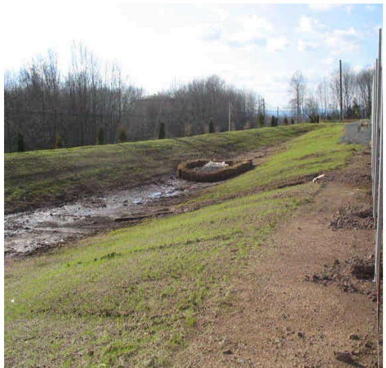
Some grass growth was observed on the seeded side slopes of the detention basins. Additional/alternative controls are still recommended to protect the inlet as turbid water may pool over and into the drain inlet.
