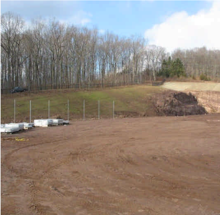
Grass growth observed on slopes during the warmer weather. Fence installation in progress.
