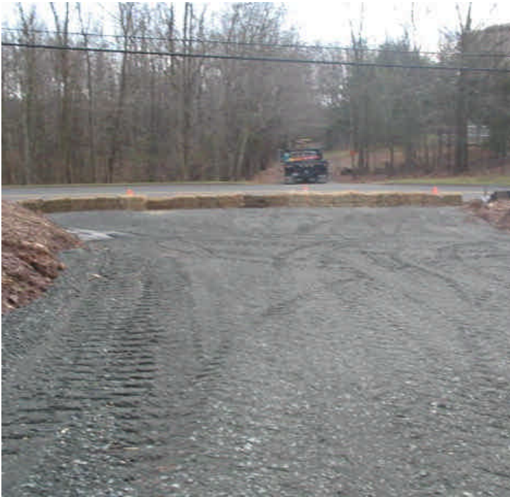
New entrance off Carpenter Lane at final grade with haybale barrier in place.
