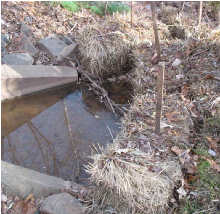
Storm drain outlet across Carpenter Lane contained settled sediment with clear standing water at the outlet pipe.
