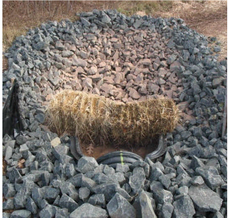
View of the culvert under the new access road. Some minor sediment was noted but was well contained in the trap. Beseck and Seg. 1A contractors are sharing the joint access road.
