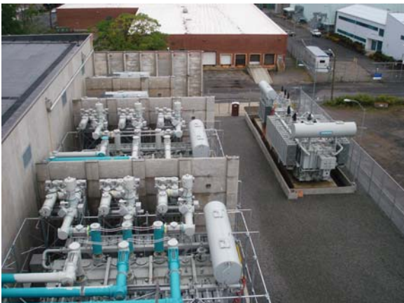
Outdoor 345kV GIS Equipment
