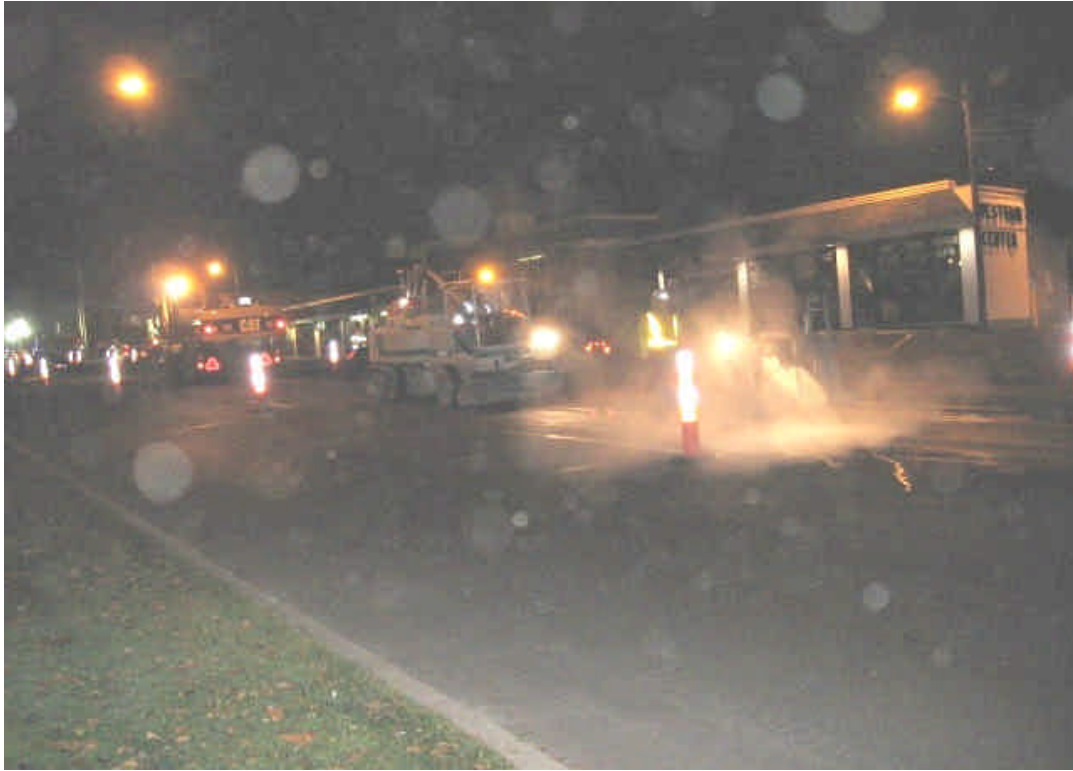
Photo of trenching and saw cutting activities in Westport from Buckley Ave. to Westfair Dr. Please note that sweeper truck is immediately following saw cutting activity to remove sediment from the roadway.
