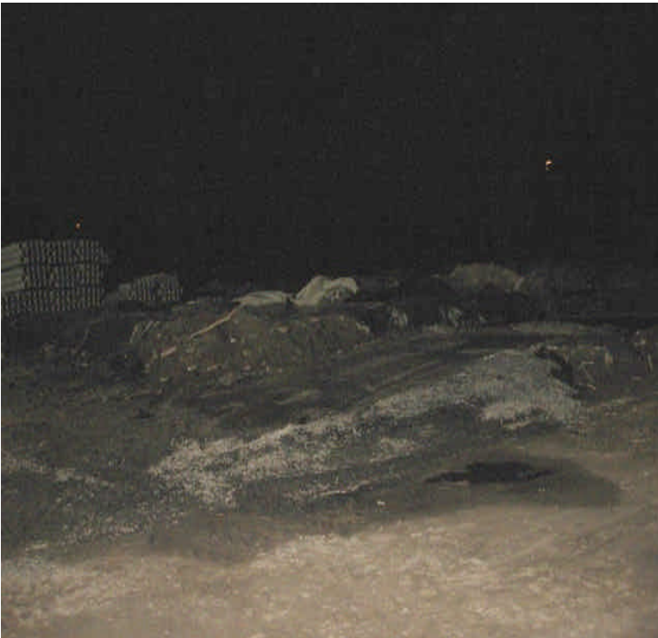
Sweeper washout area being overwhelmed and the concrete washout area is at capacity. All materials remain contained to the yard.
