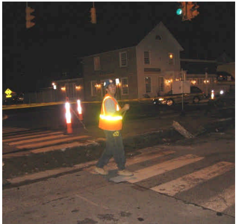
Photo of Rt. 1 trenching activities. Roadway being swept immediately following excavation of trench.
