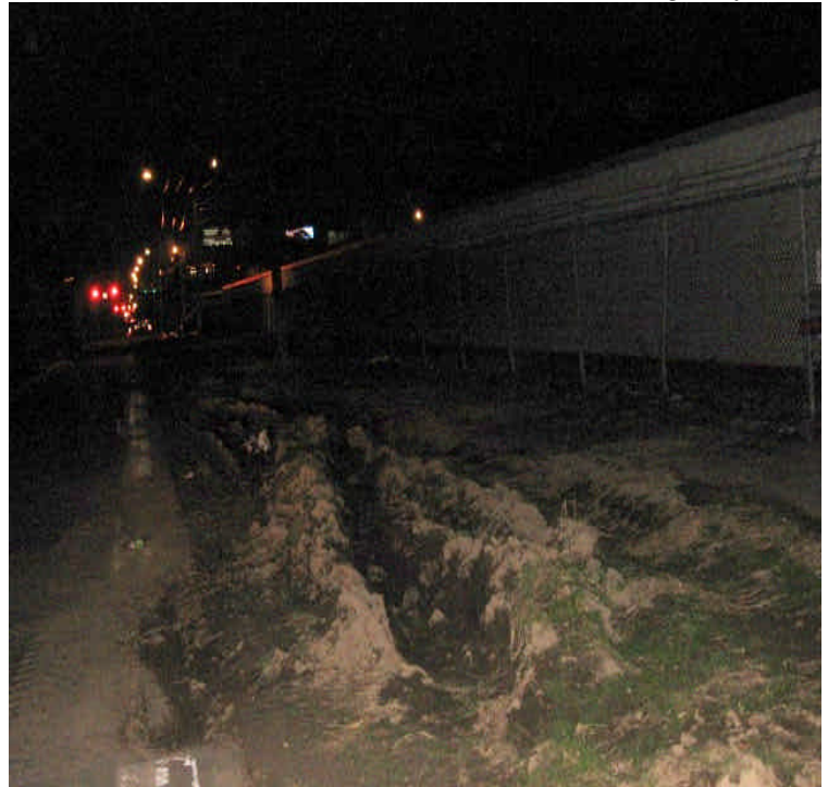
Photograph taken on Railroad Ave. near its intersection with Wordin Ave. of former trench location that has tire tracks. Tire ruts should be regraded and the area temporarily stabilized.
