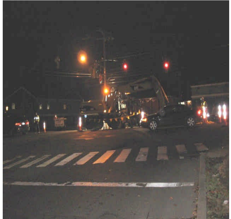
Photograph taken from Mill Plain Rd. of trenching activities of on Rt. 1. Just behind photo is an overpass with two unprotected catch basins on Mill Plain Rd. that need controls.
