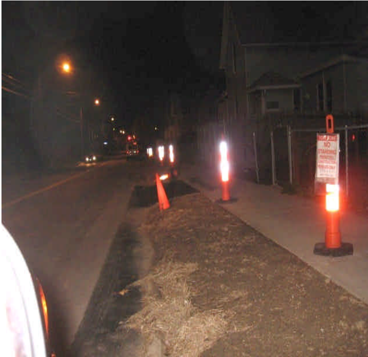
Former trench location on Broad Street that had hay mulch sparsely applied or that had blown away. Mulch should be re-applied and possibly tackified to protect exposed soils.
