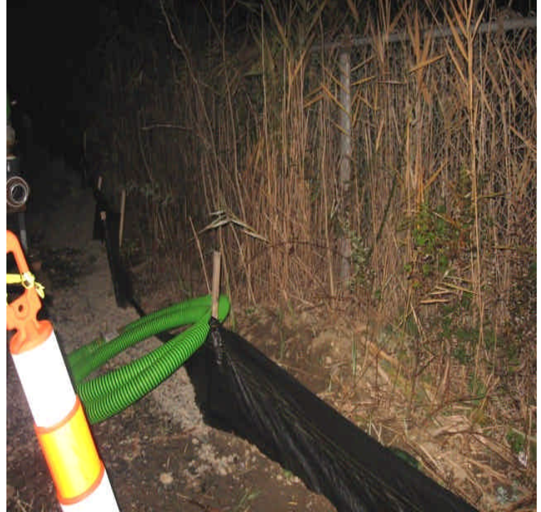
Erosion controls adjacent to resource area, and along the boundary of the yard are being compromised by stored materials.
