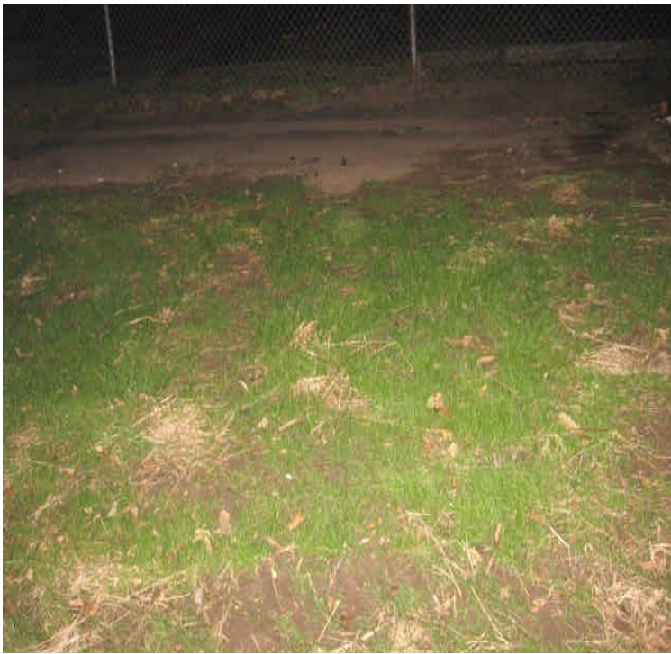
Former trench location on Railroad Ave that has temporarily stabilized with grass.
