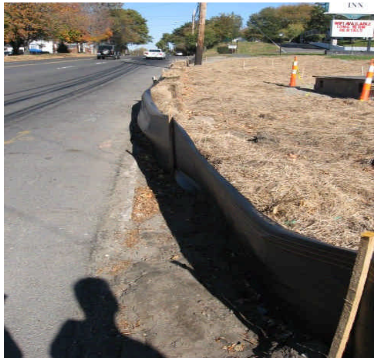
Photo of Rt. 1 and the Fairfield Inn construction area that previously experienced erosion. Area should be monitored during rain events to prevent any additional sedimentation.
