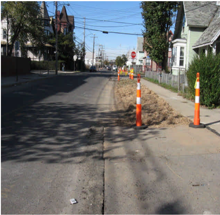
Former trench location on Broad St. that has been temporarily stabilized with hay mulch.
