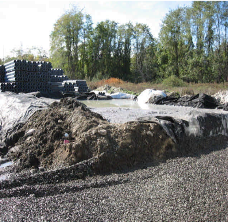
Concrete washout basin located within yard that is near capacity.
