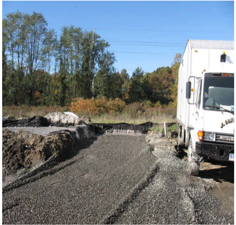
Sweeper washout area within yard is being contained.
