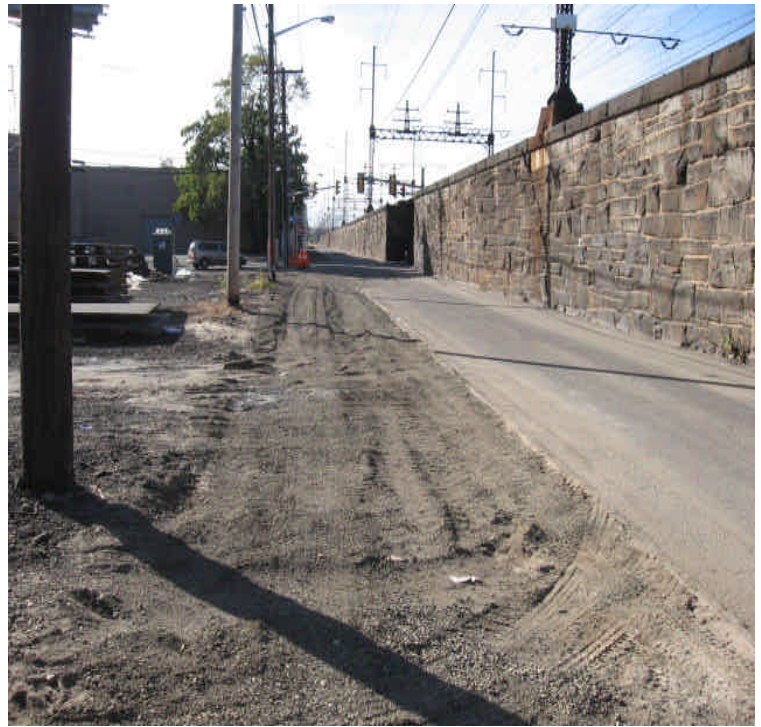
Photo taken on Railroad Ave. at the corner of Iranistan Ave. Former trench location has been closed and stabilized with stone.
