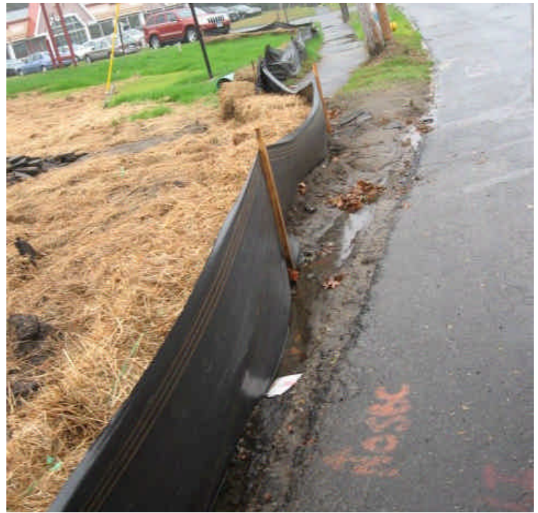
Photo of Rt. 1 in front of Fairfield Inn. Sediment in roadway has been removed. Eroded area remains between the roadway and the silt fence to be stabilized.
