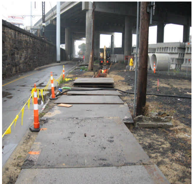
Trenching activities on Railroad Ave. near its intersection with Iranistan Ave. Area to the right is being used to temporarily store materials and frac tanks.
