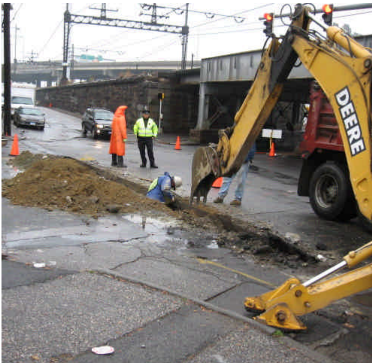
Photo of trenching activities at the intersection of Railroad Ave. and Park Ave.
