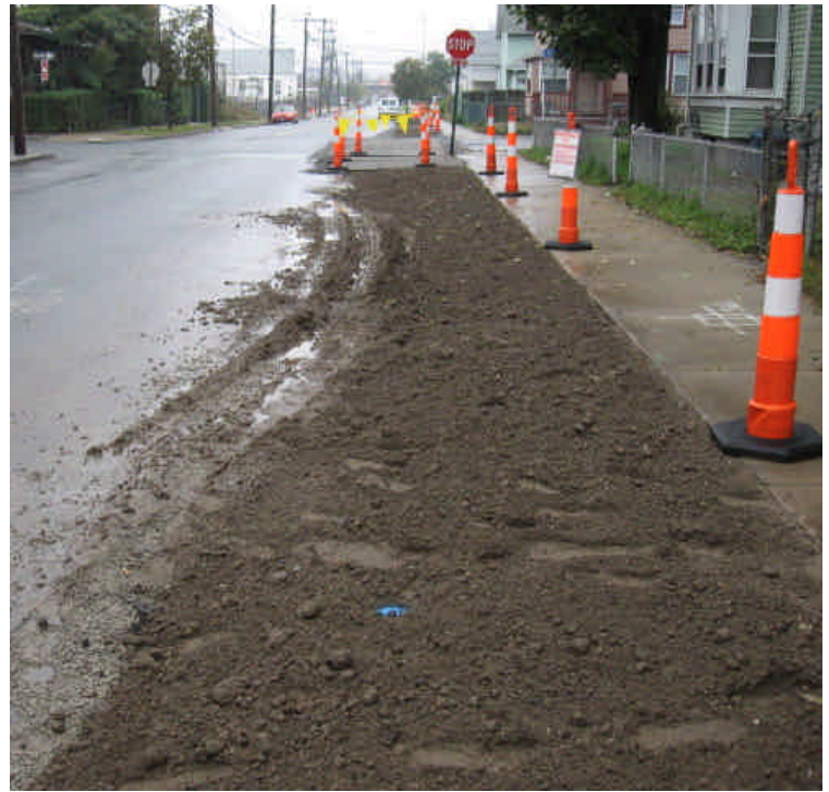
Former trench location that has been backfilled and loamed. The area should be temporarily stabilized with mulch.
