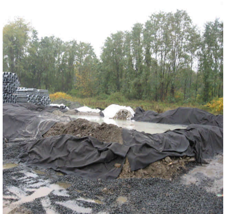
Concrete washout basin located in the Kings Highway Yard Laydown is near capacity and should be emptied when possible.
