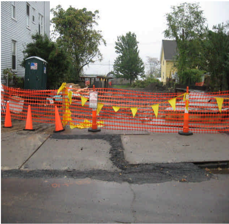
Former location of garage/shed on Broad St. that has been removed for utility installation.
