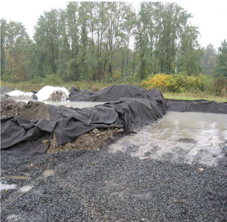
Sweeper washout area located in the Kings Highway Laydown has been re-established so that all washout materials are contained.
