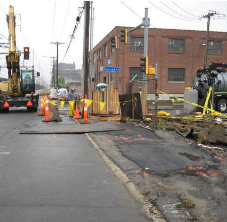
Trenching activities at the intersection of Railroad Ave. and Bostwick Ave. Vac truck is being used to excavate around utilities.
