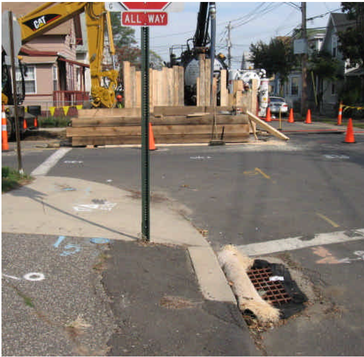
Trenching activities at the intersection of Atlantic Ave. and Broad St. Please note protected catch basin.
