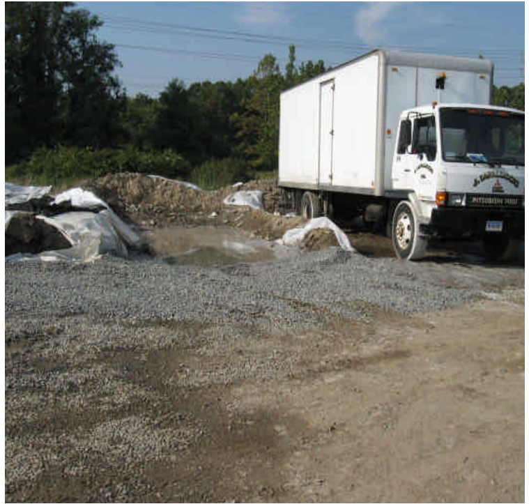
Sweeper washout area is not containing all of the washout materials to the basin. Run-off (potentially saw cutting cast-off) is located under, and in front of the right front tire of the box truck.
