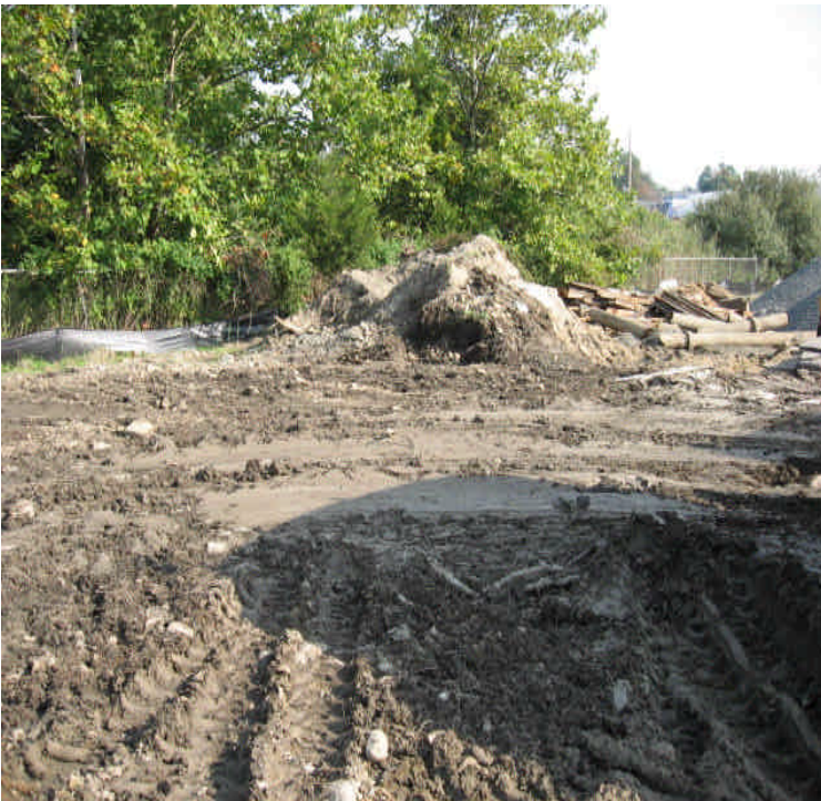
Previous location of original concrete washout basin. The soil pile should be located away from the perimeter fence
