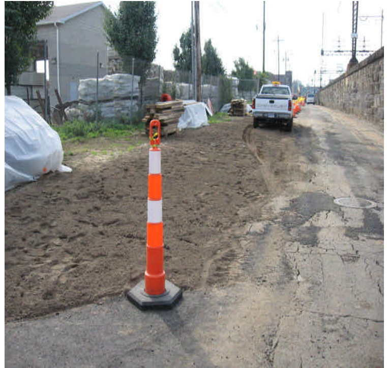
Portion of backfilled trench along Railroad Ave. near Howard Ave. It is anticipated that the area will be seeded and mulched within the week.
