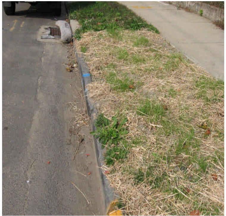
Location of previously excavated area for utility work on Broad St. Please note that grass is starting to establish in the area.
