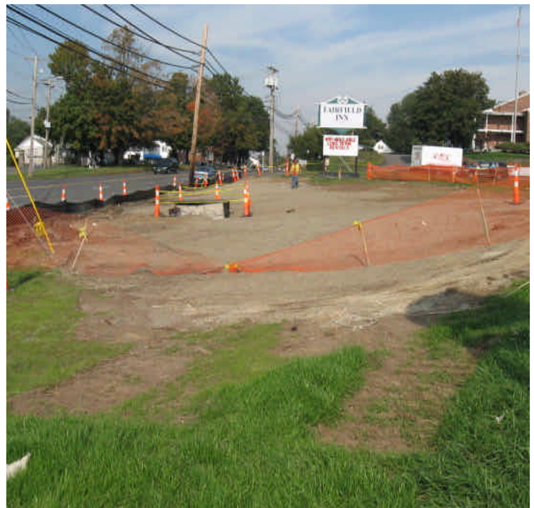
Photograph of site conditions off Rt. 1 in front of the Fairfield Inn. Erosion controls are in good shape here.
