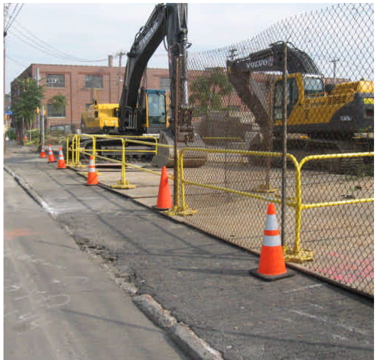
Area prepared for the installation of Vault # 7546 on Railroad Ave., north of Bostwick Ave.
