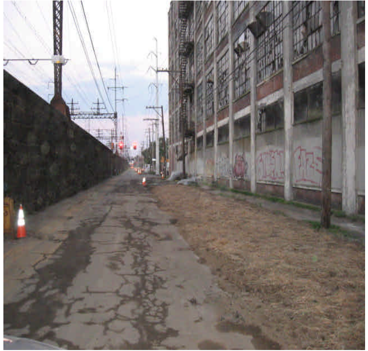
Photo taken facing east of the completed and restored trench area on Railroad Ave. between Hancock Ave and Howard Ave.
