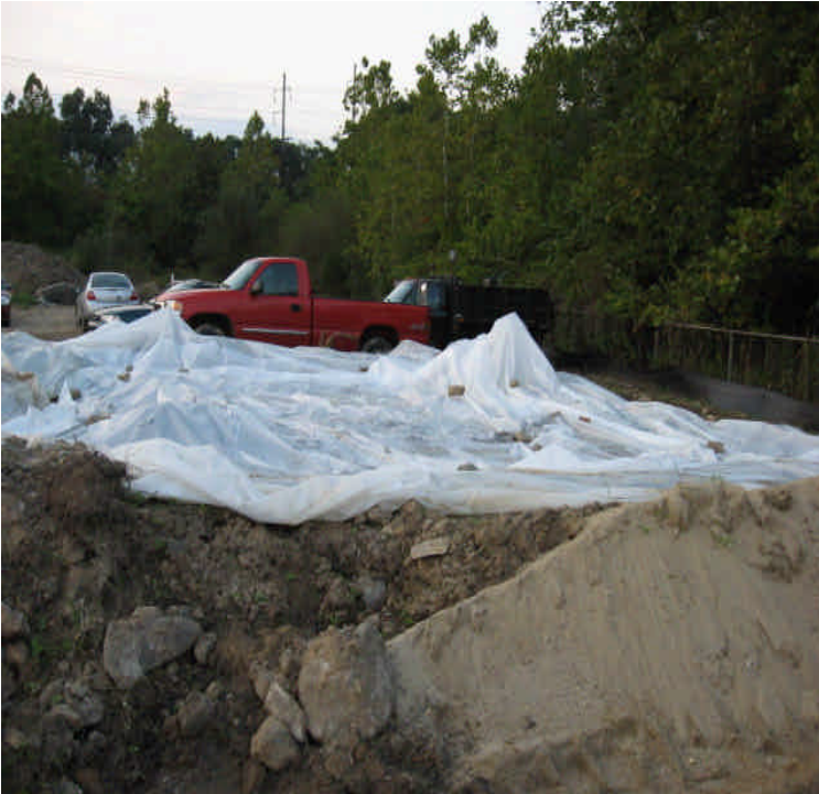
Abandoned concrete wash-out basin located in the Kings Highway laydown yard. The basin has been covered to discourage future use and prevent rainwater from mixing with the drying concrete
