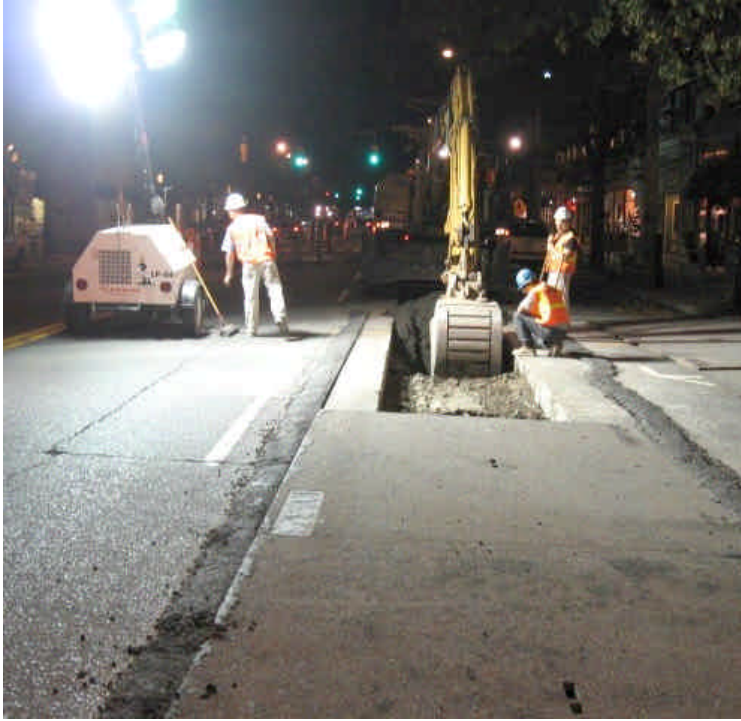
Photo taken of trenching activities on Rt. 1 between Round Hill Round Hill Rd. and Unquowa Rd.
