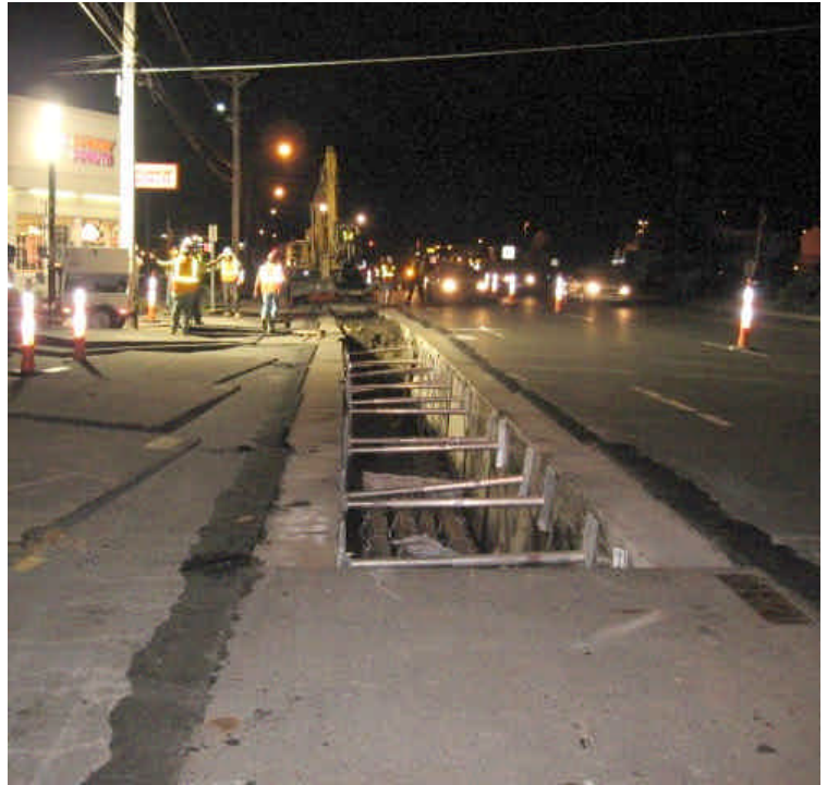
Photo taken facing west of trenching activities west of Old Post Rd.
