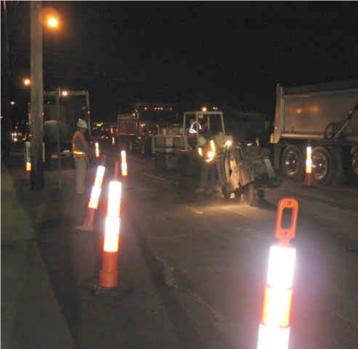
Photo of saw cutting activities along Rt. 1, west of Old Post Rd. Please note that the sweeper is immediately following saw cutting.
