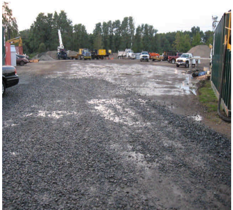
Photo of the Kings Highway laydown yard after soil surfaces were watered down before the mobilization of the night crews in an effort to prevent dust production.
