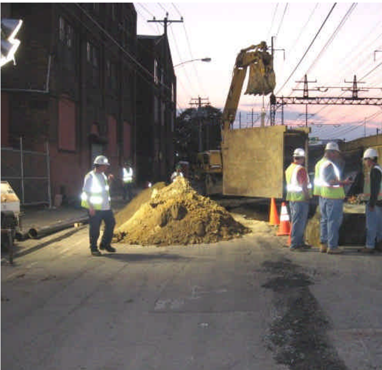
Photo taken facing west of utility work on Railroad Ave. Soil pile will be used to backfill the trench, any remaining soil should be properly disposed of.
