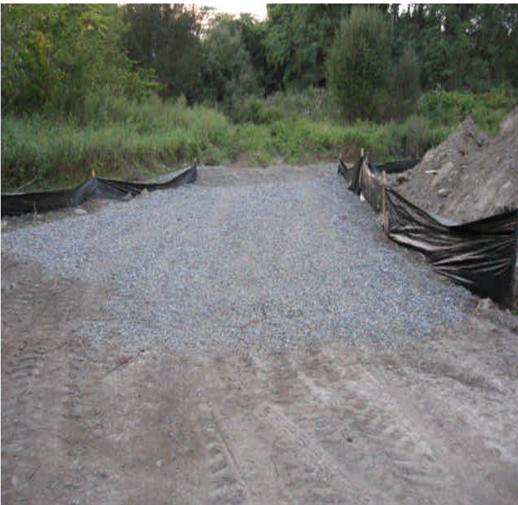
Photo showing stone berm that has been installed in the area that requires regular access by the Town of Fairfield in the Kings Highway laydown yard.
