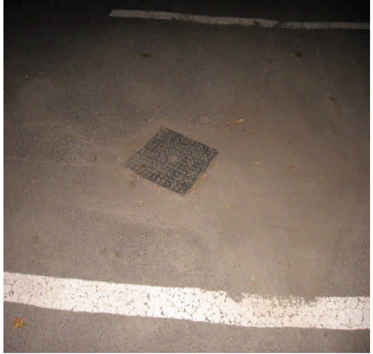
Catch basins located in the parking area adjacent to Vault #6428. Excess sediment has been removed from around the inlet.
