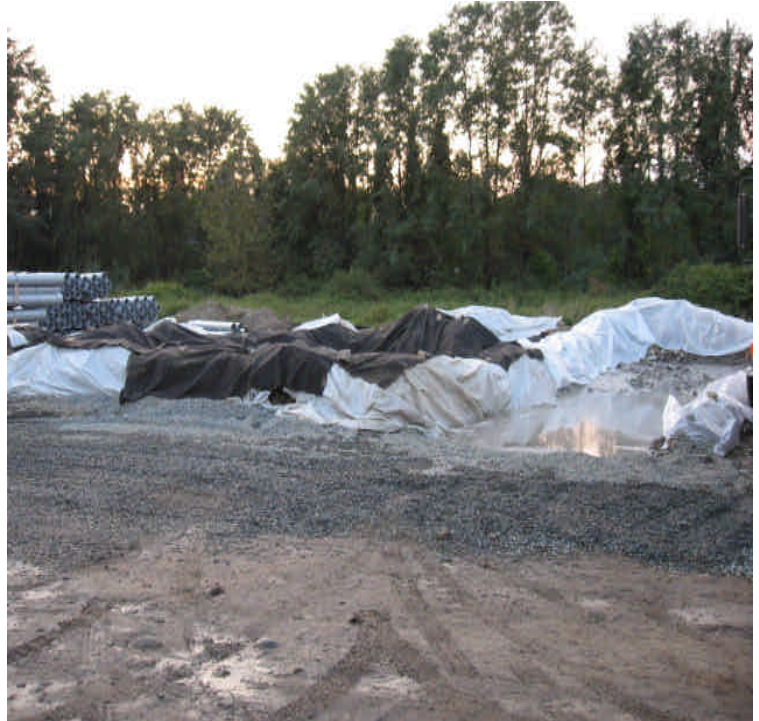
New concrete and sweeper wash-out basin located in the Kings Highway laydown yard. The basin is now properly lined.
