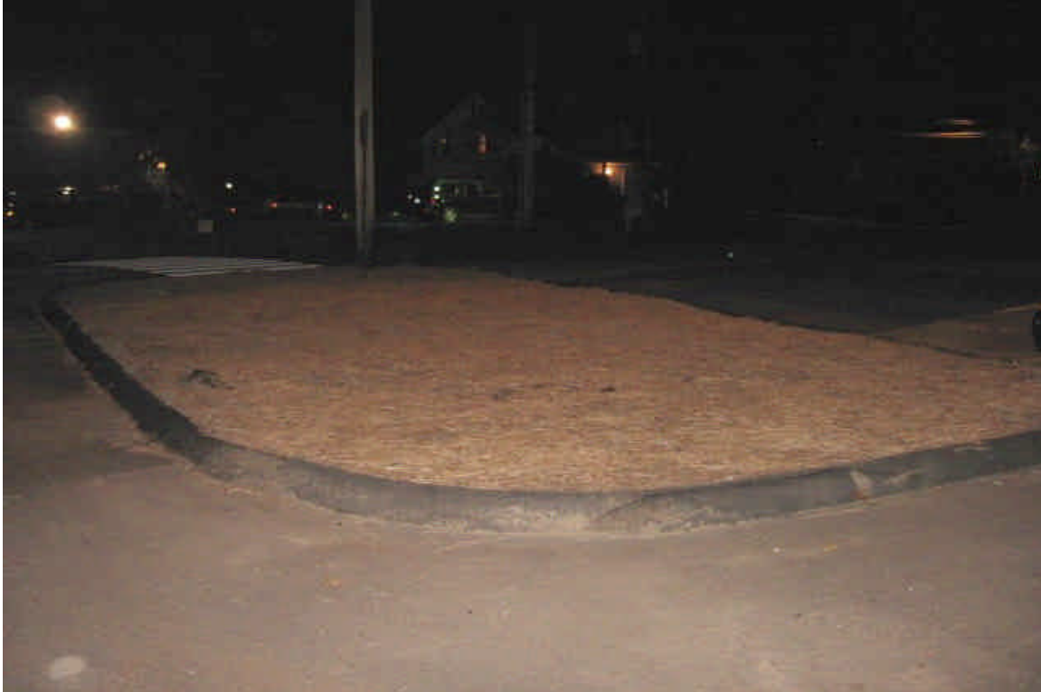
Island within parking area adjacent to Vault #6428 that has been restored and stabilized with hay mulch.
