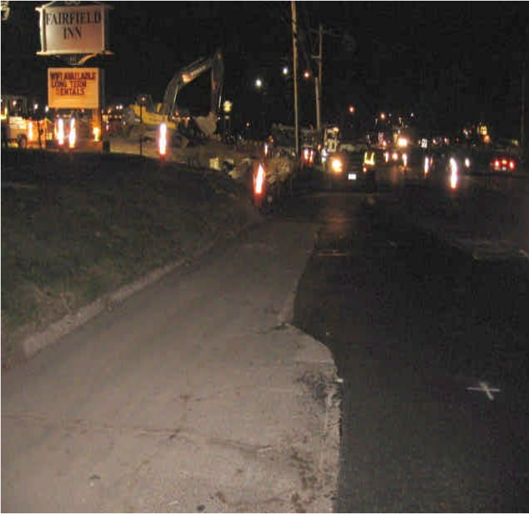
Photo of completed, as well as currently active, portions of trench work being conducted in front of the Fairfield Inn.
