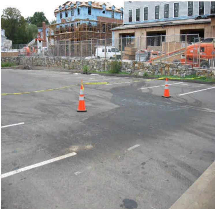
Photograph of parking area adjacent to the vault #6428 construction. Please note the spill/stain on the pavement that travels to the protected catch basin. Please see report for further details.
