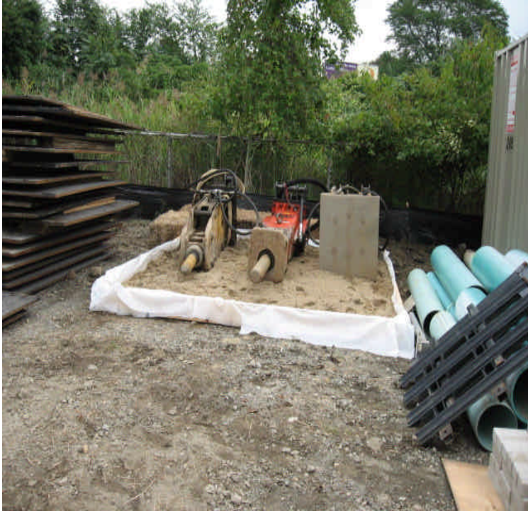
Containment area constructed within the Kings Highway storage area for the temporary storage of oil filled equipment.
