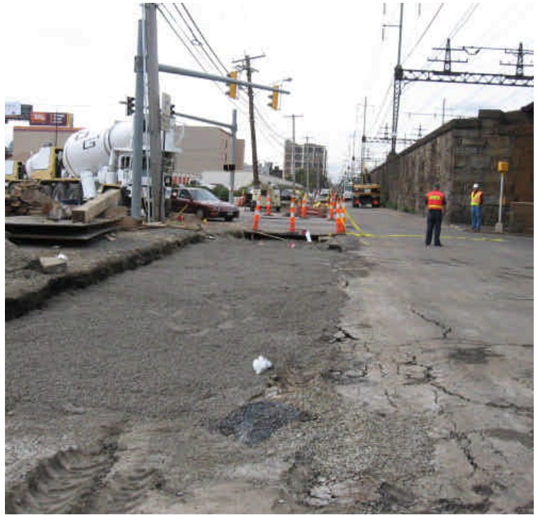
Photo taken on Railroad Ave. at its intersection with Wordin Ave. The trench in this area is being backfilled and trenching activities are progressing towards Howard Ave.
