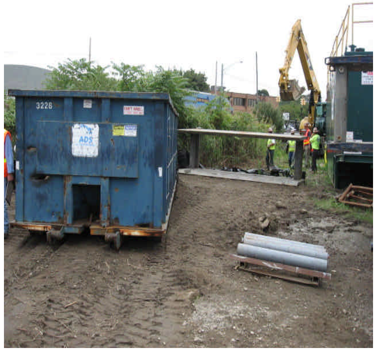
Photograph of former stockpile location and crews installing silt fence in the Kings Highway storage yard.
