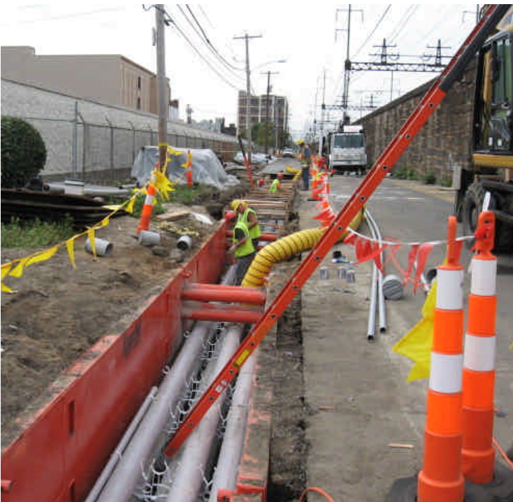
Photo of trench activities on Railroad Ave. between Wordin Ave. and Howard Ave.
