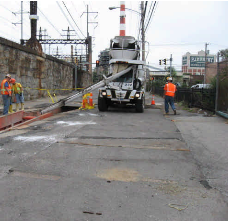
Trench being backfilled with concrete on Railroad Ave. between Lafayette Ave. and Warren Ave.
