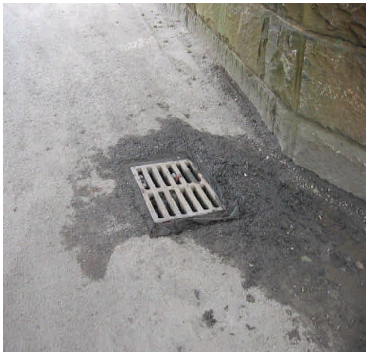
Catch basin located at the intersection of Wordin Ave. and Railroad Ave. When attempting to refresh filter fabric, it was found that the grate could not be removed without potentially causing damage.
