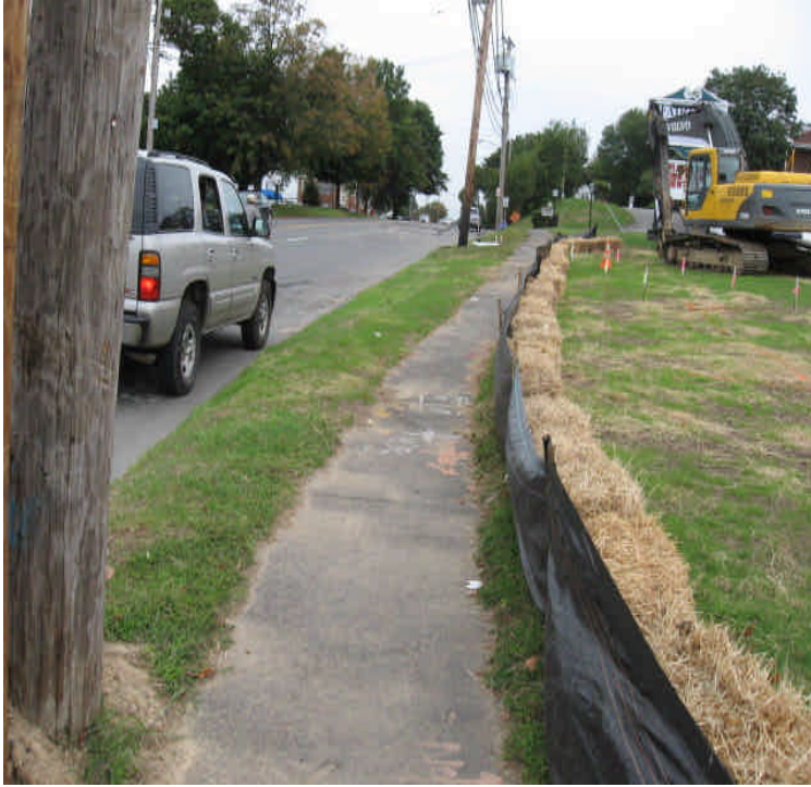
Vault #7537 construction area on the shoulder of Rt. 1. Grass is rapidly establishing in the restored area. No erosion was observed in this area.
