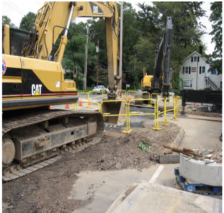
Photograph of vault #6428 construction area on Old Post Rd. The trench is being backfilled.
