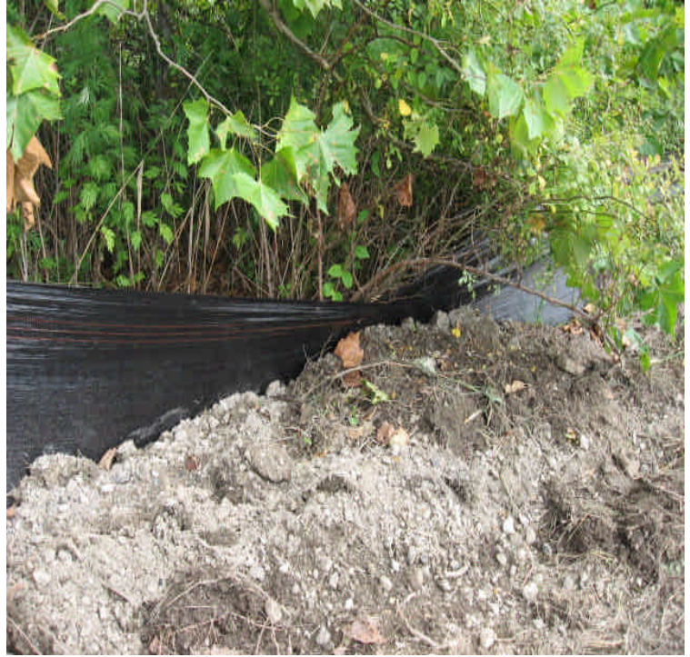
Portion of silt fence against the perimeter fence within the Kings Highway storage yard that has soils piled against them. The soils should be pulled back so that the controls are not compromised.
