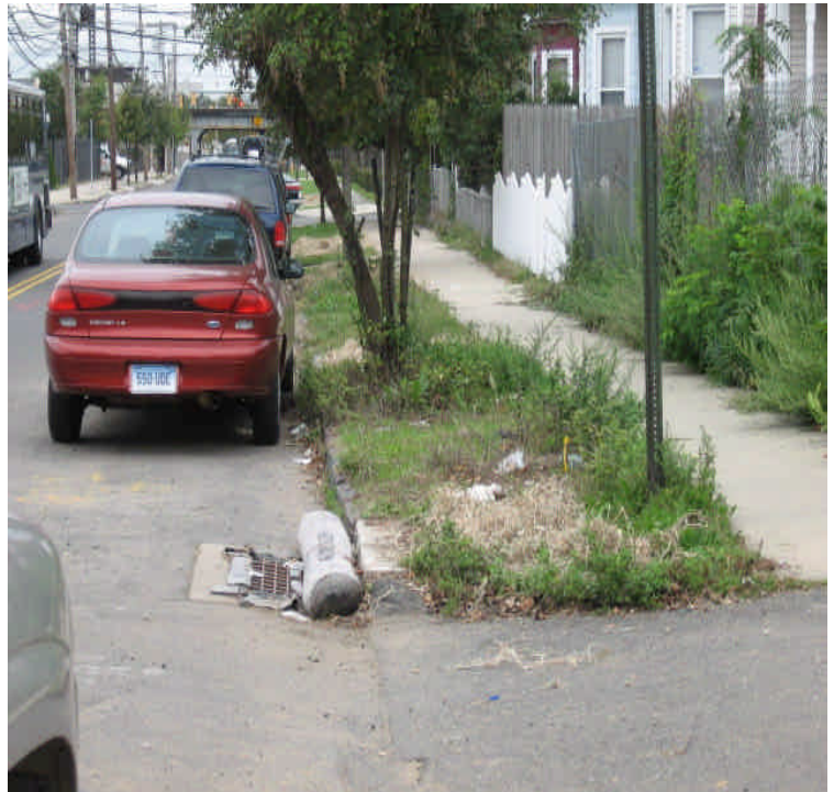
Photograph taken on Broad St. near Atlantic Ave. of catch basin protection and previously disturbed soils seeded and mulched with hay.
