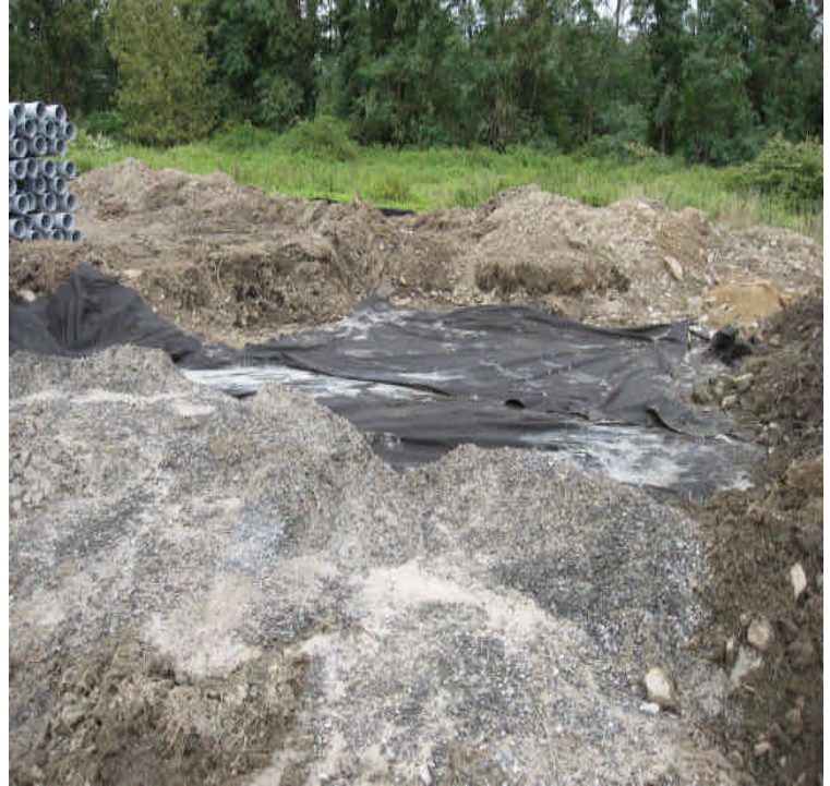
New concrete washout basin within the Kings Highway yard. Improvements to the geotextile fabric liner are still needed.
