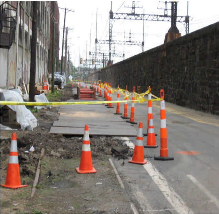
Trenching activities located on Railroad Ave. between Howard Ave. and Hancock Ave.
