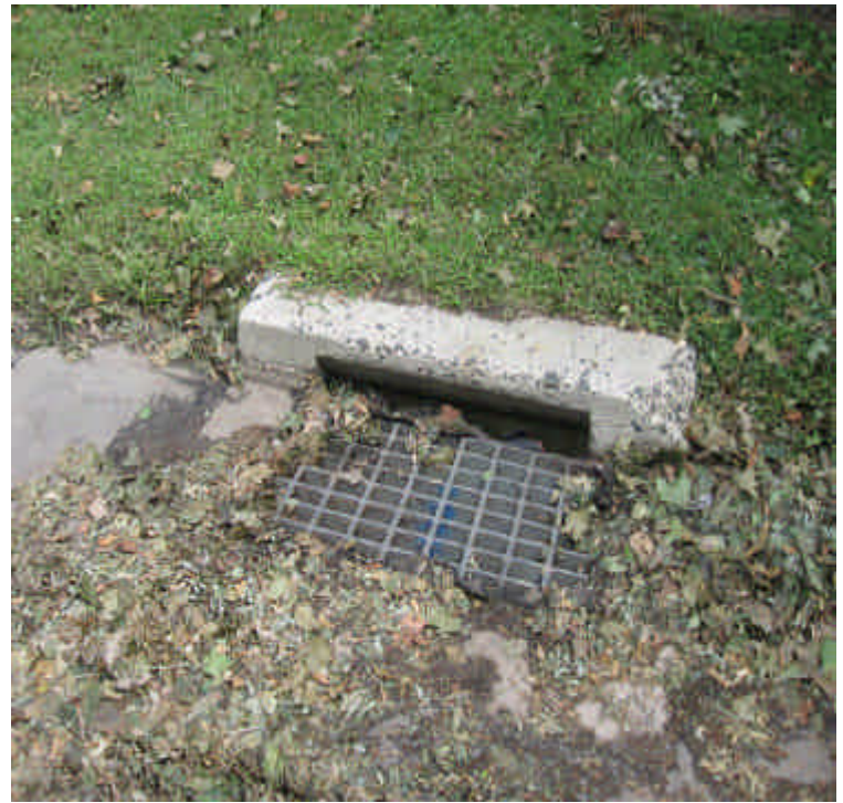
Catch basin located on Old Post Road. This basin accepts most stormwater associated with the vault #7537 construction. Controls should be installed if appropriate with CTDOT specifications.
