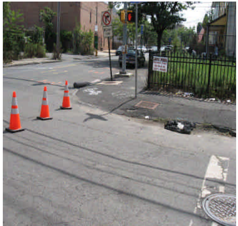
Appropriate catch basin protection at the corner of Lafayette Ave. and Railroad Ave.
