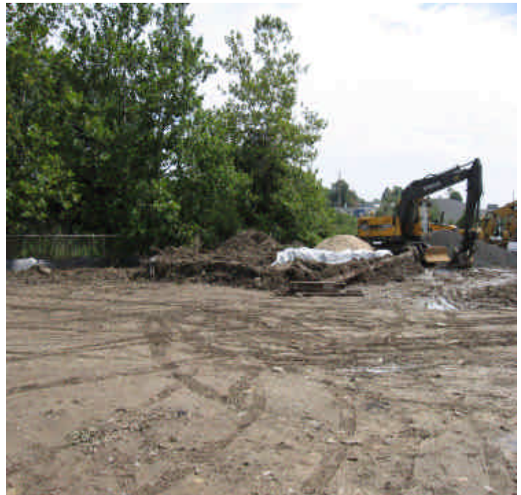
Photo of a lined pit, designated for concrete wash-out which has been installed since last week's inspection. However, it is located adjacent to the perimeter fence and would be best moved away from the sensitive areas.
