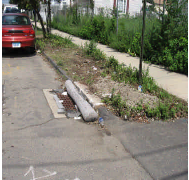
Example of appropriate catch basin protection associated with the utility work on and in the vicinity of Atlantic Ave and Broad Street.
