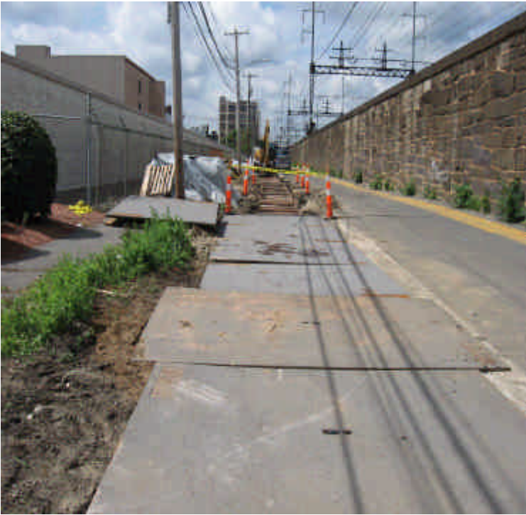
Photograph taken on Railroad Ave. looking towards Wordin Ave. of trench excavating activities.
