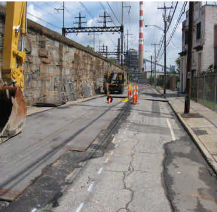
Photo of trench excavation activities on Railroad Ave. between Lafayette Ave. and Warren Ave. Photo taken facing Lafayette Ave.
