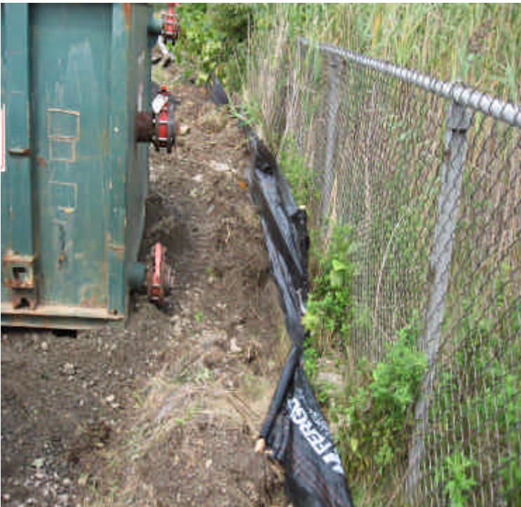
Silt fence has been installed between the Kings Highway storage yard and waterway. Portions of the silt fence have not been installed properly, either slumping or not toed-in.
