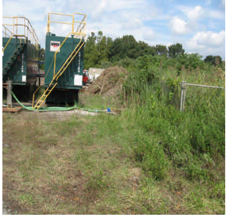
Silt fence/erosion controls still need to be properly installed in this area between the yard (and stockpile) and the waterway
