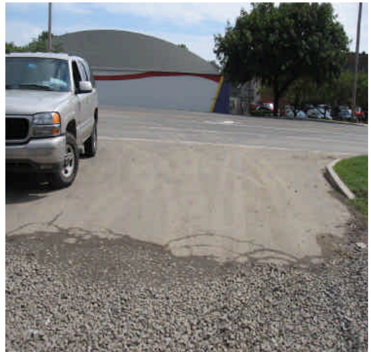
Construction entrance of the Kings Highway storage yard. Very minor amounts of sediment were tracked on the roadway in comparison to last week's inspection. The controls were improved
