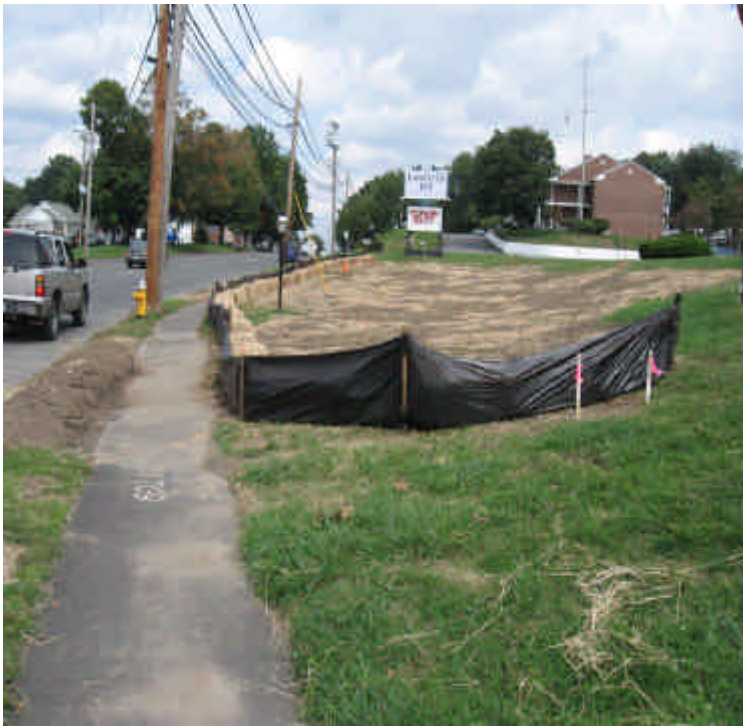
Vault #7537 construction area on the shoulder of Rt. 1. Work is complete in this area and disturbed soils have been seeded and mulched. Continue to monitor and repair/reinforce controls if runoff to the roadway is noted.
