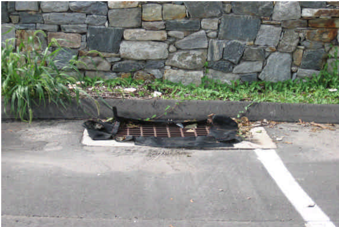
Photo of properly protected catch basin located in parking lot adjacent to vault 27 construction activities.
