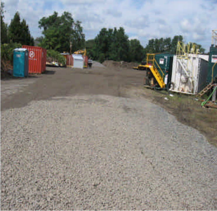
Kings Highway storage yard and construction entrance. The material used to reduce mud in the yard has visibly reduced vehicle tracking
