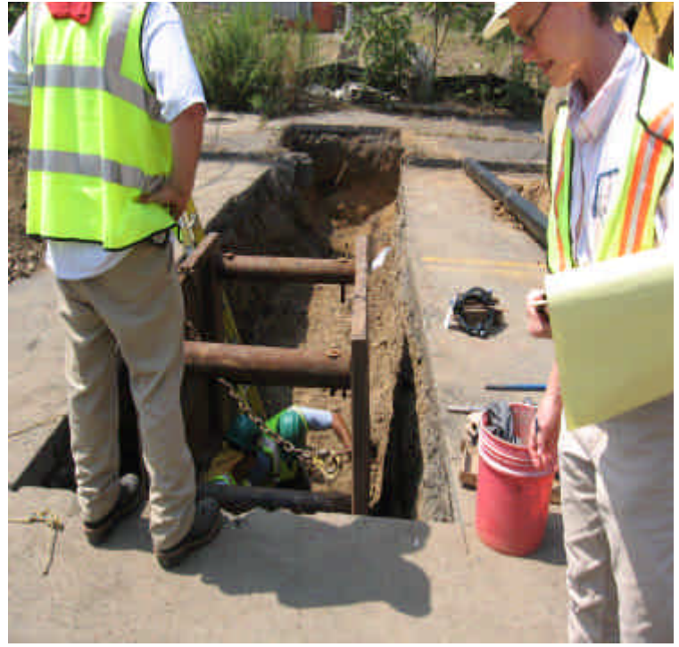
Utility relocation construction activities near the intersection of Broad St. and Cottage St.
