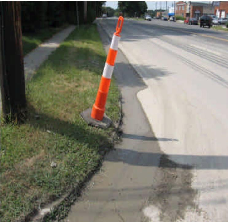
Photo taken at the intersection of Rt. 130 (Post Road) and Shoreham Village Dr. looking southwest at Rt. 130. Saw-cutting in the roadway during nightwork created a slurry of fine sediments that has accumulated along the edge of Rt. 130. (Fairfield)
