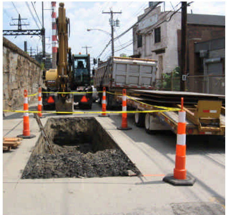
Trench excavation activities on Railroad Ave. between Lafayette St. and Warren St.
