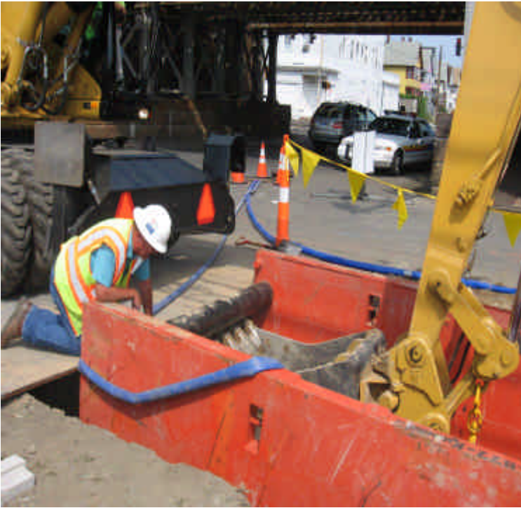
Photo of trenching activities on the shoulder of Railroad Ave. near the intersection with Warden Ave. During excavation, crews encountered an unmapped, brick, sewer conveyance system. Hoses are diverting contents out of work area to the City's sewer system.
