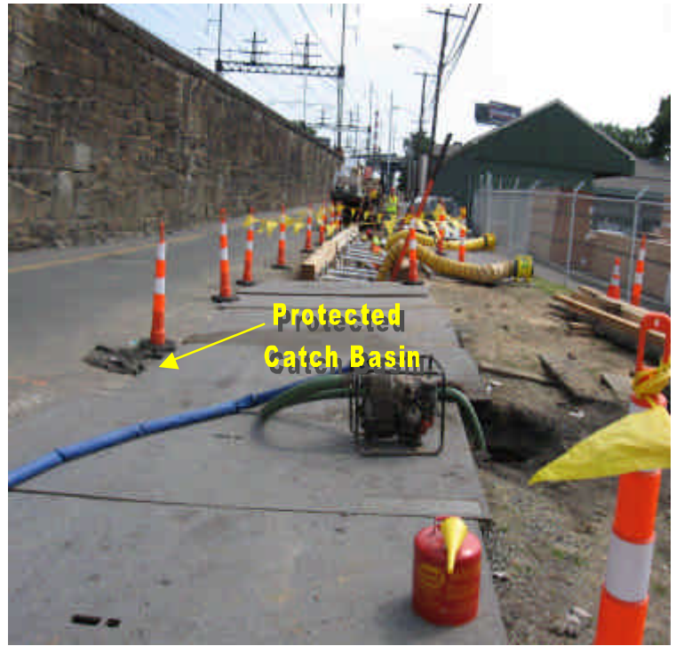
Photo of work along Railroad Ave. between Warden Ave. and Iranistan Ave. Catch basins in the area are protected.
