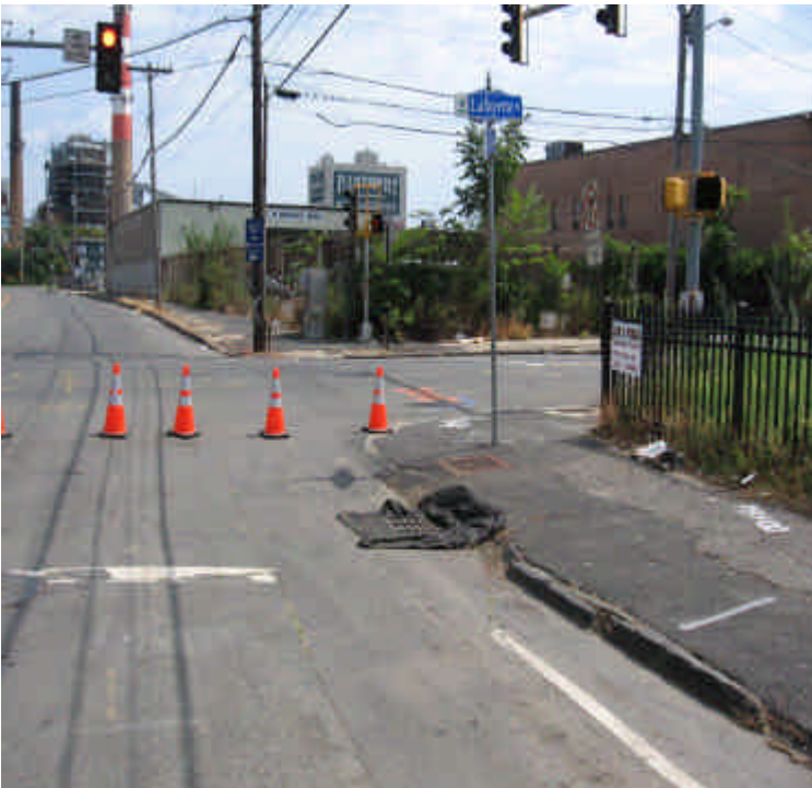
Photo taken from Railroad Ave. facing east looking at the intersection with Lafayette St. Catch basins are being protected.
