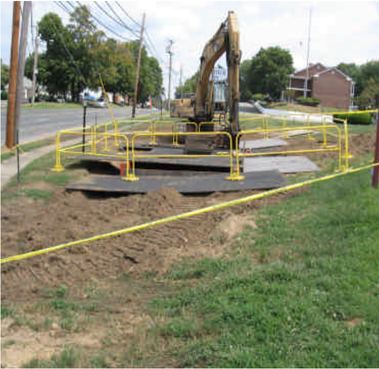
Photo of the construction activities associated with the installation of Vault 7537 adjacent to Rt. 130. (Fairfield)
