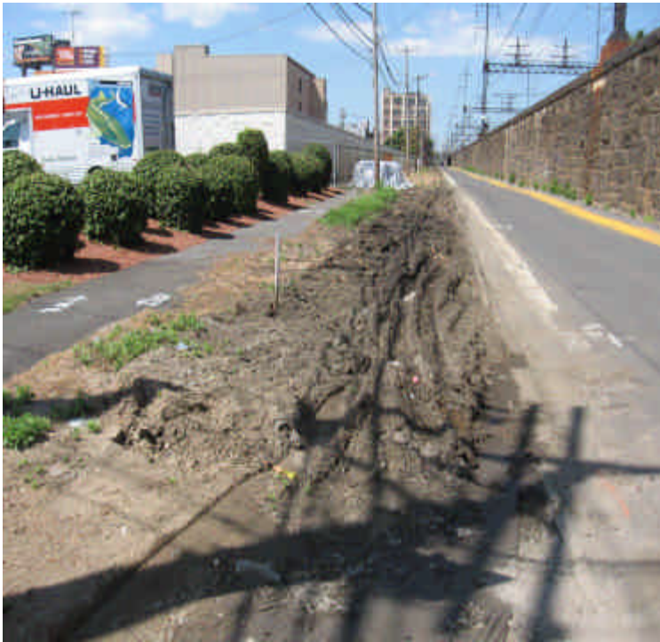
Work area along Railroad Ave, between Warden Ave and Howard Ave. Railroad ties were pulled up and currently stored to be removed from site (in background of photo). Regrade and restore roadside area when feasible.
