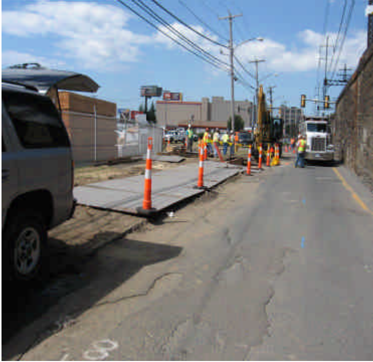
Photo of trenching activities on the shoulder of Railroad Ave. near the intersection of Railroad Ave. and Warden Ave.
