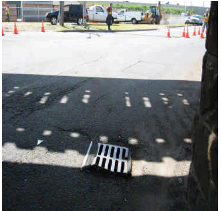
Protected catch basin located under commuter rail on Warden Ave near intersection with Railroad Ave.
