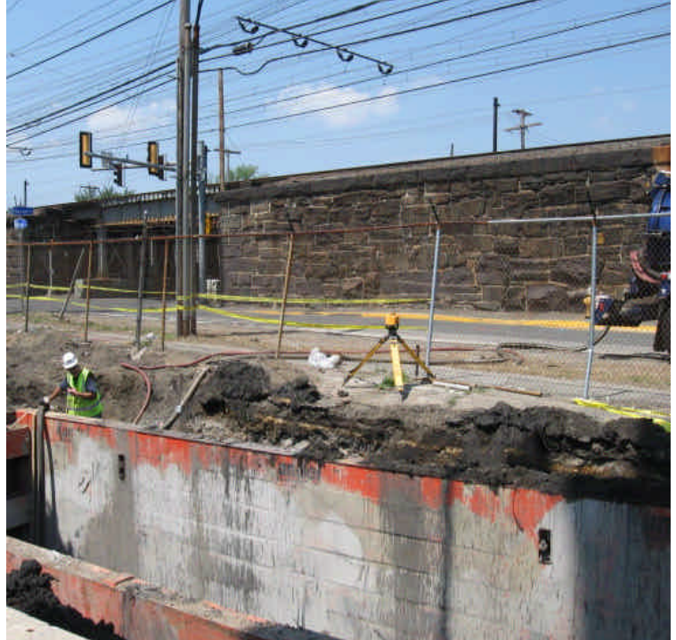
Vault opening within parking lot with a vacuum truck parked on Railroad Avenue removing water from the excavation.
