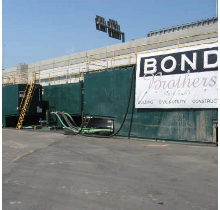
Frac tanks located at the contractor's storage area. These serve as holding, settling and filtration tanks for dewatering
