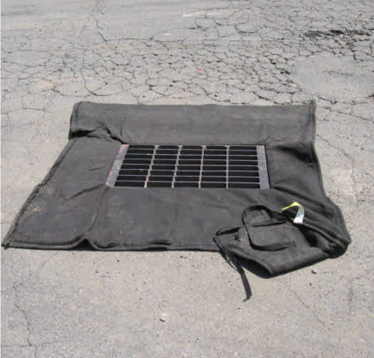
Catch basin with filter fabric located adjacent to construction area within the parking lot.
