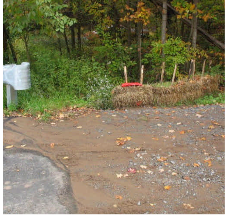
Extra haybales are needed to prevent runoff at Mansion Rd. entrance.
