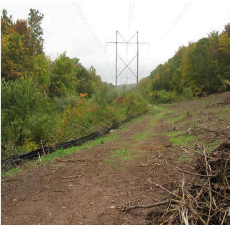
Silt fence looking north off High Hill Rd.
